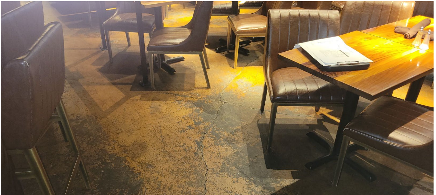
Photograph 6. Minor cracking in the northwestern portion of the 13 Coins Restaurant on the King Street property. Cracking size and amount appear to be the same as the 2021/2022 inspections.
