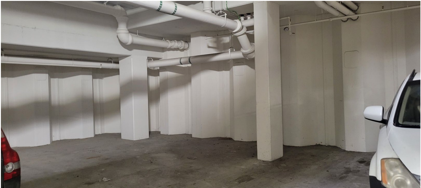
Photograph 2. Steel sheet pile walls in the parking garage. No damage or areas of concern were observed.
