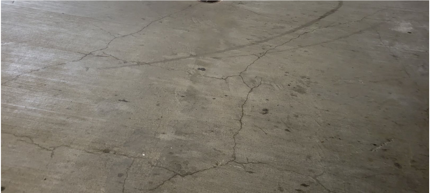
Photograph 3. Nonstructural hairline cracking in the underground parking garage. Cracking does not appear to have worsened since the 2021/2022 inspections. This area is to be monitored in the next annual inspection; repairs are not needed at this time.
