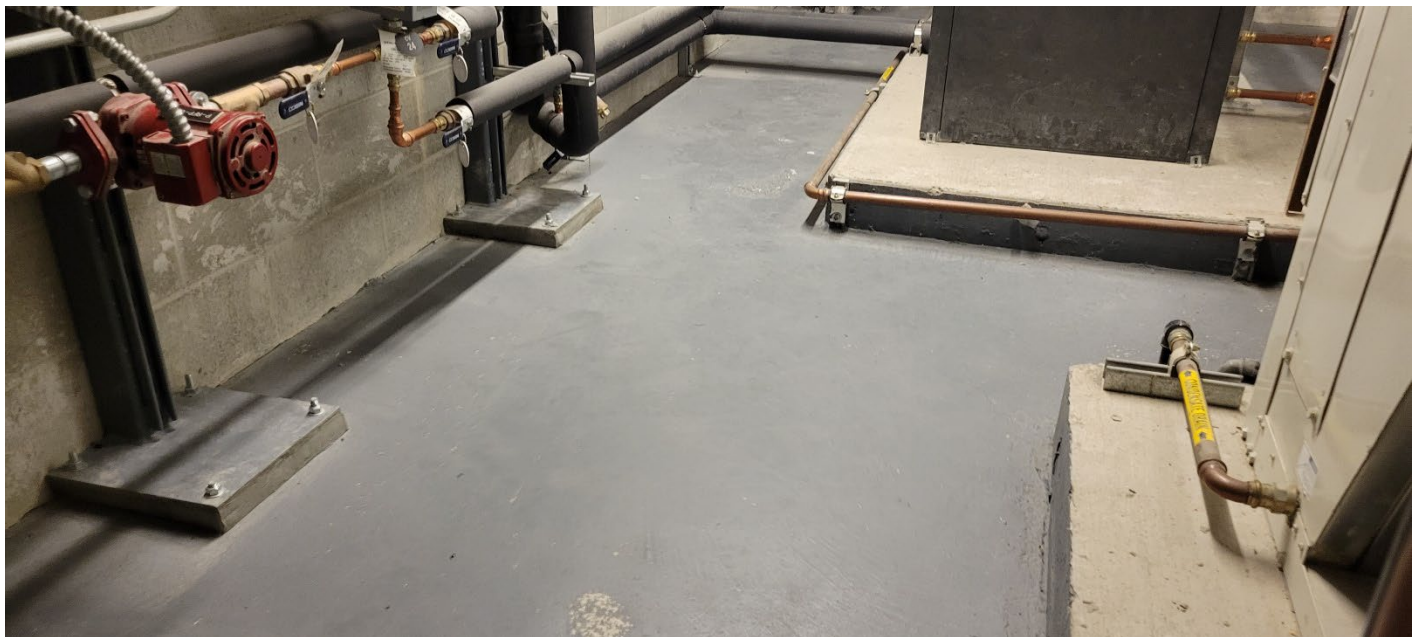
Photograph 4. Machine rooms free of visible structural cracking. Hairline cracking in maintenance areas are painted over with epoxy paint.
