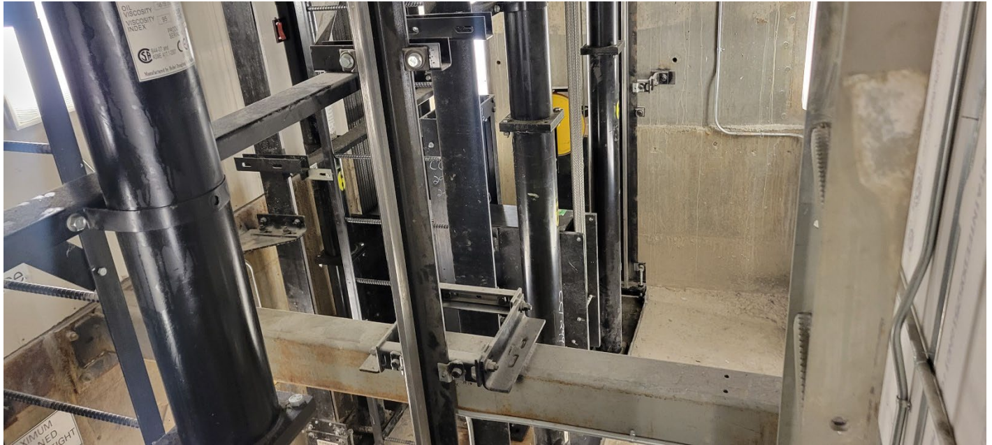
Photograph 5. Elevator pits free of visible structural cracking.
