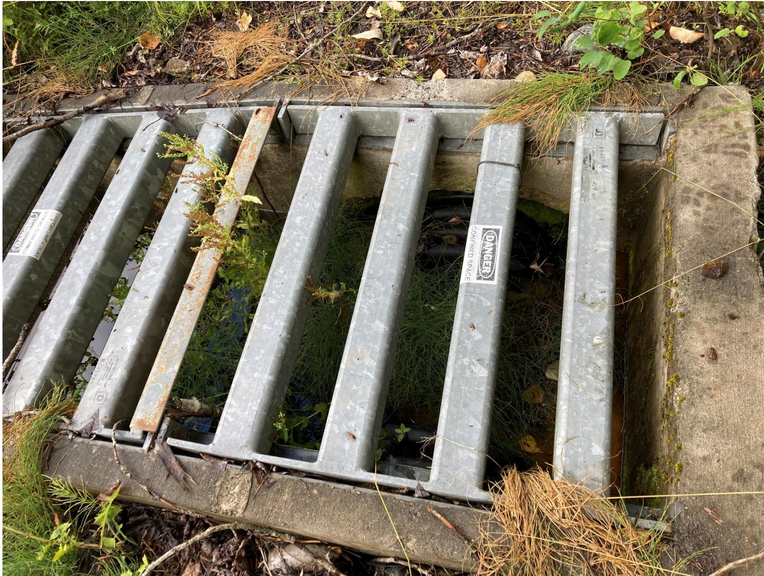
Photo 4: French drain catch basin with standing water and vegetation
