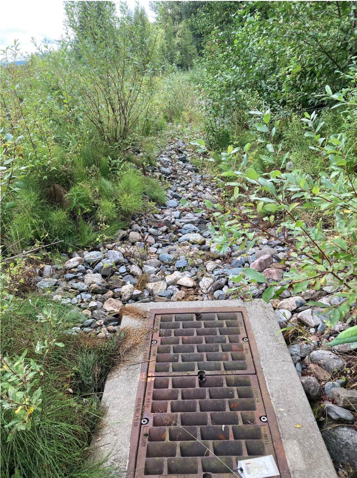
Photo 3: French drain and catch basin on TDF-1
