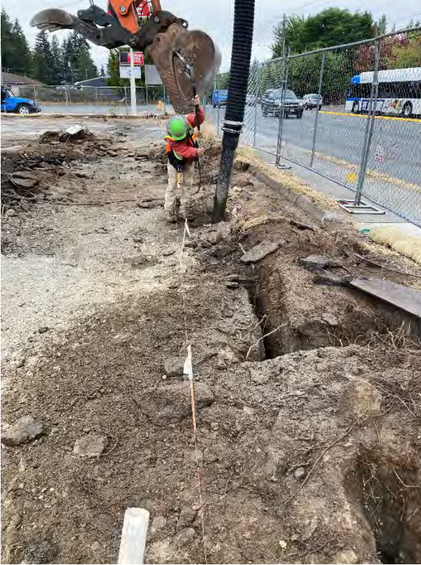
Photo 3: Ongoing potholing and locating of communication/fiber lines on the north end of the site.
