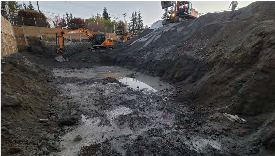
Photo 1. Groundwater seepage at the base of the excavation before digging began for the day.
