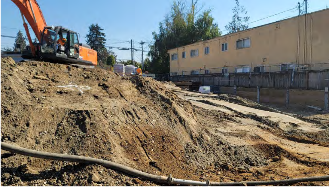
Photo 1: Soil ramp for soil nail drill access in the southwest corner of the site. Photo looking south.
