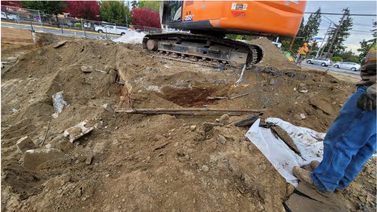
Photo 1: View of pipe discovered near north side of site, adjacent to a known UST. Photo looking north.
