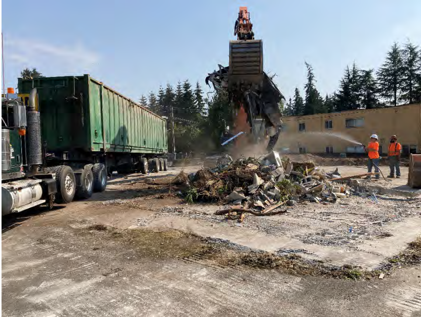
Photo 1: Final building debris pile being loaded into dumpster for disposal, dust control being deployed via garden hose.
