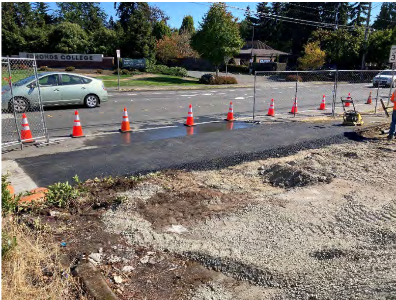
Photo 2: Quarry spalls installed for the stabilized construction entrance on 68 th Avenue, viewing southeast.
