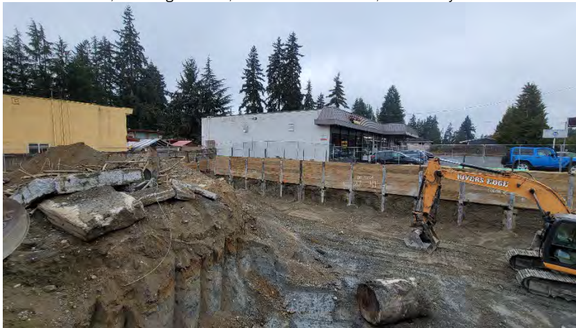
Figure 1. Facing the west, note the obvious color change (blue-gray to more gray-brown) that appears to follow the clean / contaminated boundary. The blue-gray dirt shows obvious signs of contamination (high PID readings, heavy petroleum-like odors, and moderate to heavy sheens).
