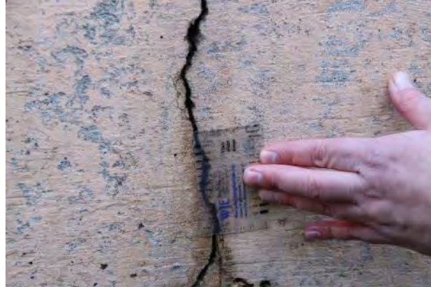
Figure 3b. Lower portion of crack on January 10, 2023.
