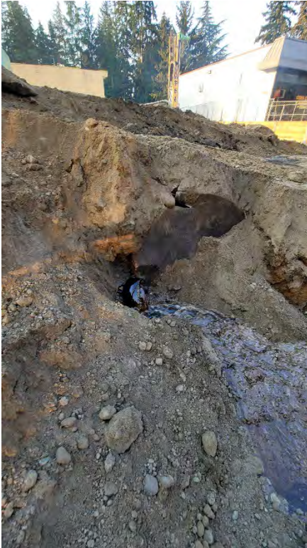
Figure 2. Photo of damage to UST.
