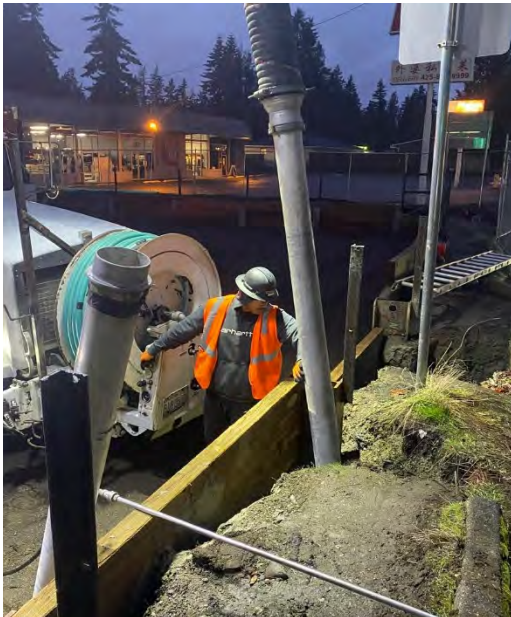
Figure 1. The beginning of removal of the N07-N7.5 cell using the vac truck and high-pressure water wands
