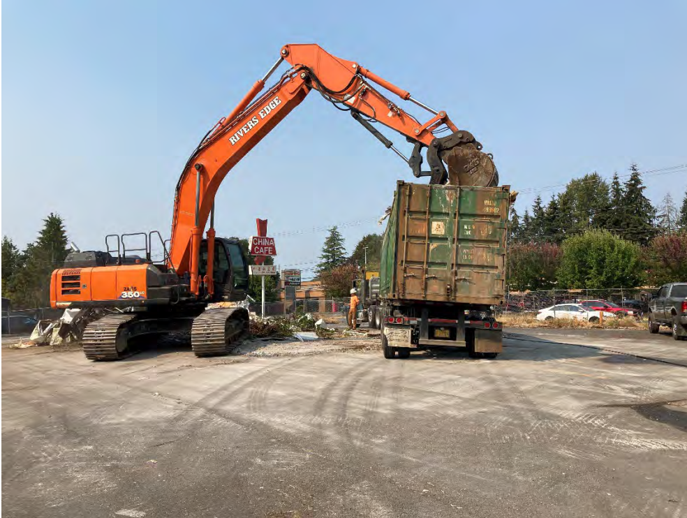
Photo 1: Completion of building demolition, REES is controlling for dust with a garden hose in the photo.
