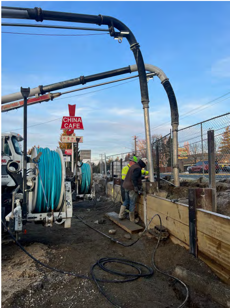
Photo 1. The beginning of removal of the N08.5-N09 cell using the vac truck and high-pressure water wands.
