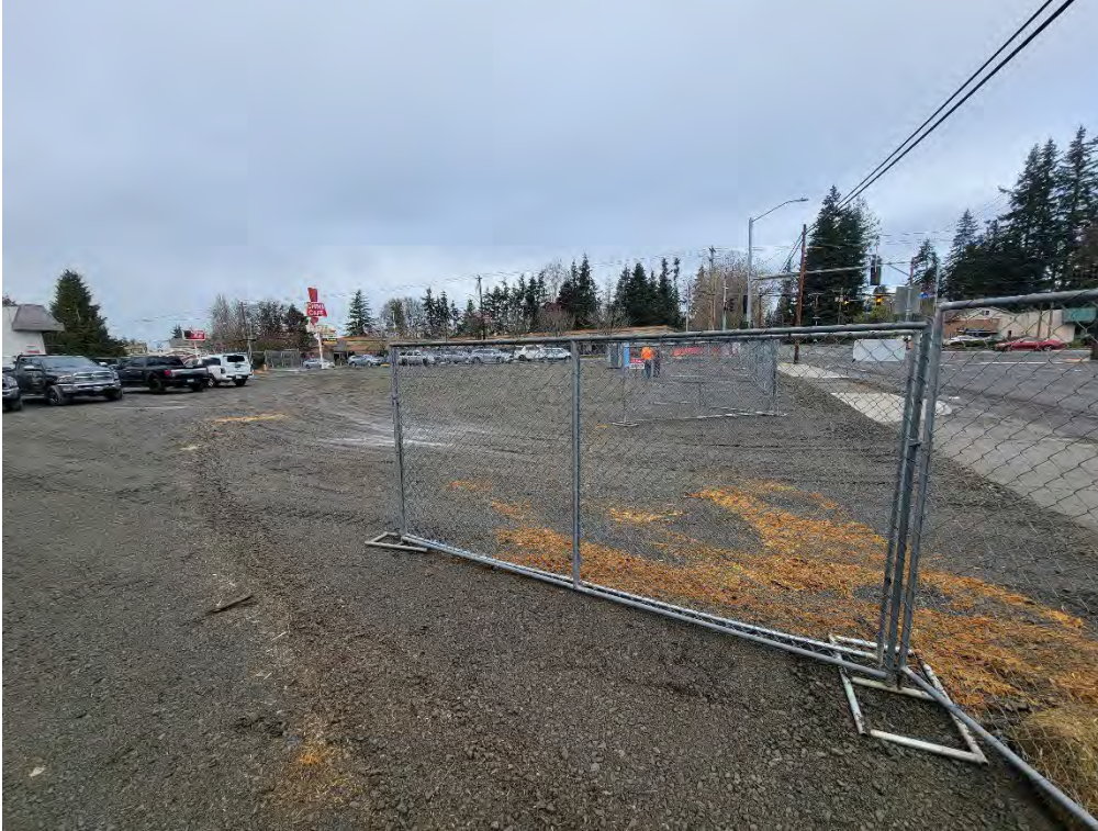
Photo 3. Final restored Site conditions as of 1/6/2023, looking north along the east side of the Site.
