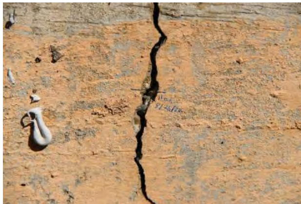
Figure 2a. Upper portion of crack on August 25, 2022.
