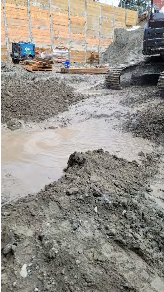
Figure 2. Groundwater seepage following light rains earlier in the day.
