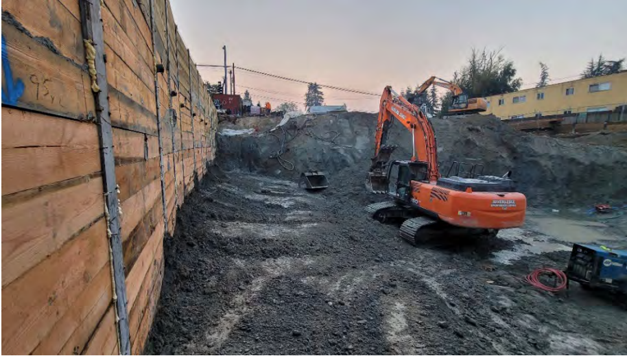
Photo 1. The site near the beginning of the day, facing southeast, showing the extent of groundwater seepage overnight.
