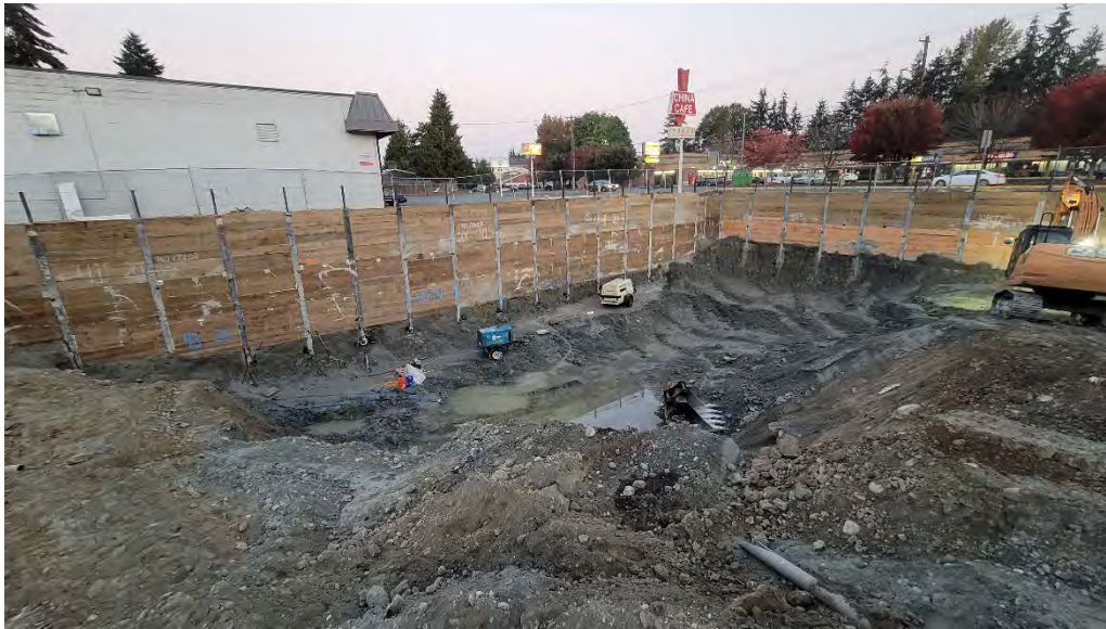
Figure 1. The northwest corner of the excavation as seen at the beginning of the day today (10/17)
