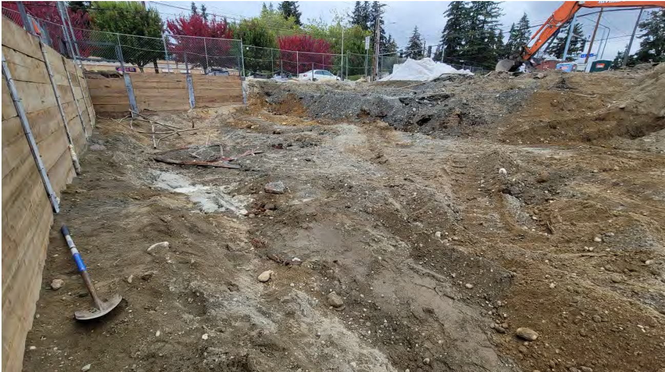
Photo 4: Excavation of clean soil progressing west to approximate elevation 444. Photo looking north.
