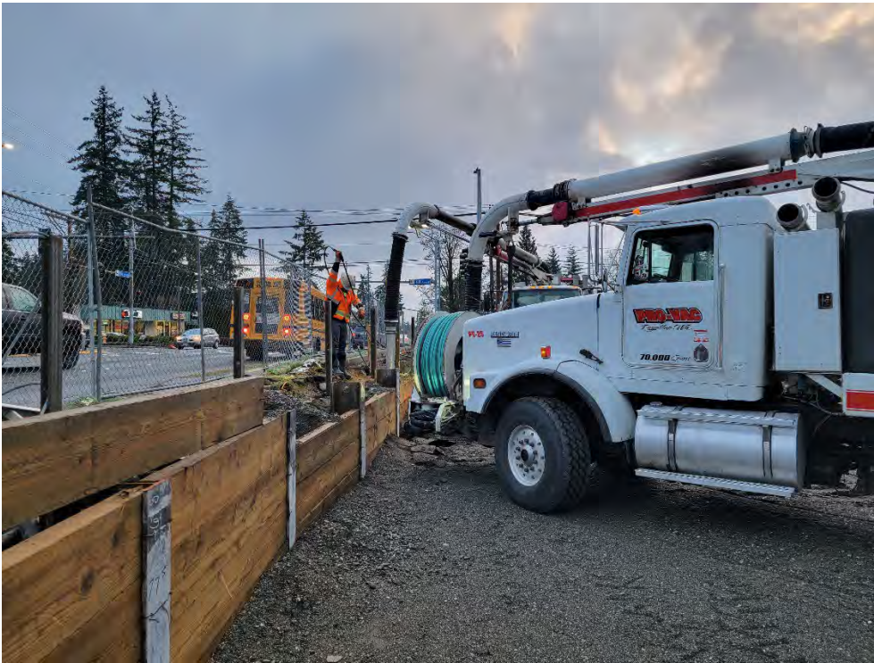
Photo 1. The beginning of removal of the N08-N08.5 cell using the vac truck and high-pressure water wands.
