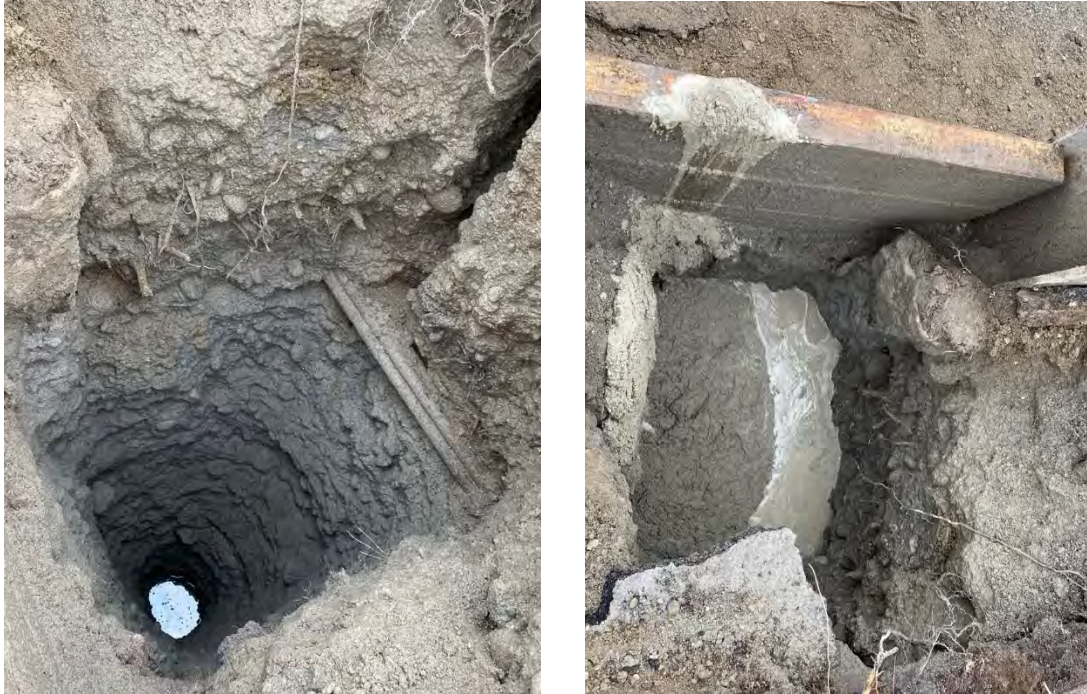
Figure 2. The bottom of the excavation at the N07-N7.5 cell filled with water from the high-pressure water wands used to cut through dense fill materials (left). The N07-N7.5 cell after being filled with controlled density fill (cdf) material (right).
