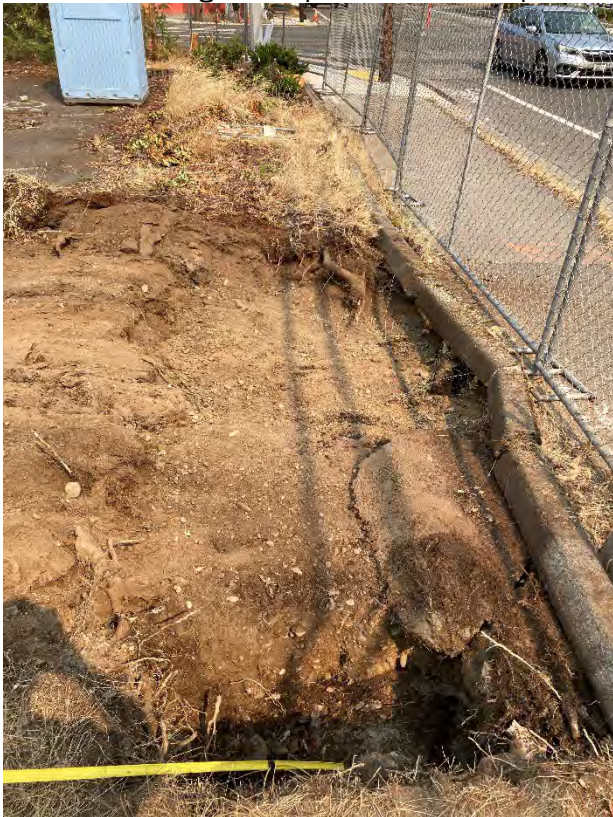
Photo 4: Minor excavation for water meter location on the west side of the site.
