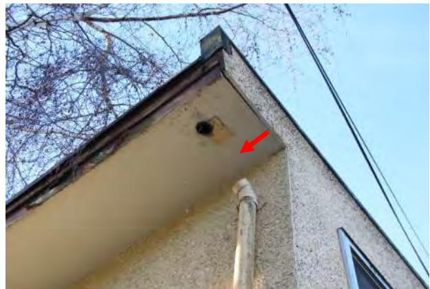
Figure 4b. Downspout at northeast corner of Subject Structure on January 10, 2023 (red arrow indicates location of fallen section).
