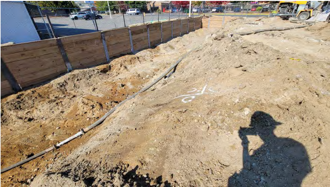
Photo 2: Lagging progressing north along the west wall and east along the north wall to N03. Photo looking northwest.
