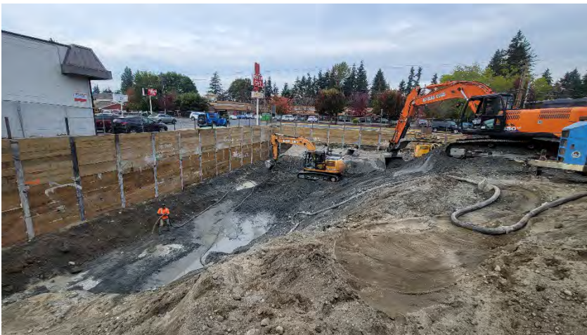
Photo 2. Excavation along the west wall, standing in a similar location to Photo 1—facing north, near the end of the day.
