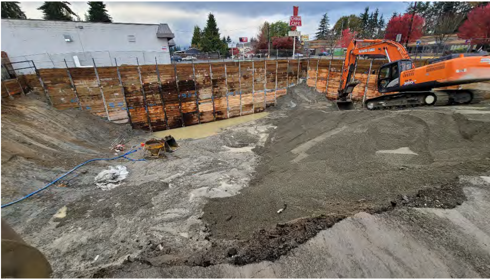
Photo 1. Amount of groundwater accumulation and back fill gravel near the beginning of the day.
