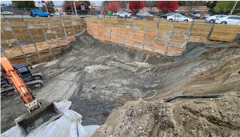
Figure 2. The northern extent of the excavation near the end of the day.
