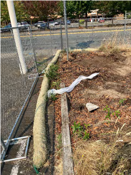
Photo 2: Installed straw wattle in the northwest corner of the site for erosion control.
