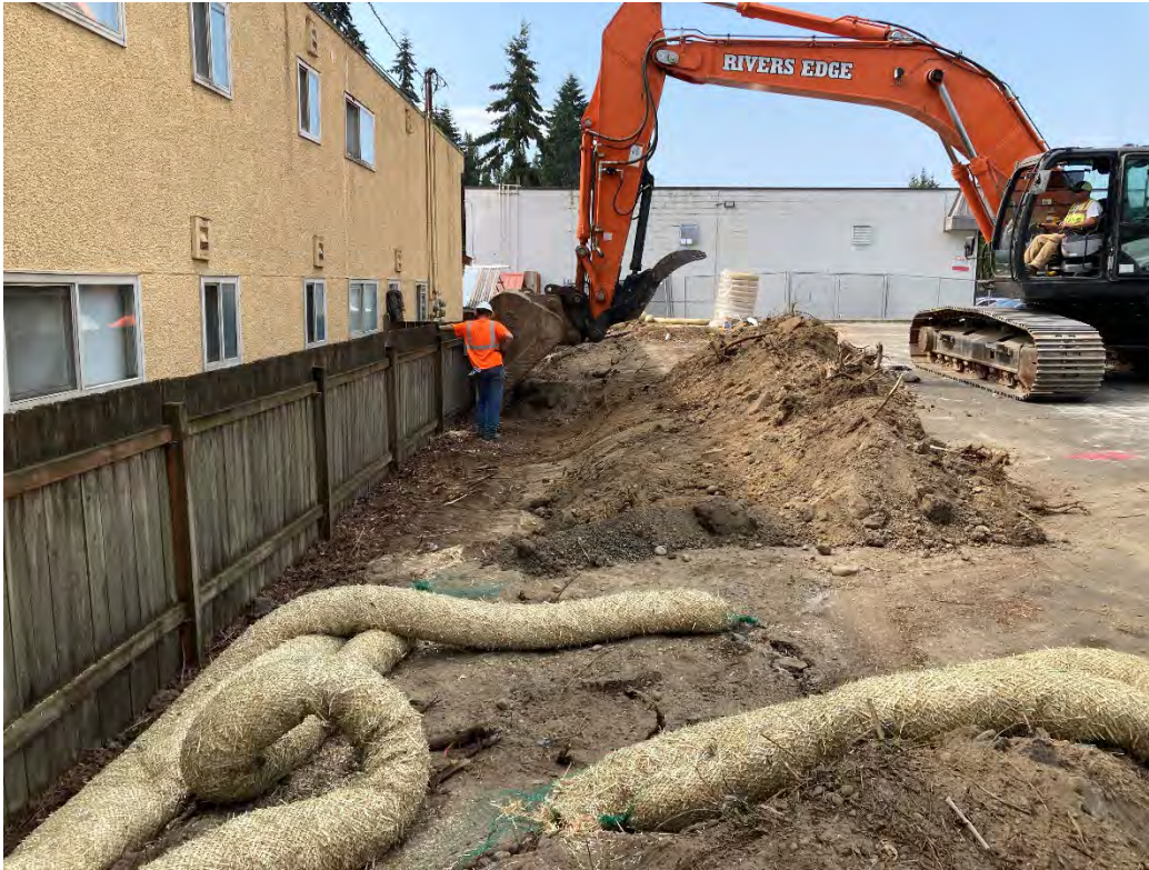
Photo 3: Soil being scraped from the incline at the south end of the site. Straw wattle at the ready for deployment as erosion control.
