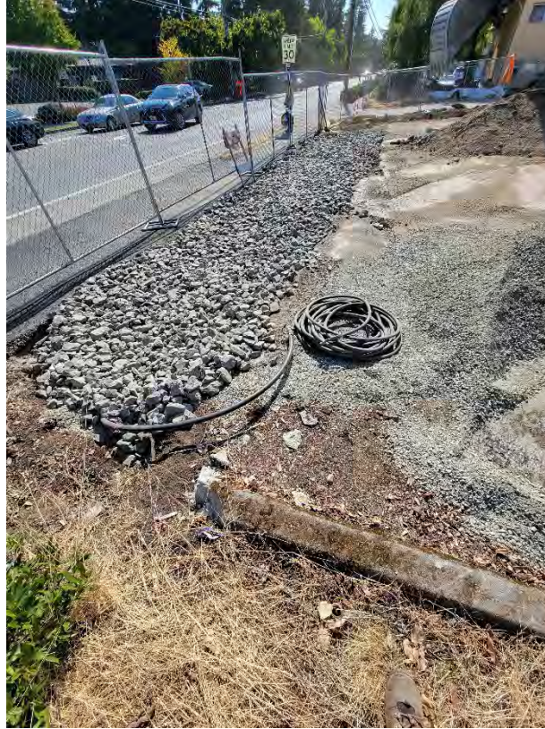
Photo 3: Quarry spalls installed for the stabilized construction entrance on 68 th Avenue, looking southeast.
