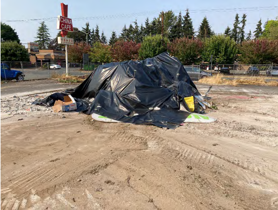
Photo 3: Building debris pile covered with plastic at the end of the day.
