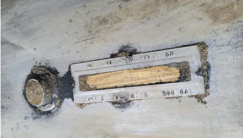
Photo 2. Label found on the side of UST 2.
