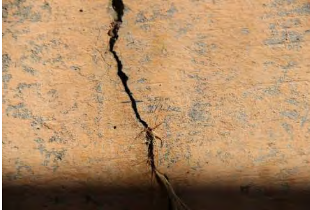
Figure 3a. Lower portion of crack on August 25, 2022.
