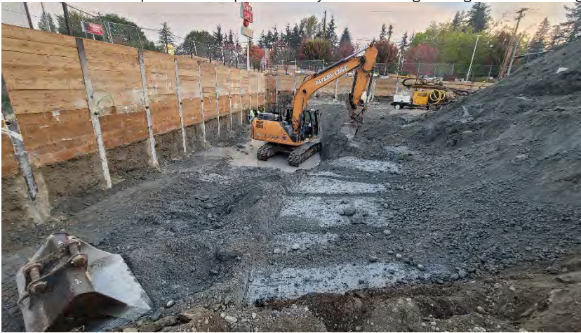
Photo 1. Excavation along the western edge of the site, facing north, at the beginning of the day.
