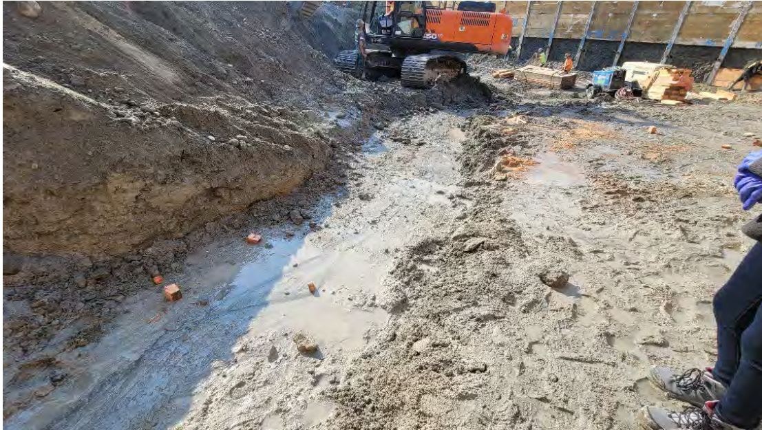
Figure 1. Mitigating groundwater seepage from the northeast corner of the site.
