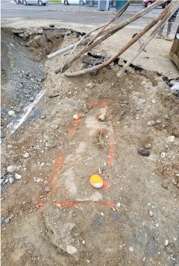
Figure 2. UST 3 is outlined in orange spray-paint. The rocks that are painted orange are covering the tank ports.
