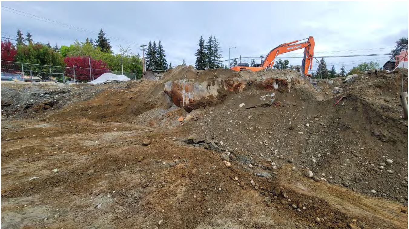
Photo 2: Photo of excavation advancing up to former building foundation. Photo looking northeast.
