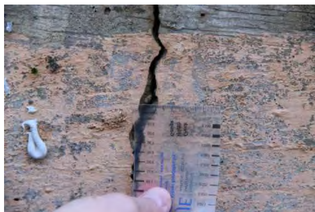
Figure 2b. Upper portion of crack on January 10, 2023.
