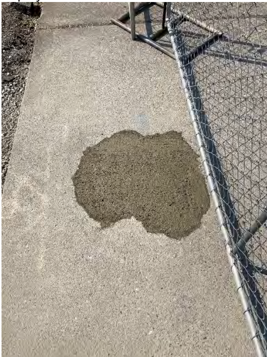
Photo 4: Water main patch.
