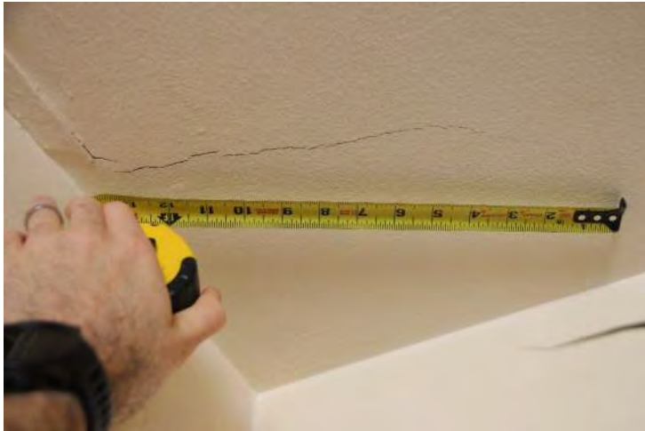
Figure 3. Closer view of crack in ceiling finish in Unit 131 on January 10, 2023
