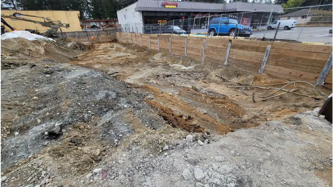
Photo 3: Excavation of clean soil progressing west to approximate elevation 444. Photo looking southwest.
