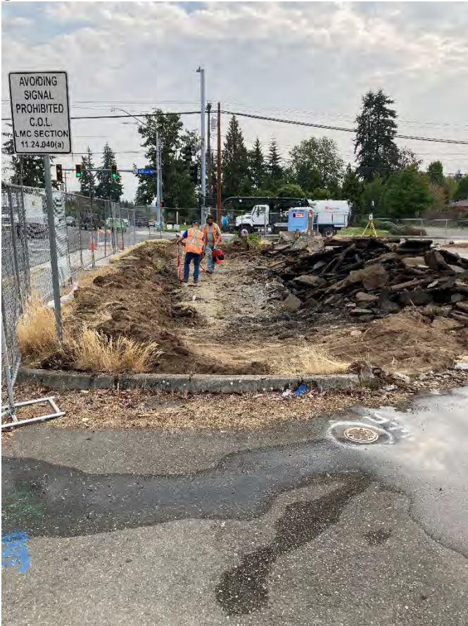
Photo 2: Asphalt being peeled back by REES at the north end of the site.
