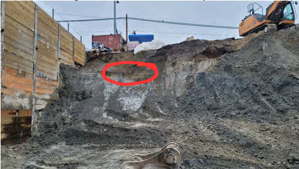
Figure 1. Contaminated sand layer in the eastern sidewall.
