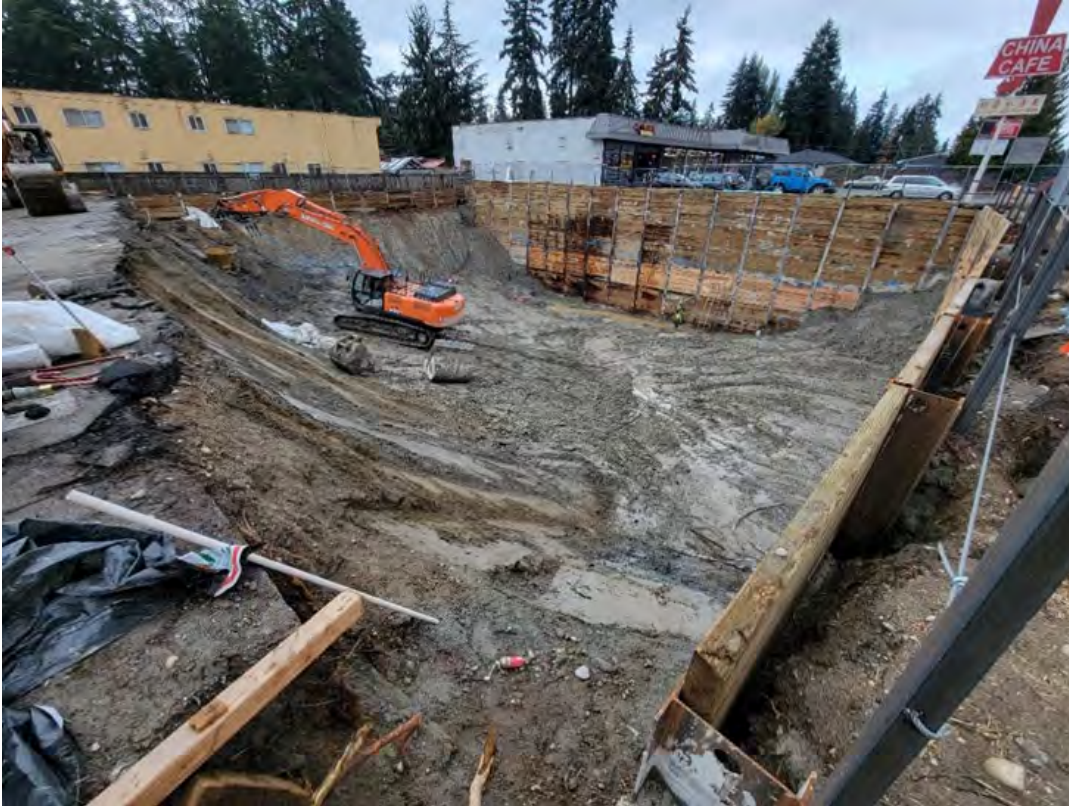
Photograph 1. Final IA excavation extents as photographed prior to initiating backfill, looking southwest.
