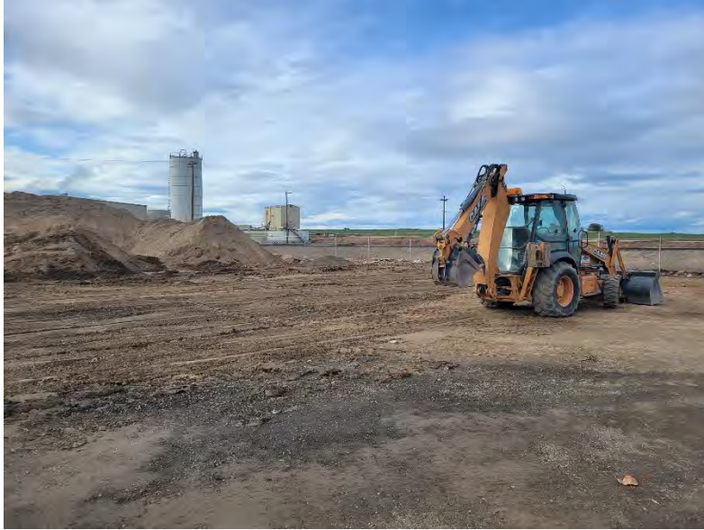
Photo 25. View of backfilled west pit at end of SVE operation. Photo taken on November 7, 2022, facing north.
