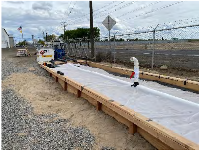
Photo 17. View of SVE treatment system. SVE treatment system was located along the southern fence line. Photo taken on June 1, 2022.
