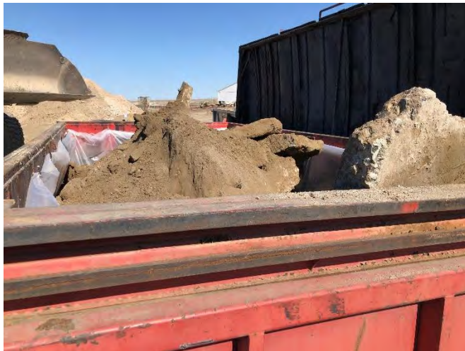
Photo 11. View of broken concrete in dumpster. Photo taken on March 11, 2021.
