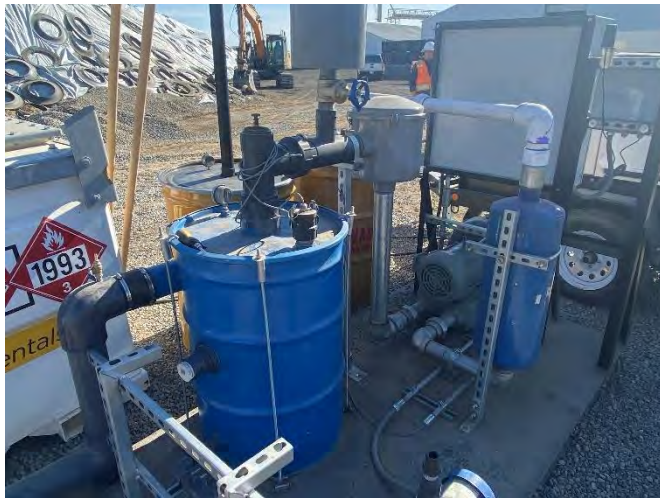
Photo 19. View of SVE treatment system skid. Photo taken on June 1, 2022.
