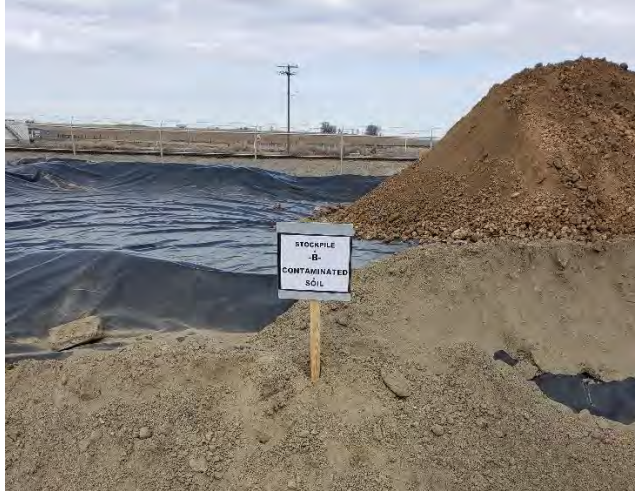
Photo 5. Detail of signage used to label contaminated soil stockpile during excavation activities.
