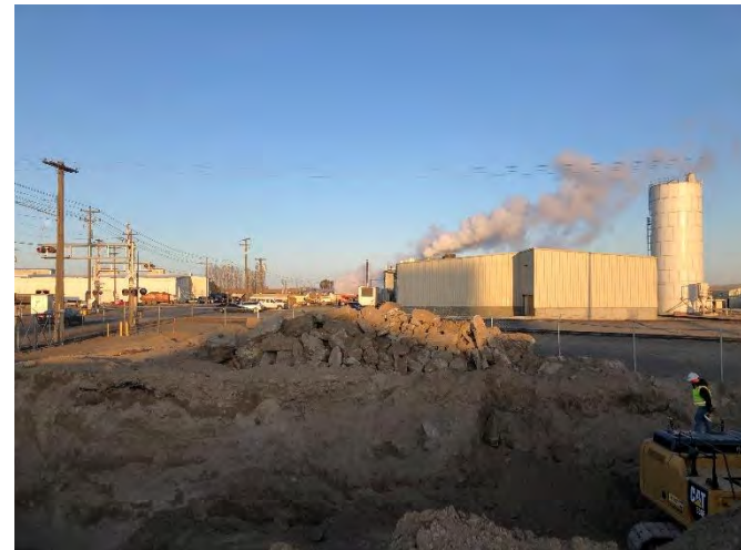
Photo 12. View of broken concrete stockpile near western fence line. Concrete was disposed of at the Waste Connections Landfill in The Dalles, OR. Photo taken on March 30, 2021, facing west.
