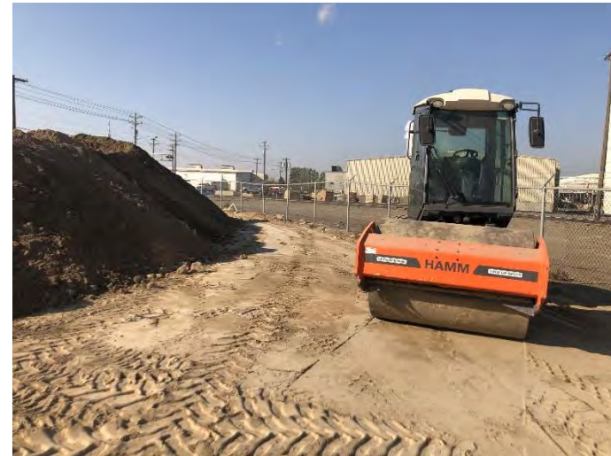
Photo 24. View of compaction activities in north portion of west pit. Photo taken on October 20, 2021.
