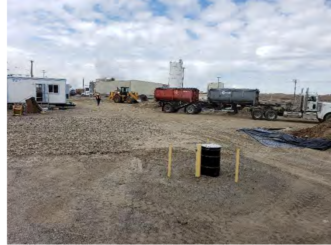
Photo 6. View of contractor's trailer, rock track pad, and MW-6S. Photo facing west, taken on March 10, 2021.
