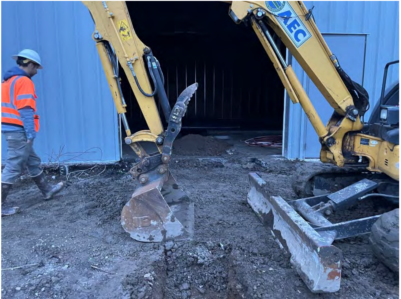
Figure 9: Outside overview of SVE Building trench at end of workday, 01/26/2023, facing North
