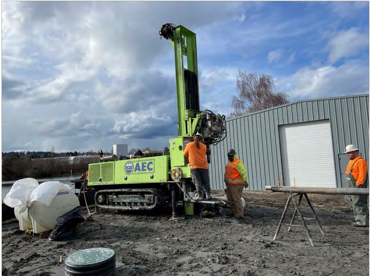
Exhibit A-16: Photo of the Sonic Drill Rig to the South of the AS/SVE Building, Looking Northwest
