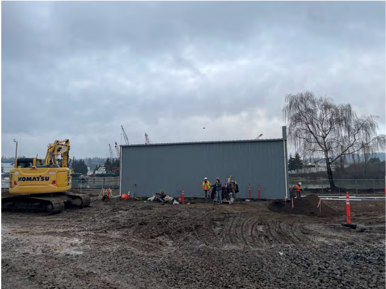
Figure 1: Overview of AS/SVE Building that separates the southern and northern trenches, facing West. Trenches are approximately 10 feet east of Duwamish River
