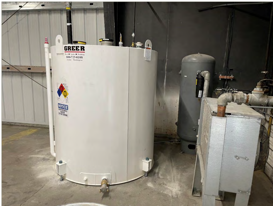
Exhibit A-14: View of the Storage Tank Inside of the AS/SVE Building, Looking East
