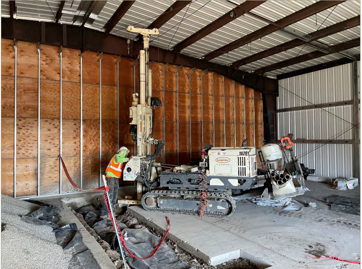
Exhibit A-17: Photo of the Direct-Push Drill Rig Inside of the AS/SVE Building, Looking Northeast
