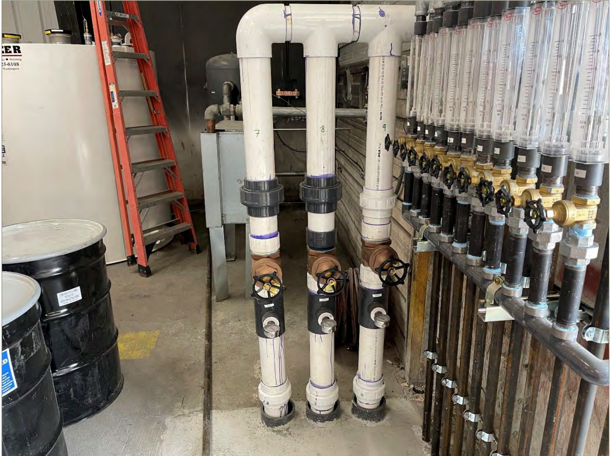
Exhibit A-9: View of the Three SVE Extension Pipes Inside of the AS/SVE Building, Looking East
