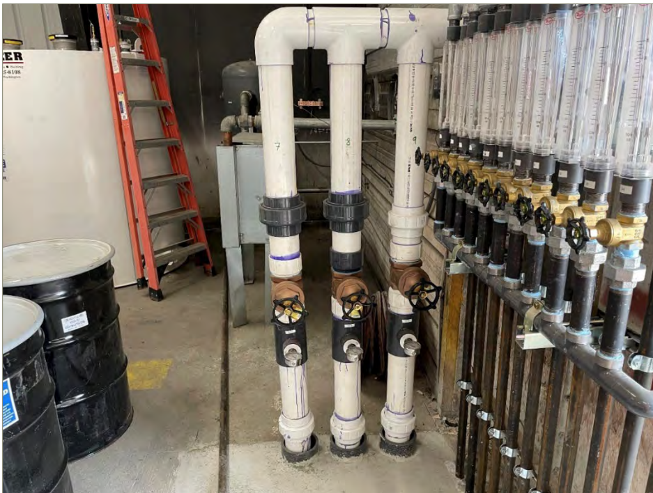
Exhibit 5-2: View of the Three SVE Extension Pipes Inside of the AS/SVE Building, Looking East
