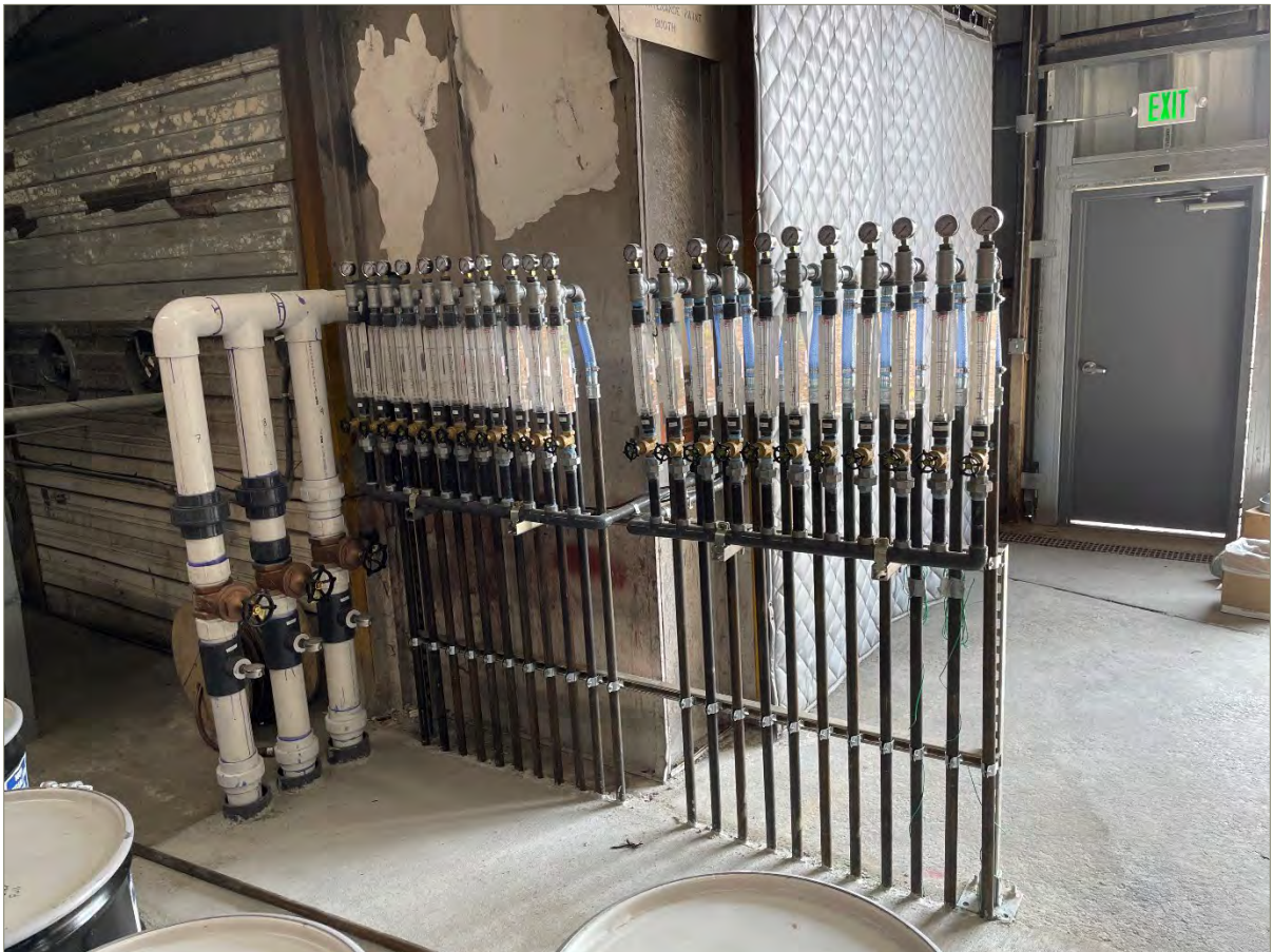
Exhibit 5-1: View of the 22 AS Extension Lines Inside of the AS/SVE Building, Looking Southeast
