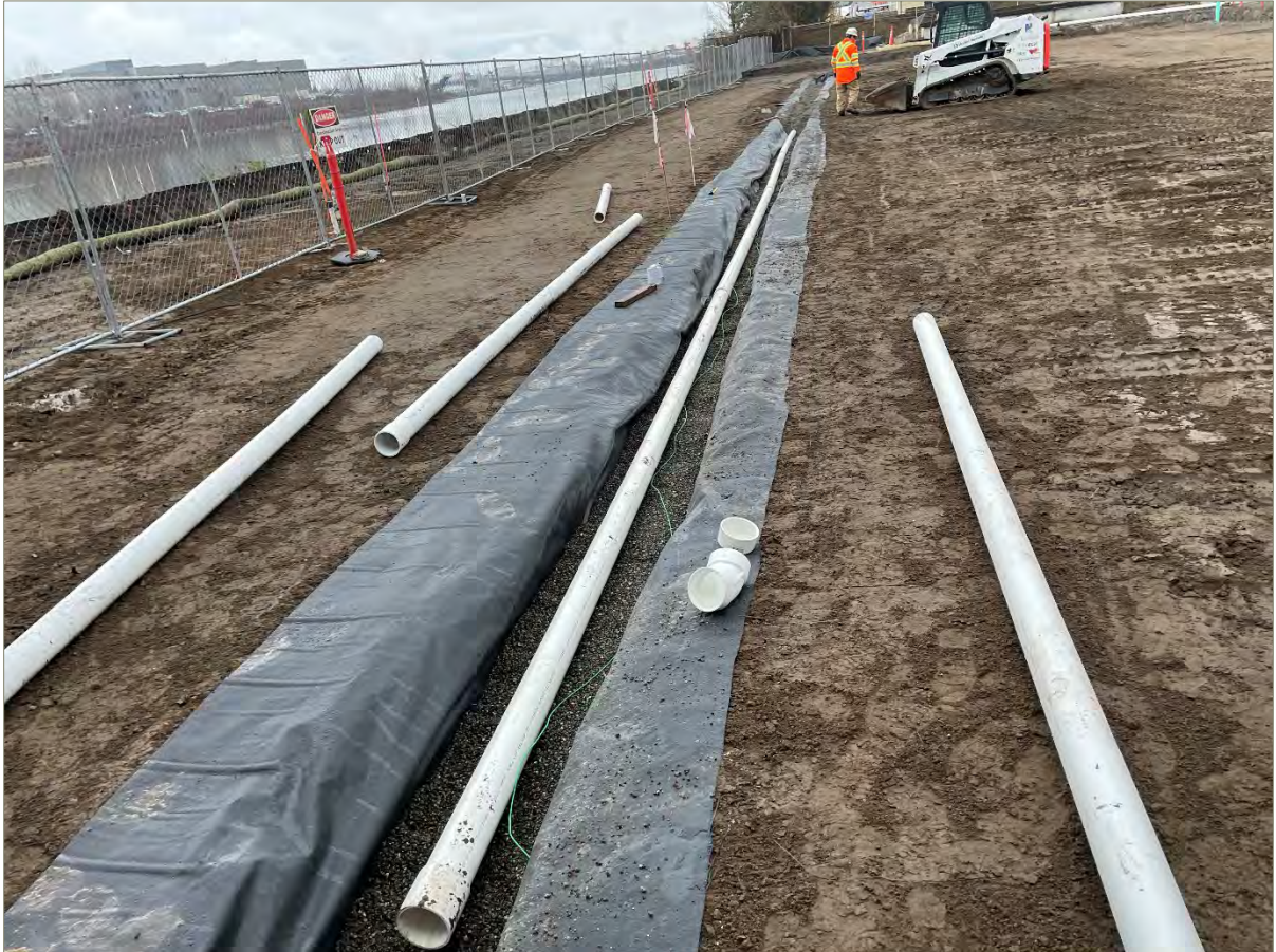
Exhibit A-8: Photo of Construction of the SVE Extension Located North of the AS/SVE Building, Looking North
