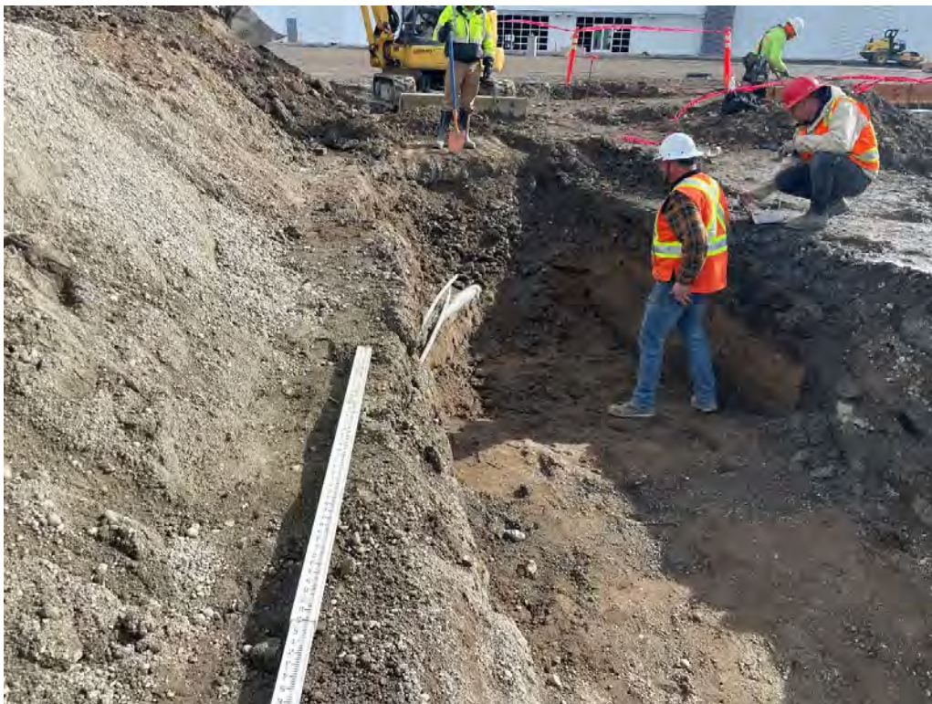
Figure 97: Exposure of Set of Pipes Unaffiliated with this Project
