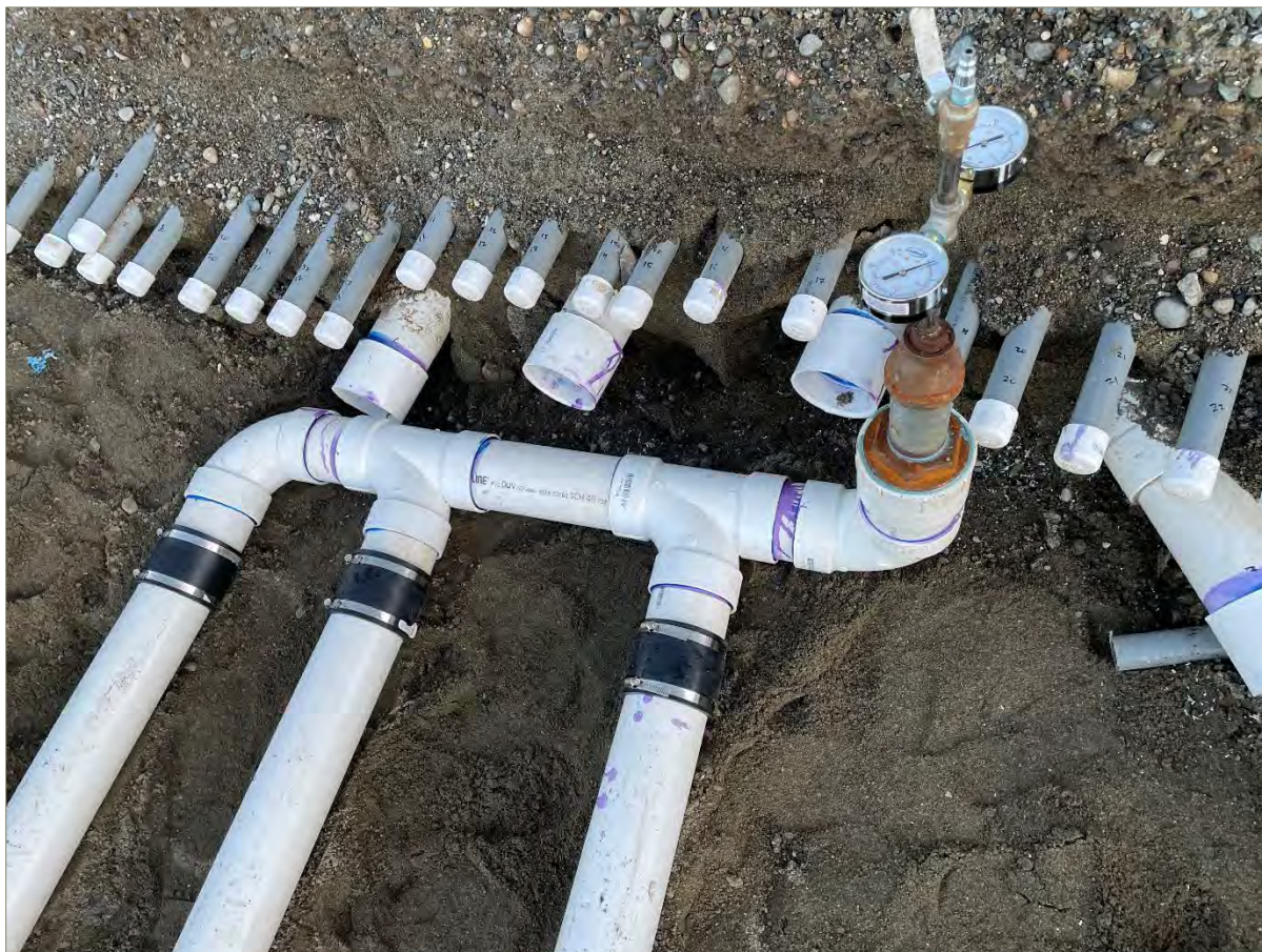
Exhibit A-19: Photo of Temporary Manifold and Test Gauges Attached to SVE Lines in the Replumbed AS/SVE Trench
