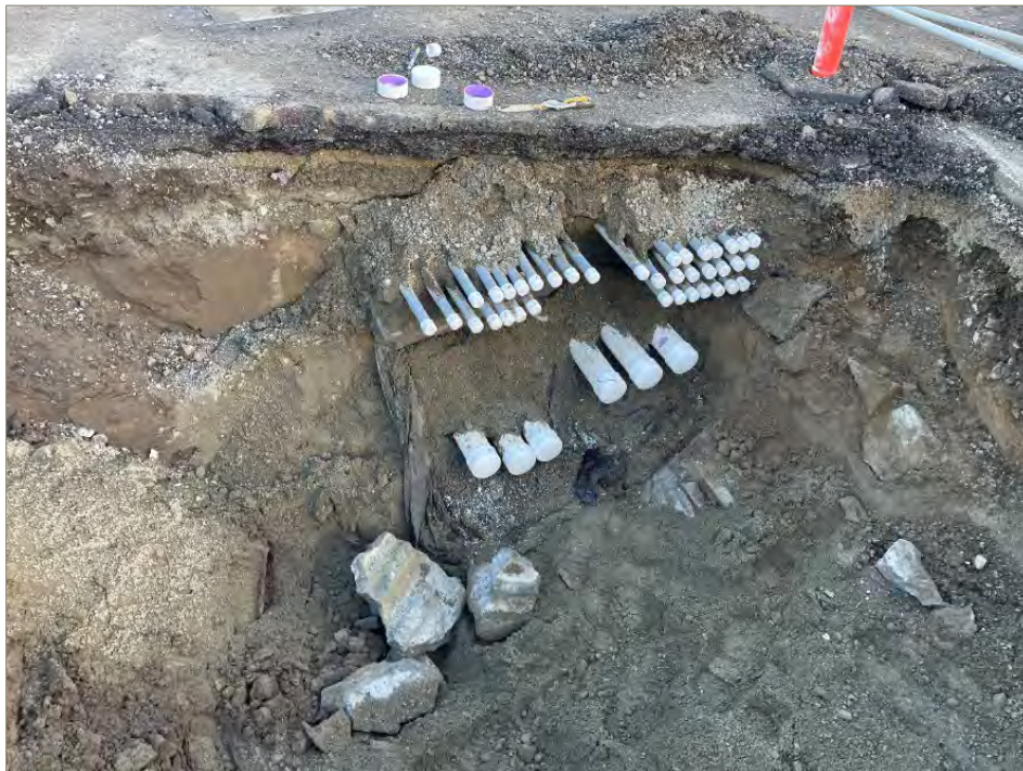
Exhibit A-11: View of the East Terminus of the Disconnected and Capped AS/SVE Pipes, Looking East
