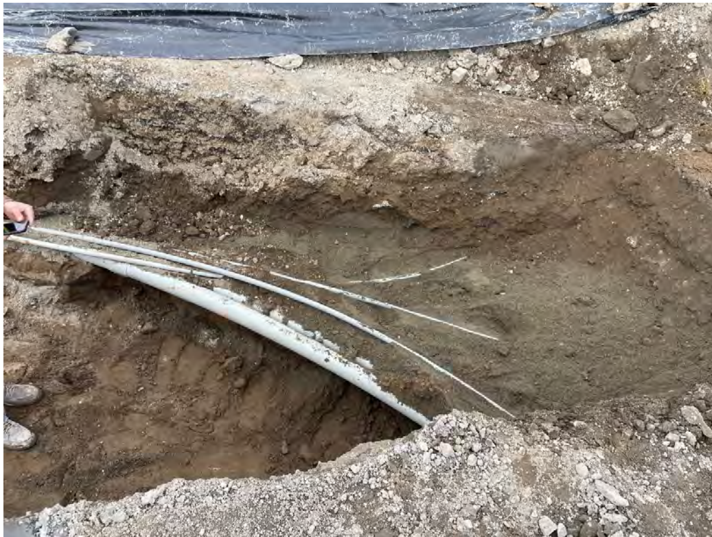
Figure 101: Unaffiliated Pipes Exposed After Concrete Layer is Removed
