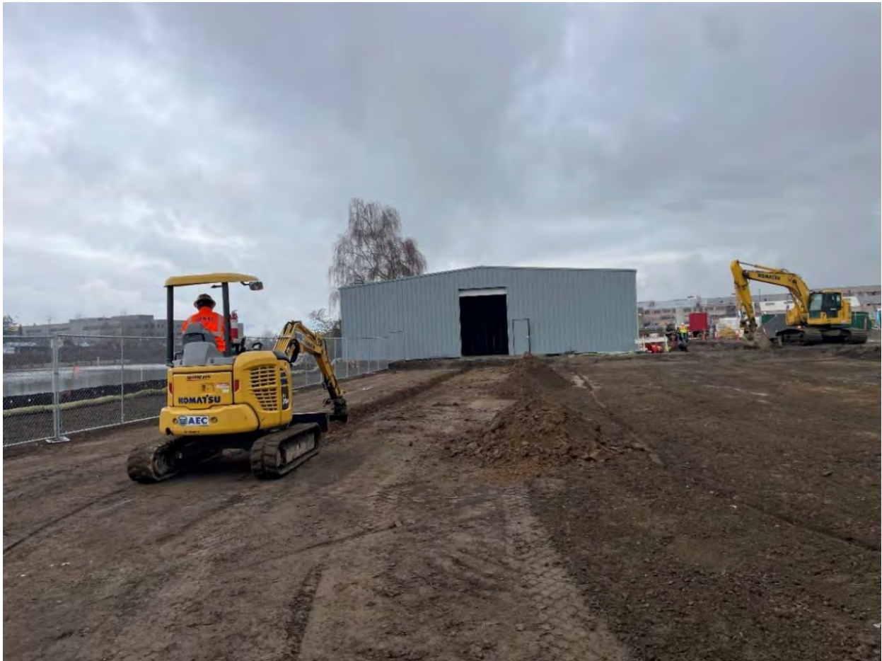
Figure 5: Overview of southern trench during excavation when monitor arrived on site, facing North
