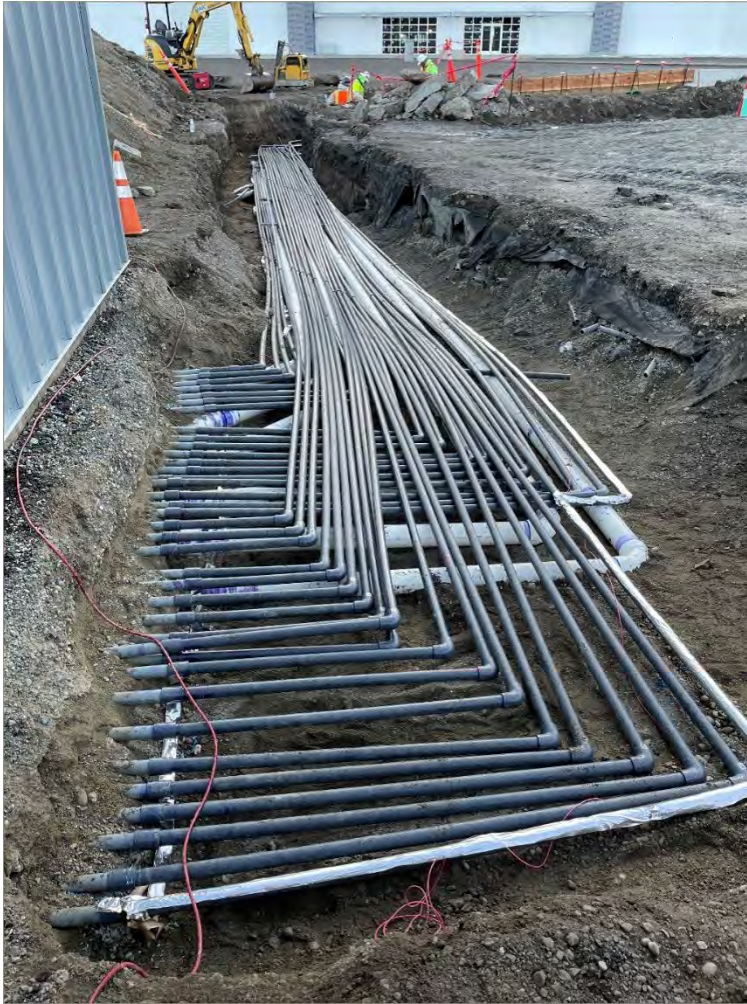
Exhibit A-13: New Replumbed AS/SVE Lines, Looking East
