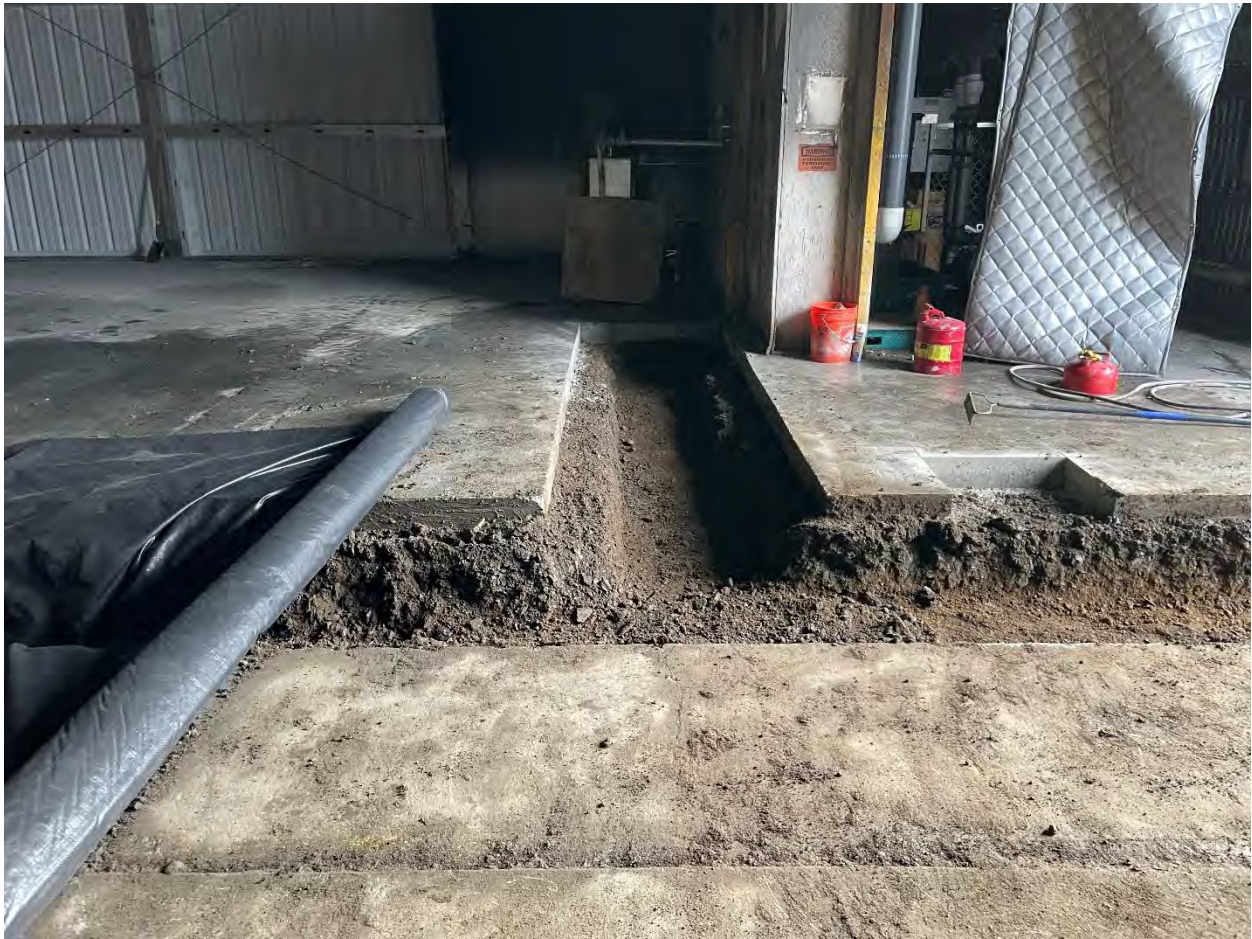
Figure 12: Overview of AS/SVE Building trench branch at completion of excavation, facing East
