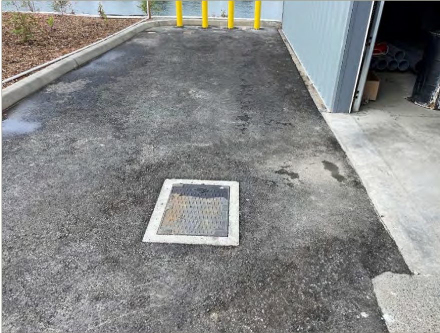
Exhibit A-3: Photo of an AS Wellhead Concrete Vault to the South of the AS/SVE Building, Looking West
