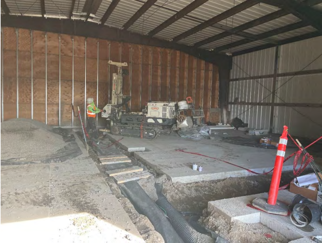
Figure 59: Overview of AS/SVE Building Before Drilling
