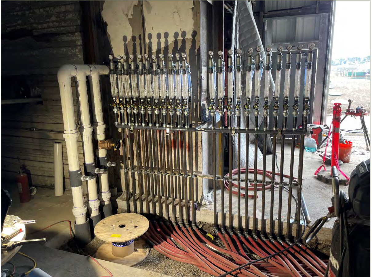
Exhibit A-5: View of the Aboveground AS Extension Components Inside of the AS/SVE Building
