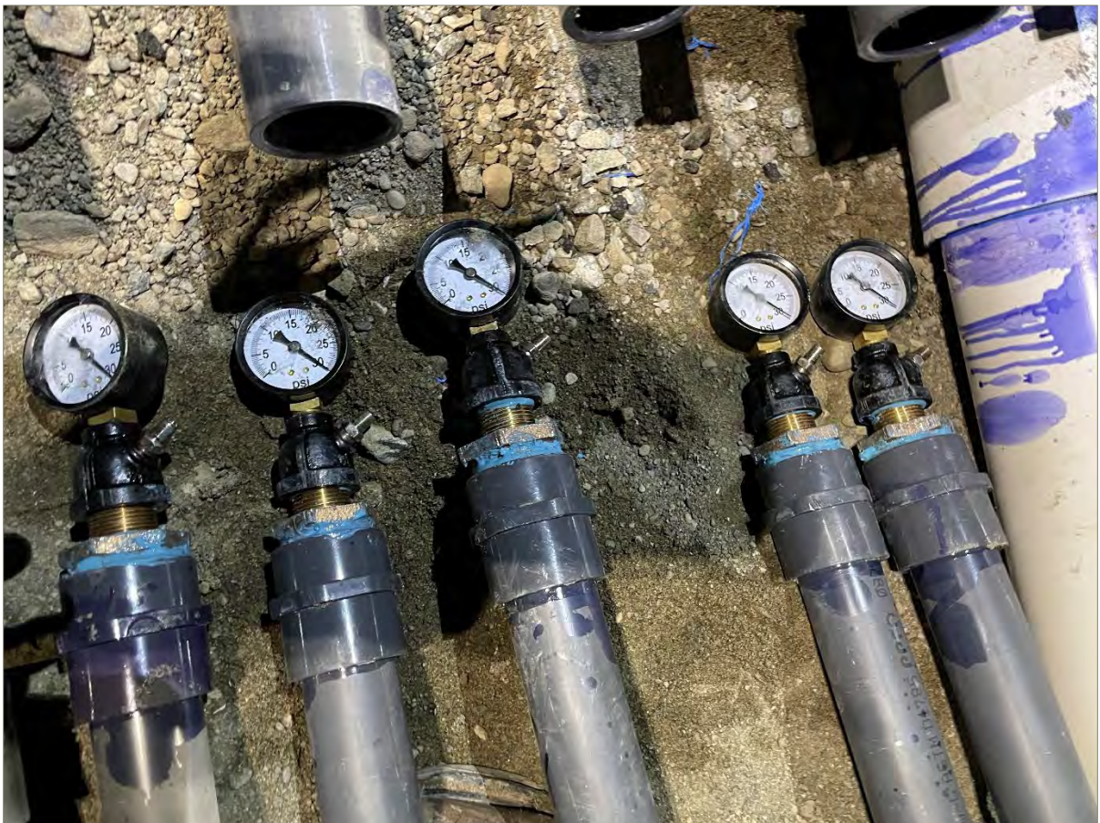
Exhibit A-18: Photo of Test Gauges Attached to AS Lines in the Replumbed AS/SVE Trench
