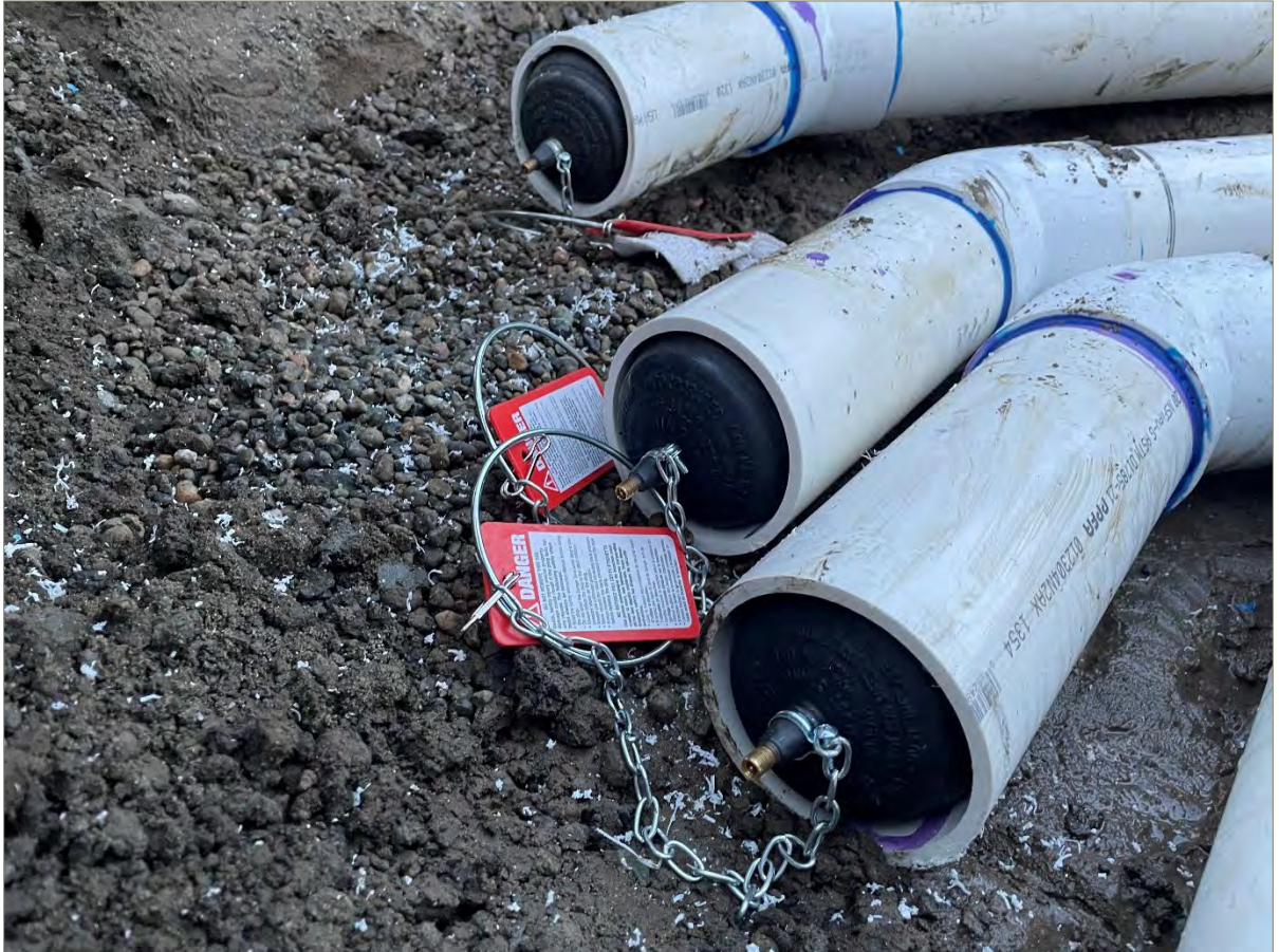
Exhibit A-20: Photo of Temporary Plugs Attached to SVE Lines in the Replumbed AS/SVE Trench
