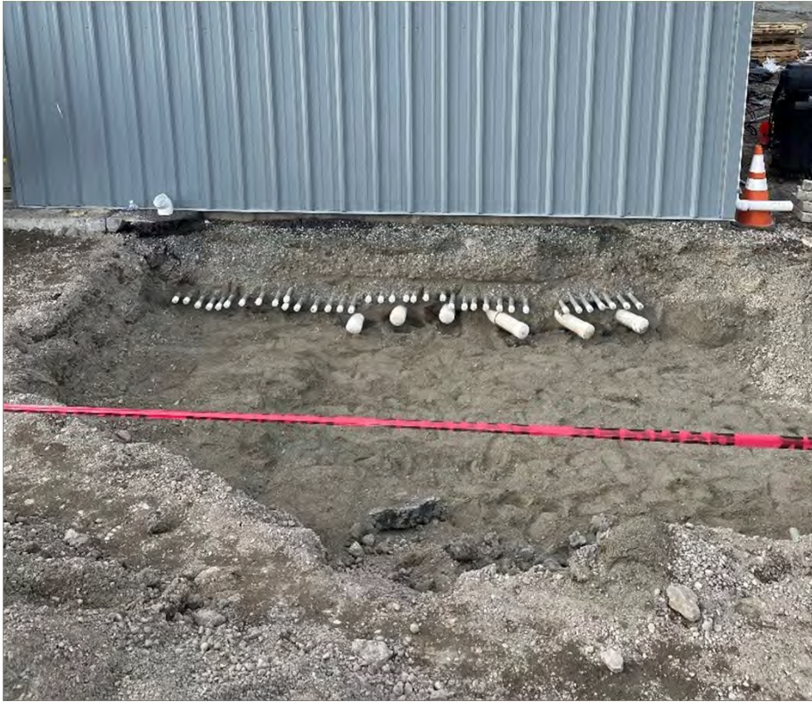
Exhibit A-12: View of the West Terminus of the Disconnected and Capped AS/SVE Pipes, Looking North
