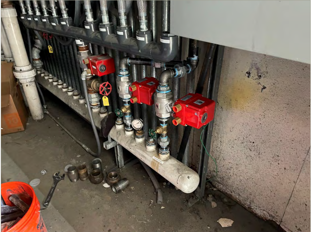
Exhibit A-6: View of Ball Valves BV-4 and BV-5 Connected to the Main AS Header
