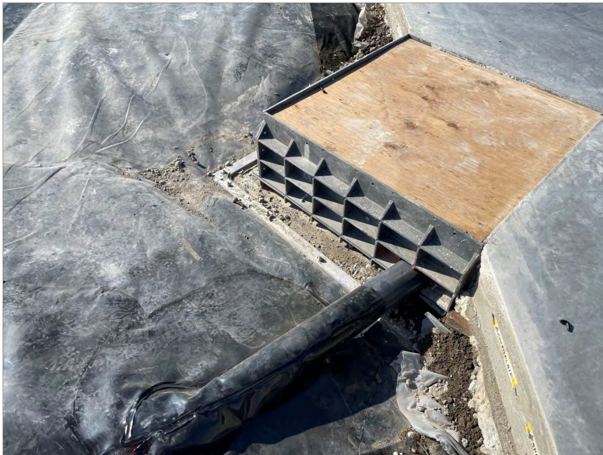
Exhibit 4-5: Riser Pipe Emerging from Underneath the Vapor Barrier and Entering a Column Form
