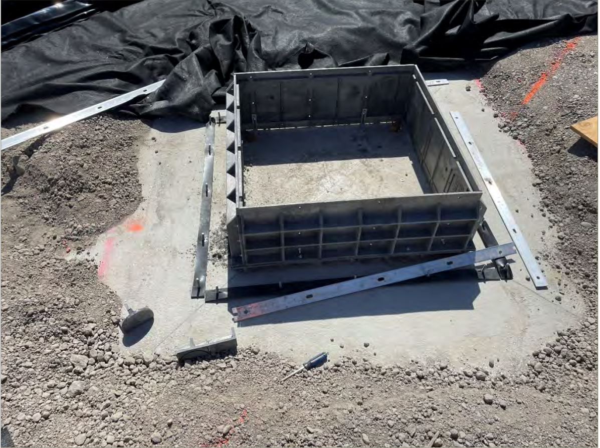
Exhibit 4-4: Batten Strips Anchored to a Column Footing (Prior to Attachment of the Vapor Barrier)
