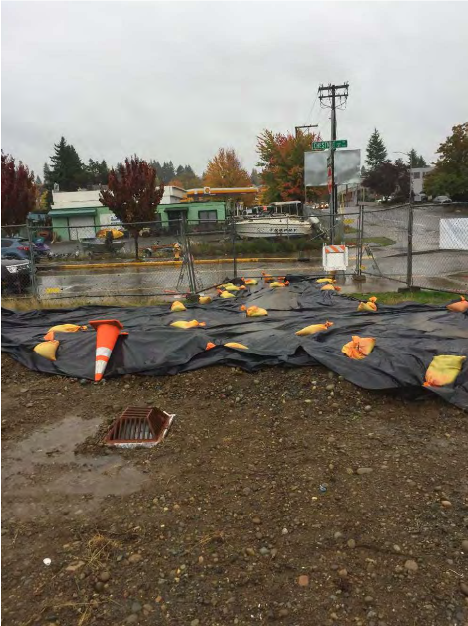
Photo 1 – Turbidity Sample Location 1 – Outside of Parcel 2/3 – Water on plastic sheeting @ sidewalk cut on Chestnut Street.
