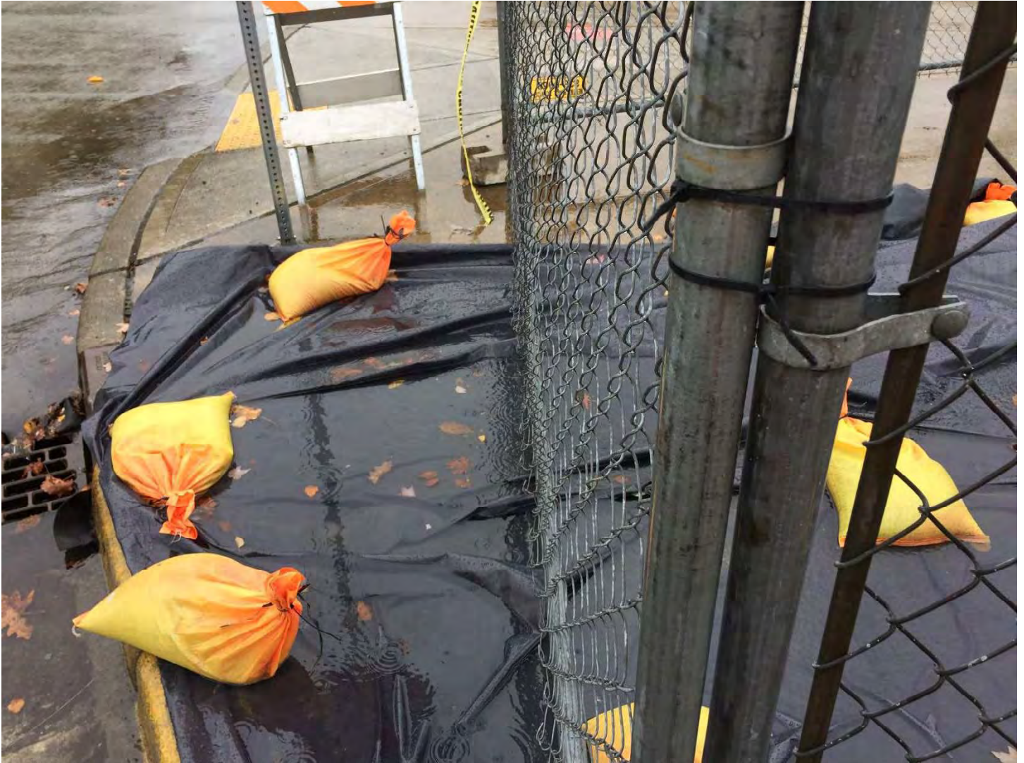
Photo 1 – Turbidity Sample Location 1 – Outside of Parcel 2/3 – Water on plastic sheeting @ sidewalk cut on Chestnut Street
