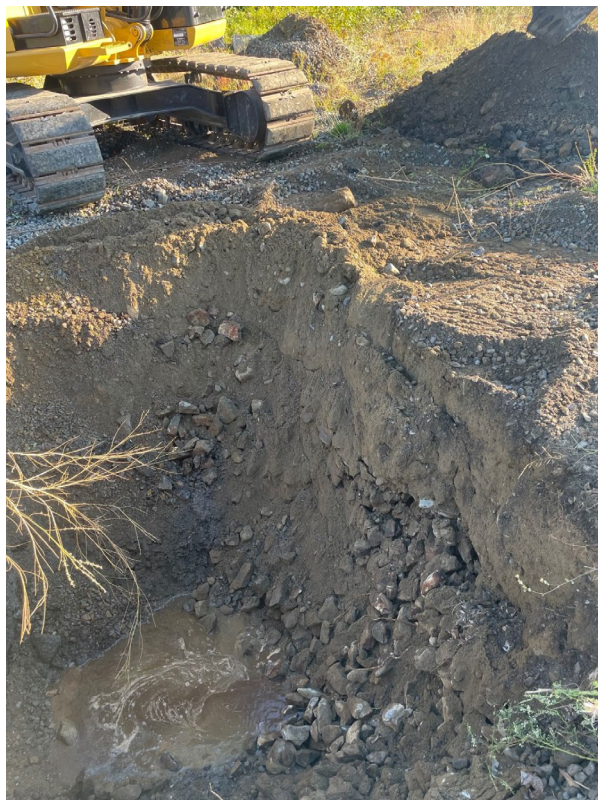
Photograph 4. 2016 excavation quarry spall backfill ~4 feet north and east of MW-04 (facing NE)
