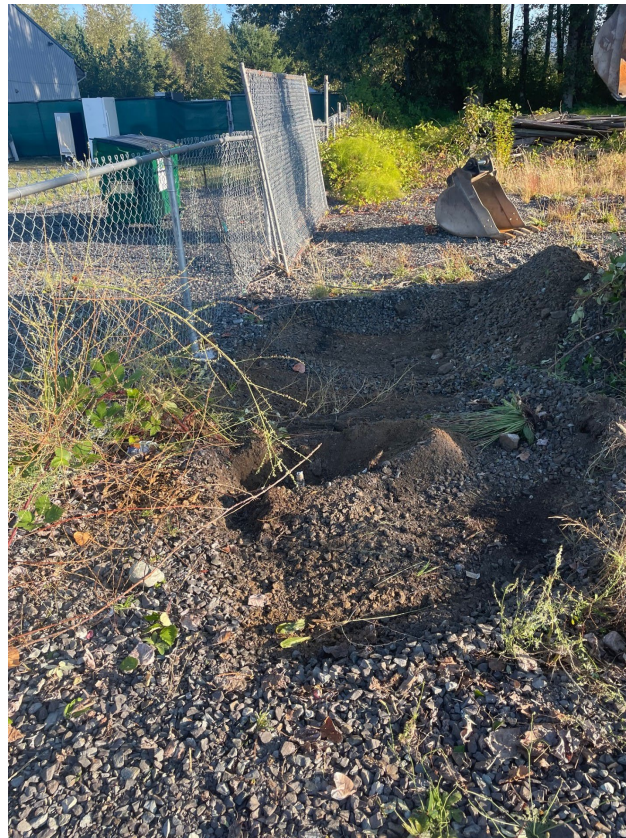
Photograph 2. Surface soil removal from fence line to north, east and south (facing N)
