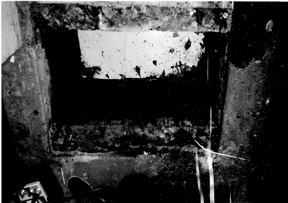
26 Close-up of the sump; note the absorbent pad.
