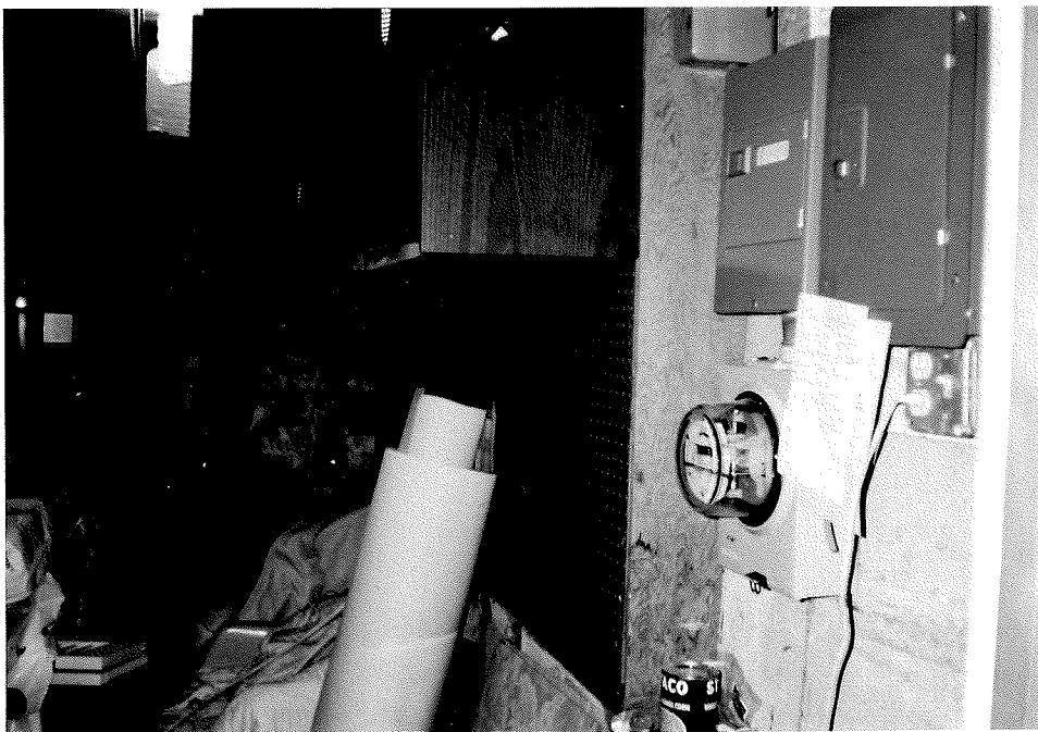
24 View to the east of the storage room located east of the laundry room in the basement of the Monterey Apartments.
