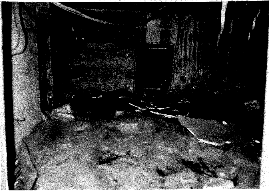
37 View to the north of the crawl space of the Del Roy Apartments.
