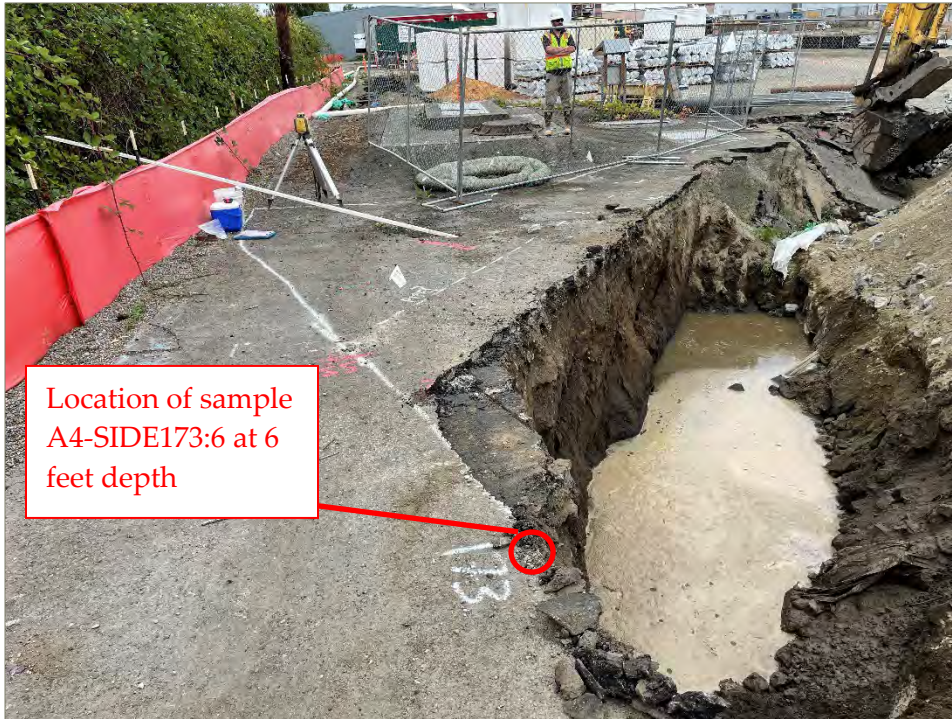
Exhibit A-13: Excavation Activities at Northwest Sidewall of Area 4. Photo taken on August 26, 2022. View direction is north.
