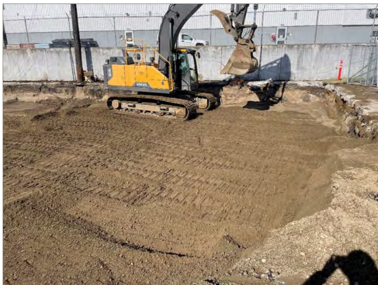
Exhibit E-1: Photo of Gravel Borrow Delivered to Area 1 on the 8801 Property
