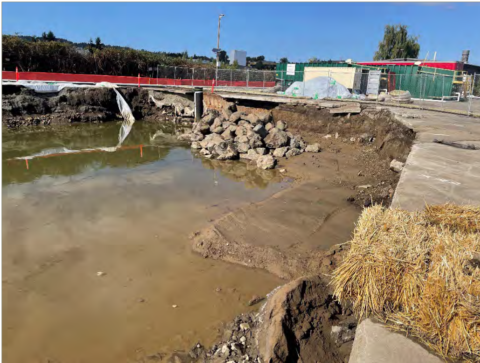
Exhibit A-18: Area 5 – View of the North Portion of the Excavation. Photo taken on October 1, 2021. View direction is northwest. Water in the excavation is groundwater and was later removed and treated. Rocks were part of support for the sheet pile wall that is in the north west corner of the excavation.
