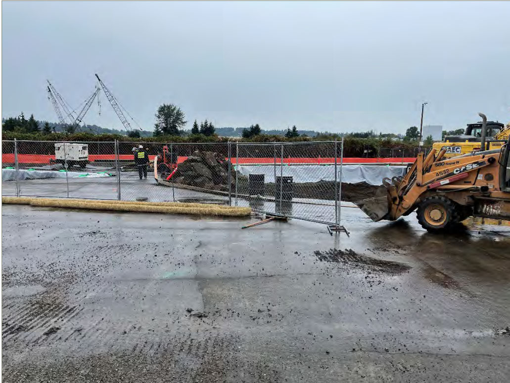
Exhibit B-4: Photo of Area 4 (left) and Area 5 (right) on September 17, 2021 View direction is west. Straw wattles are shown around the excavation perimeter. White plastic sheets are shown on excavation sidewalls. An orange silt fence is shown on the property boundary.
