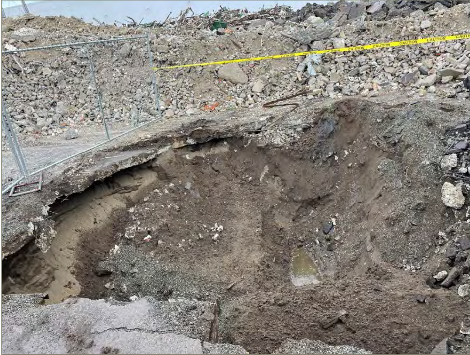
Exhibit A-25: Area 7 – View of the North Sidewall Final Extent. Photo taken on October 6, 2021. View direction is north. Groundwater was observed in the excavation bottom.
