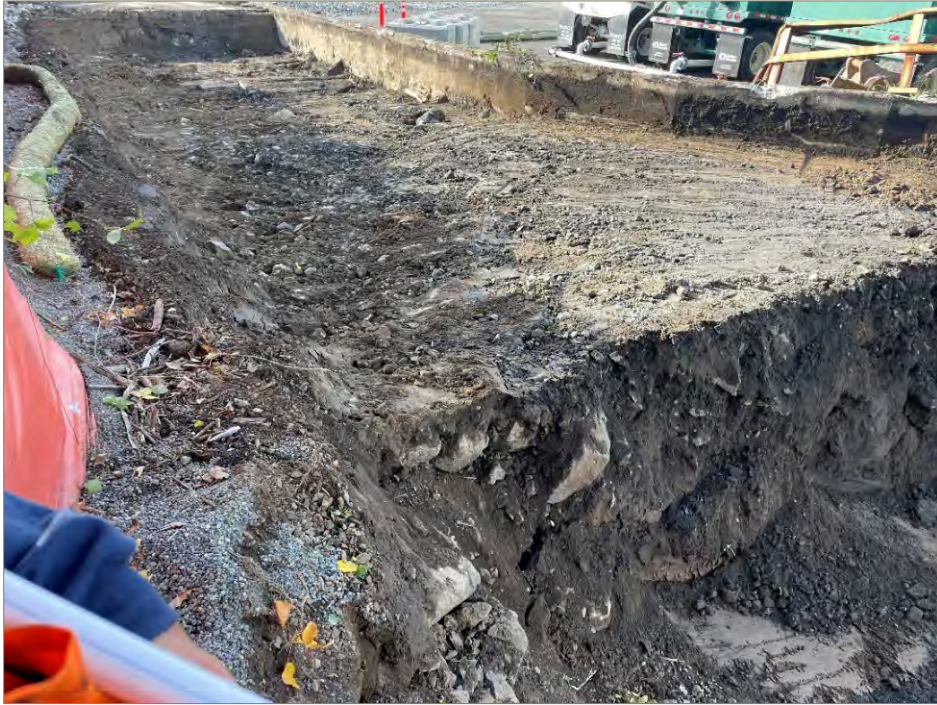
Exhibit A-9: Area 3 – View of the West Portion of the Excavation. Photo taken on September 28, 2021. View direction is northwest. The excavation was later expanded. Large rocks and concrete are visible in the sidewalls shown at the center of the photo and into the background. The large rocks and concrete are part of the shoreline berm.
