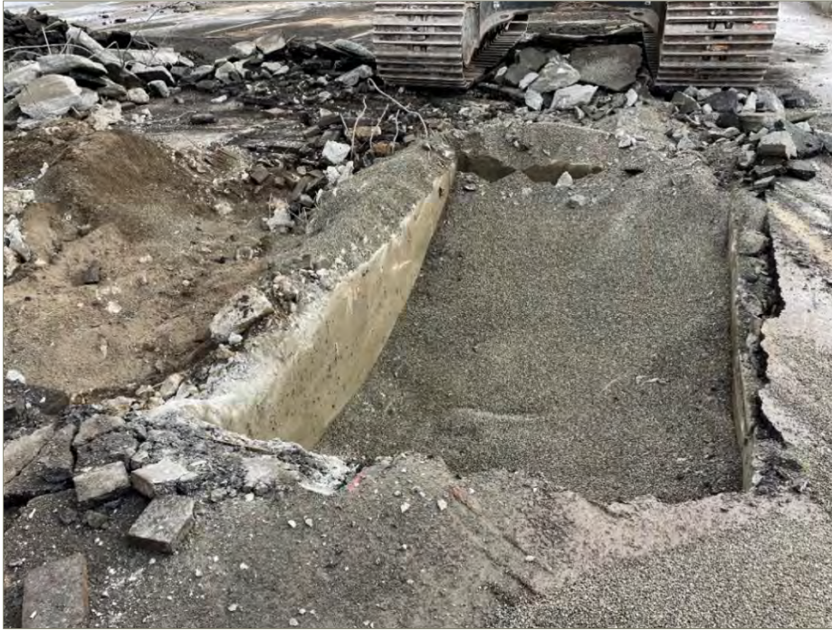
Exhibit A-21: Area 7 – View of the Pavement Removal Over the Excavation. Photo taken on October 4, 2021. View direction is east. A concrete vault filled with pea gravel is shown in the south (right) half of the excavation.
