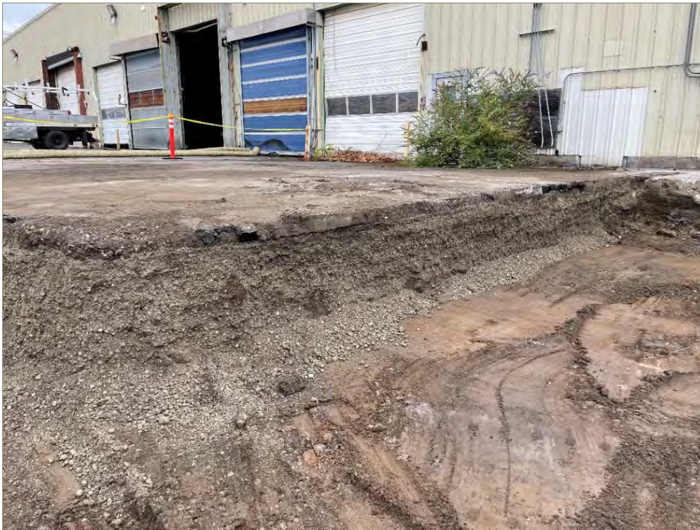
Exhibit A-6: Area 2 – View of the Northeast Portion of the Excavation. Photo taken on September 20, 2021. View direction is northeast.
