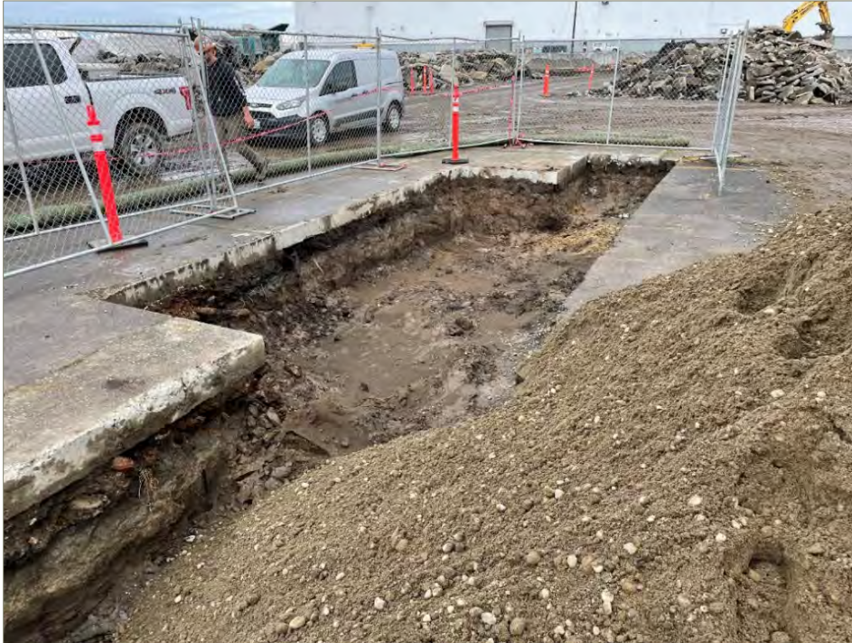
Exhibit A-7: Area 2 – View of the North Portion Final Extent of the Excavation. Photo taken on November 3, 2021. View direction is northwest. Imported Gravel Borrow is shown in the center and right foreground.
