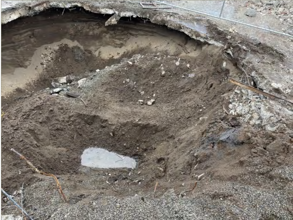
Exhibit A-23: Area 7 – View of the West Sidewall Final Extent. Photo taken on October 6, 2021. View direction is west. Groundwater was observed in the excavation bottom.
