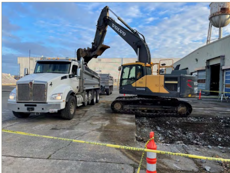
Exhibit B-1: Photo of Excavation at Area 2 on September 20, 2021. View Direction is North.
