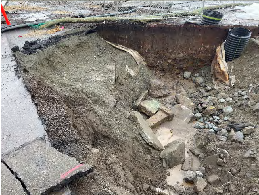
Exhibit A-19: Area 5 – View of the Northwest Corner Final Extent of the Excavation. Photo taken on November 4, 2021. View direction is north. The visible large rocks are concrete blocks that are part of the shoreline berm and were left in place. A portion of sheet pile wall is shown extending into the excavation. A plastic pipe for the sump is shown in the top right corner of the photo and was later removed. Imported Gravel Borrow is shown on the right side of the photo.
