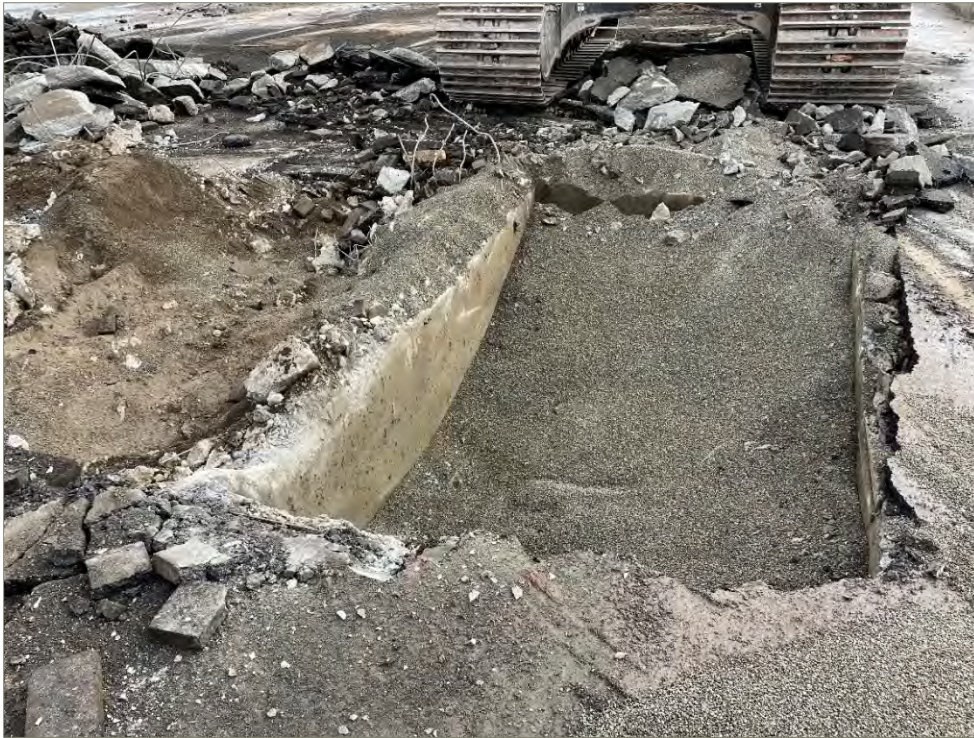
Exhibit 5-9: Area 7 – View of the Vault Uncovered After Pavement Was Removed from the Excavation. Photo taken on October 4, 2021. View direction is east. A concrete vault filled with pea gravel is shown in the south (right) half of the excavation.
