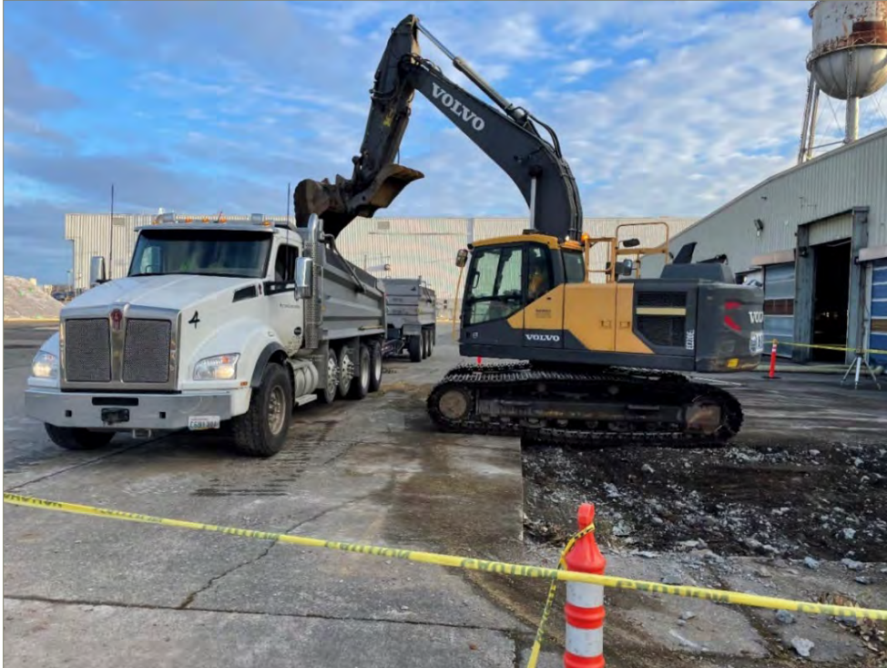
Exhibit A-4: Area 2 – Excavation and Hauling. Photo taken on September 20, 2021. View direction is north.
