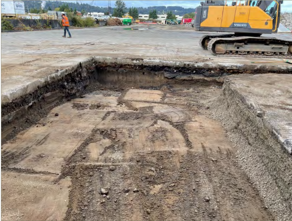
Exhibit A-5: Area 2 – View of the Southwest Portion of the Excavation. Photo taken on September 20, 2021. View direction is North. The shown excavation extents were later expanded.
