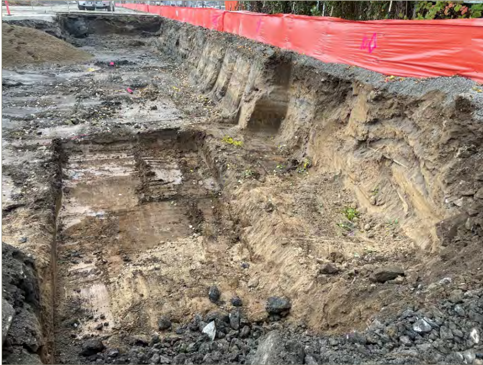
Exhibit A-11: Area 3 – View of the Central Portion of the Excavation. Photo taken on October 18, 2021. View direction is east. The southeast corner sidewall was expanded.
