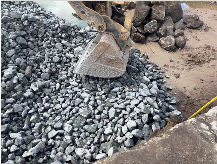
Exhibit E-3: Photo of Quarry Spalls (Foreground) Delivered to Area 5 on the 8801 Property
