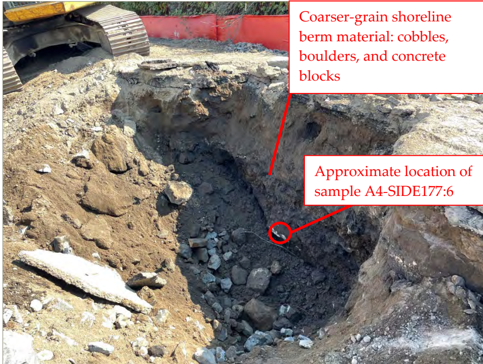
Exhibit A-15: Excavation Activities at Area 4 Sample A4-SIDE177:6. Photo taken on August 31, 2022. View direction is south.
