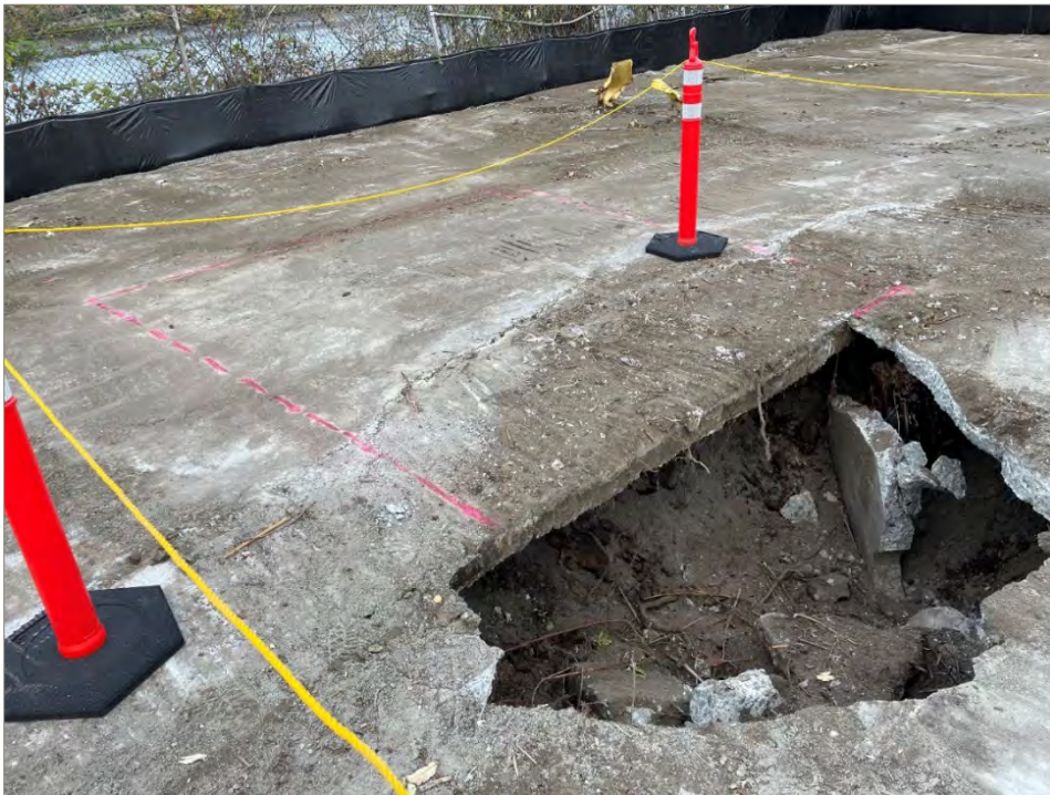
Exhibit A-26: Area 8 – View of the Void in the East Half of the Excavation. Photo taken on October 4, 2021. View direction is northwest. The pink outline shows the extent of that was excavated later.
