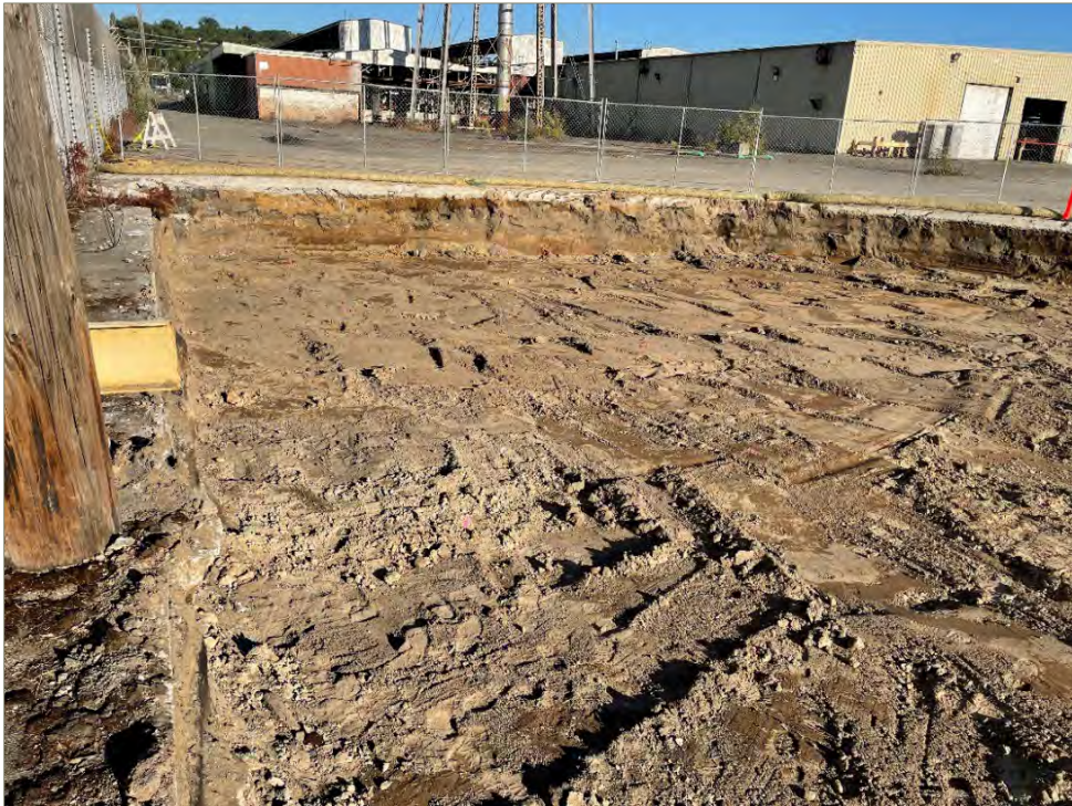
Exhibit A-1: Area 1 – Final Extent of Northeast Corner. Photo taken on September 21, 2021. View direction is east.
