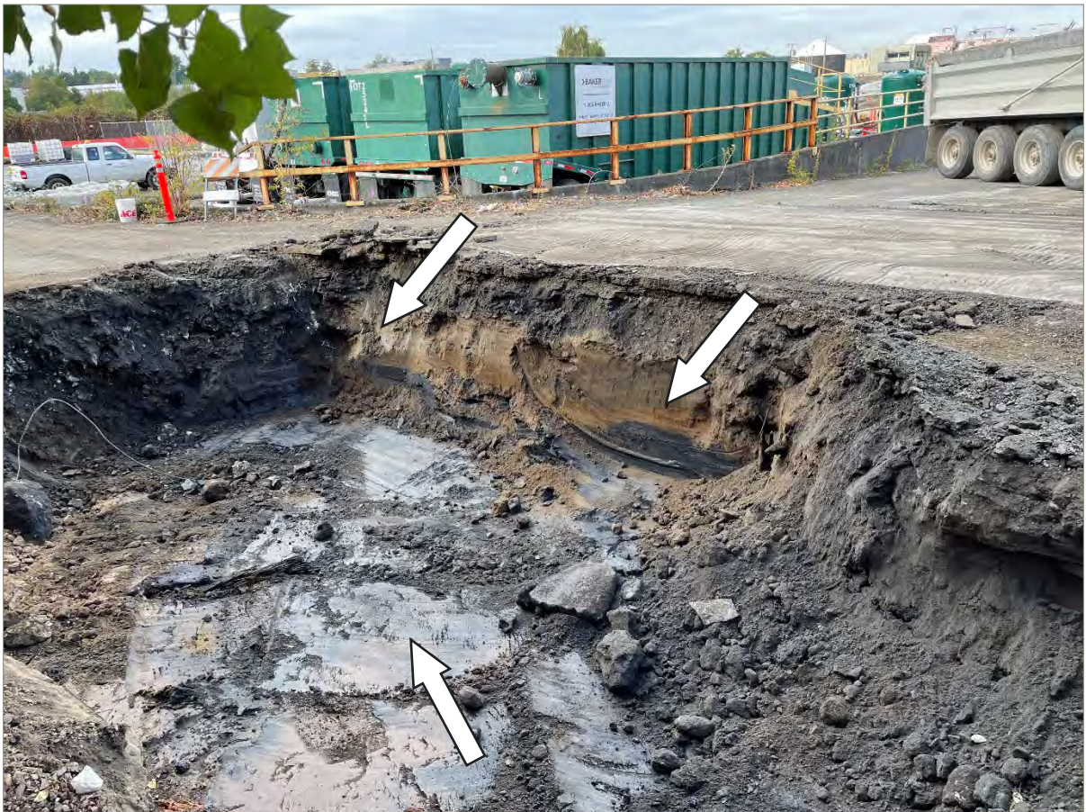
Exhibit 5-3: Photo of the North Portion of Area 3 on September 22, 2021. View direction is northwest. Black-stained soil was observed in the excavation sidewalls and bottom and are identified by white arrows in the photo. The black-stained soil was removed during subsequent expansion of the excavation.
