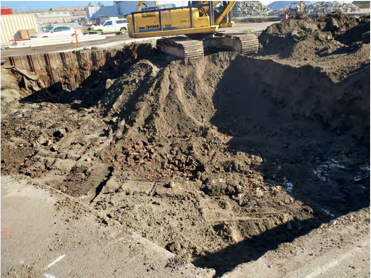
Figure 13. Loosely piled bricks in Area 5
