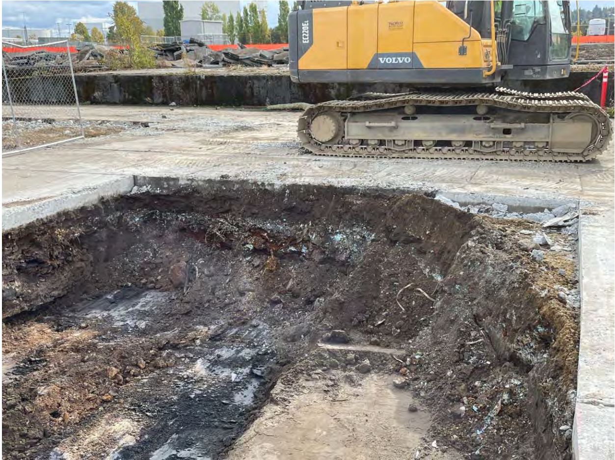
Figure 1. Area 2 Brick and plastic pipe fragments in sidewall
