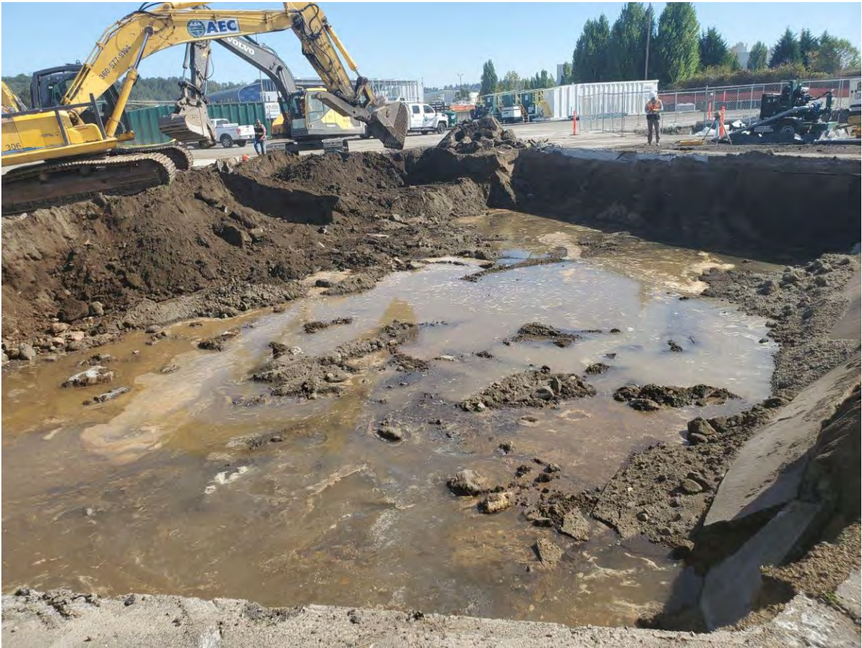
Figure 14. Area 5 inundated with water
