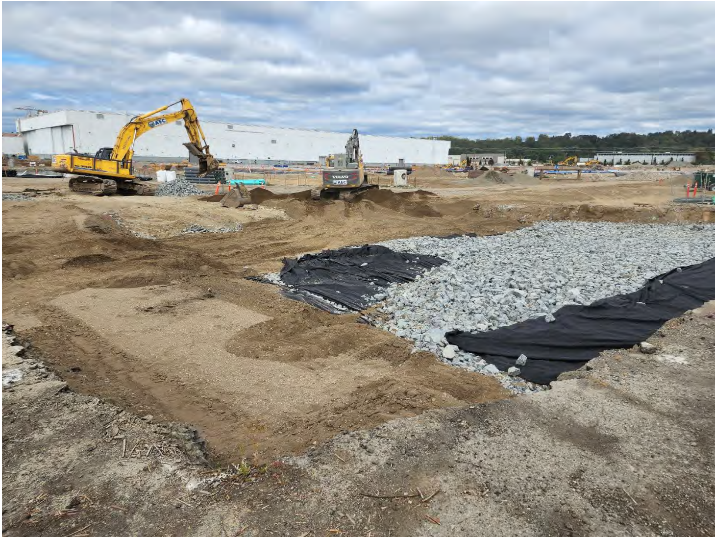
Figure 4. Excavations completed and pit being refilled with quarry spalls on 8/26/22, aspect facing Northeast.
