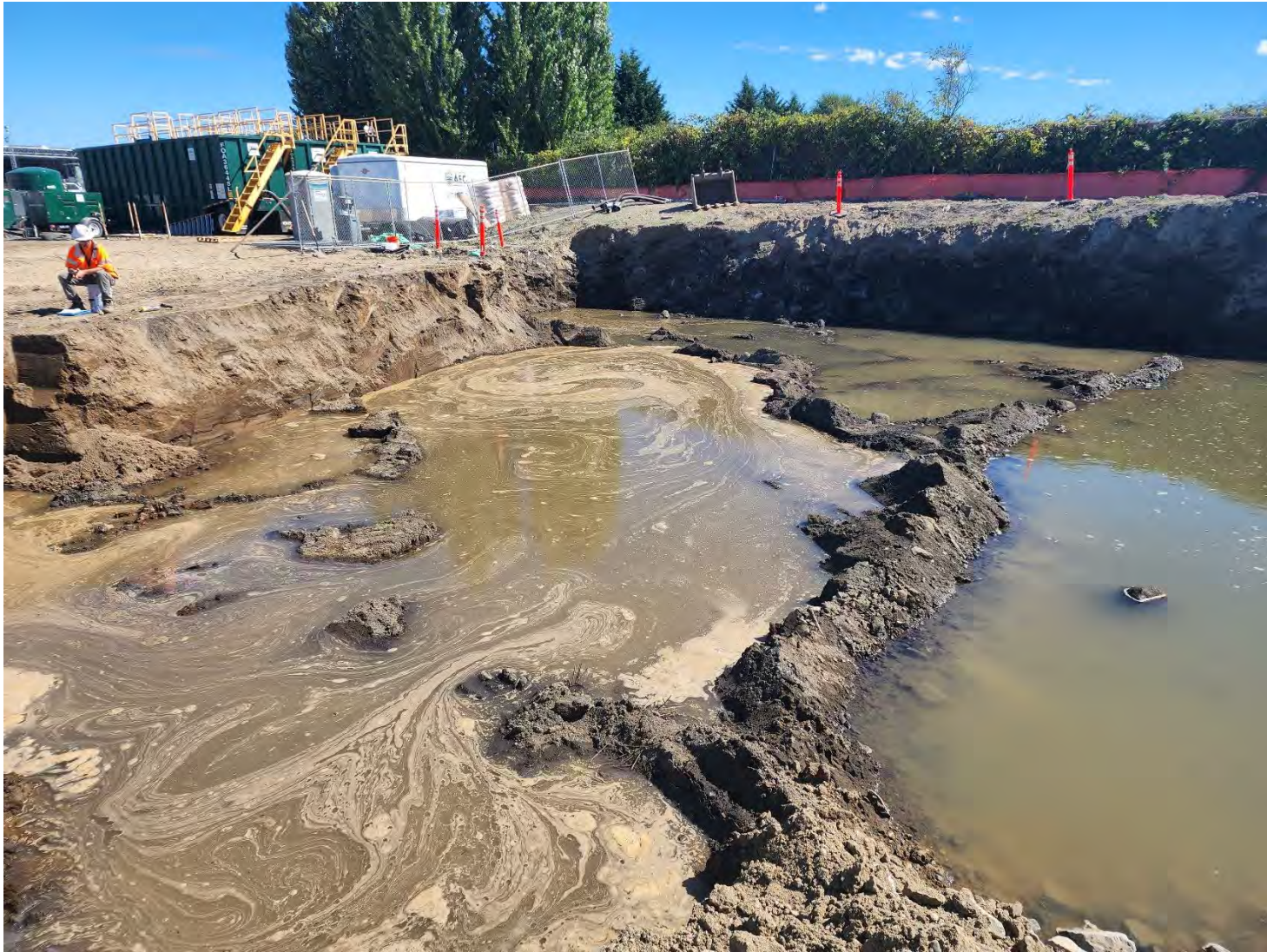
Figure 3. Excavation pit after groundwater breach on 8/22/22, aspect is facing Southeast.
