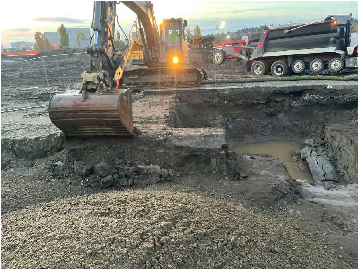
Figure 1. Area 2 Brick fragments and metal
