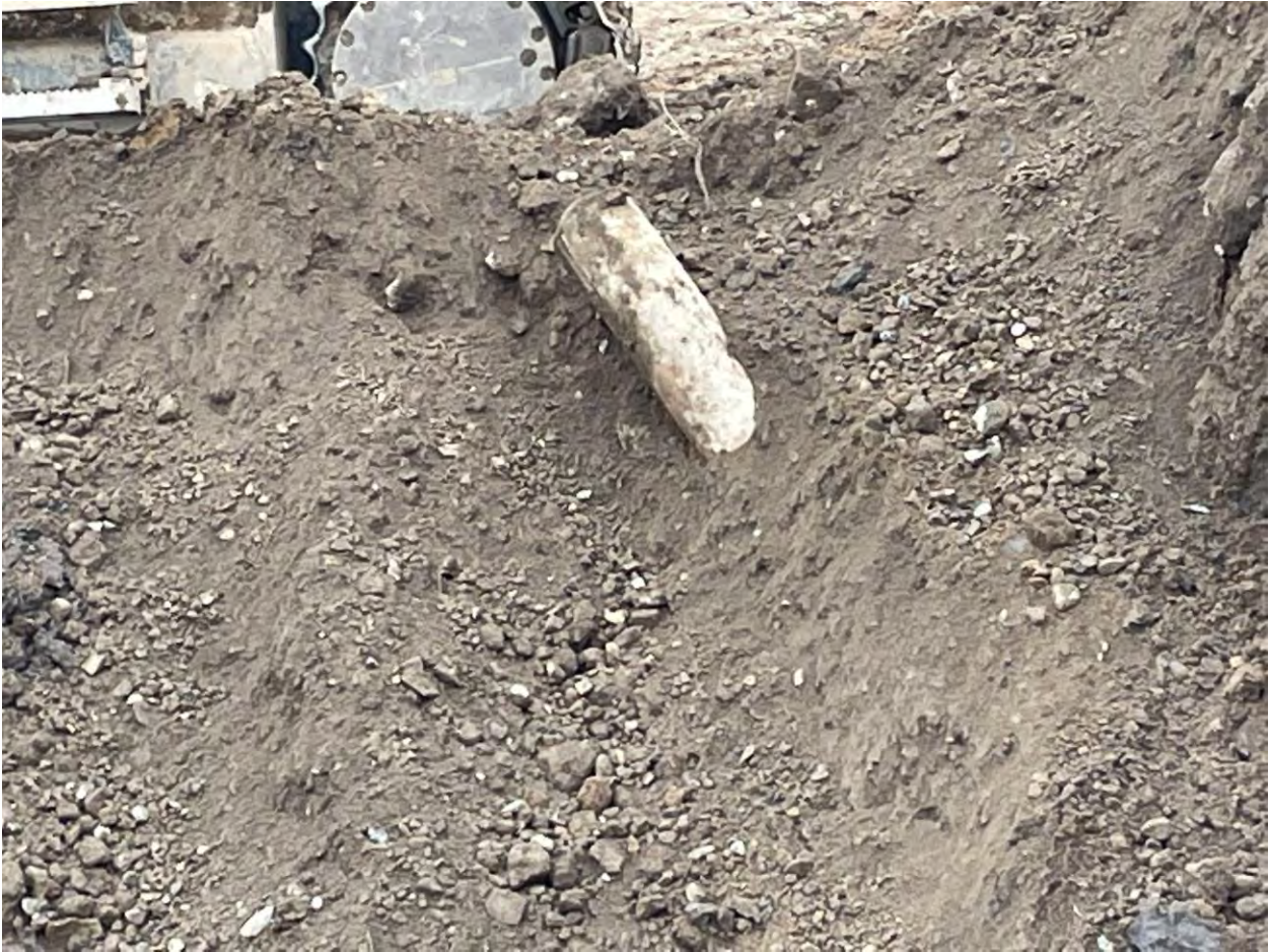
Figure 5. Asbestos pipe from Area 4
