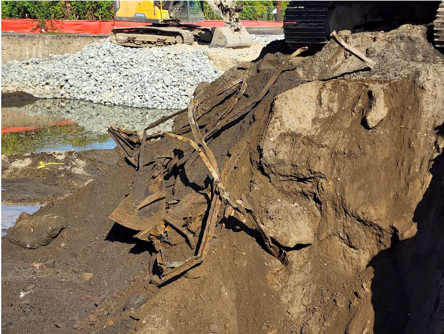
Figure 2. Metal debris observed during excavations on 8/22/22, aspect facing North.
