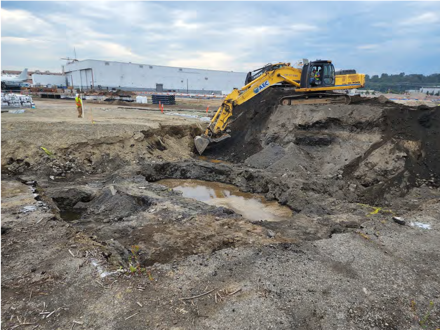
Figure 2. Extent of excavation as of 8/18/2022. Photo taken from the SW corner of the property facing NE.
