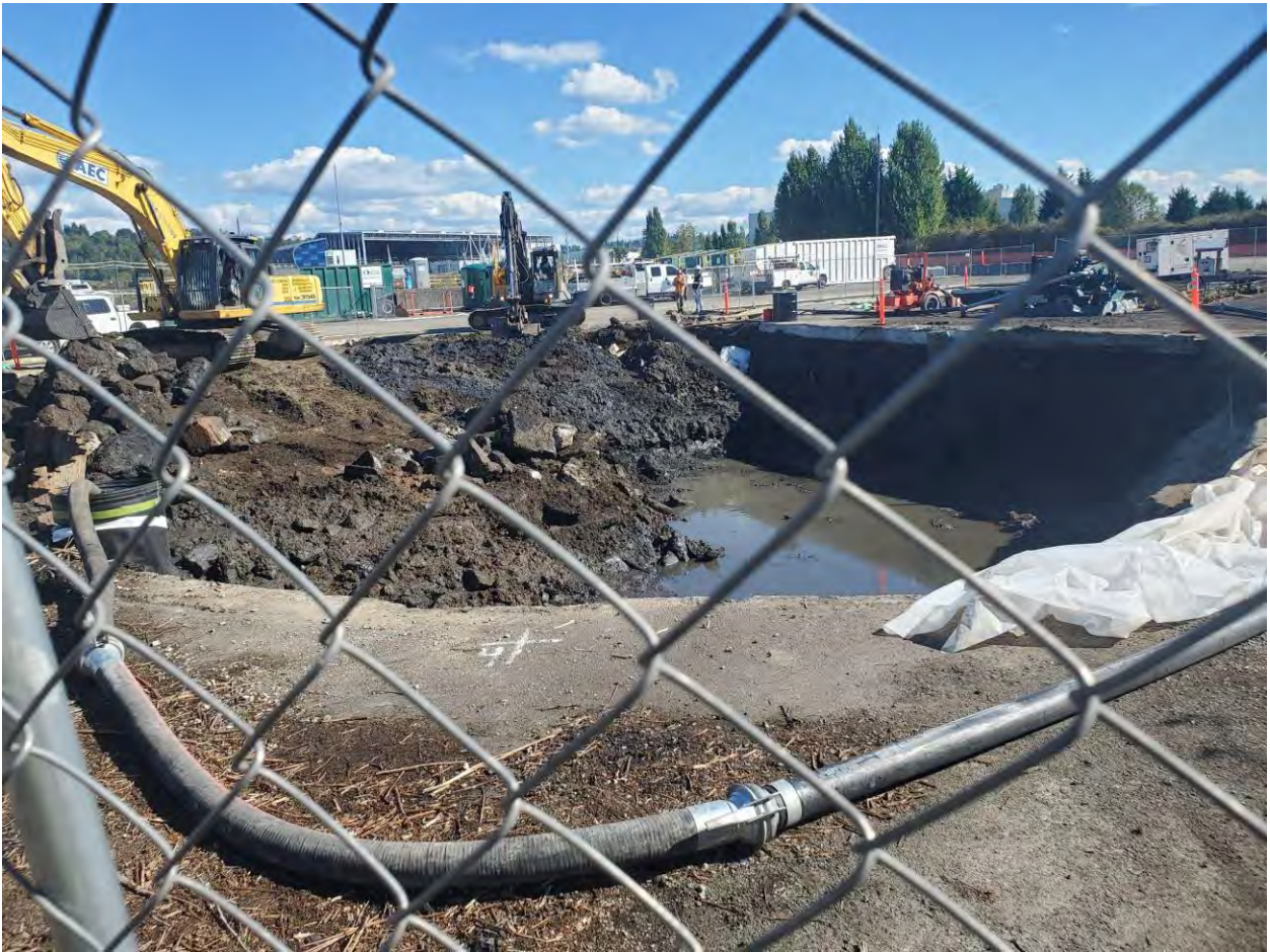
Figure 5. Area 5 inundated with water
