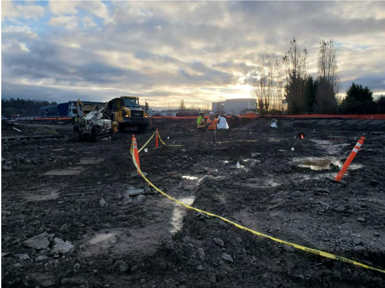
Figure 3. Standing water, muddy surfaces throughout most of drilling areas
