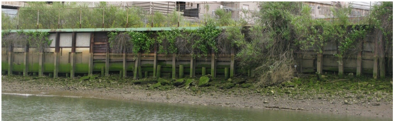
Figure 3 Port of Seattle's wooden bulkhead on the northern side of the Site.
