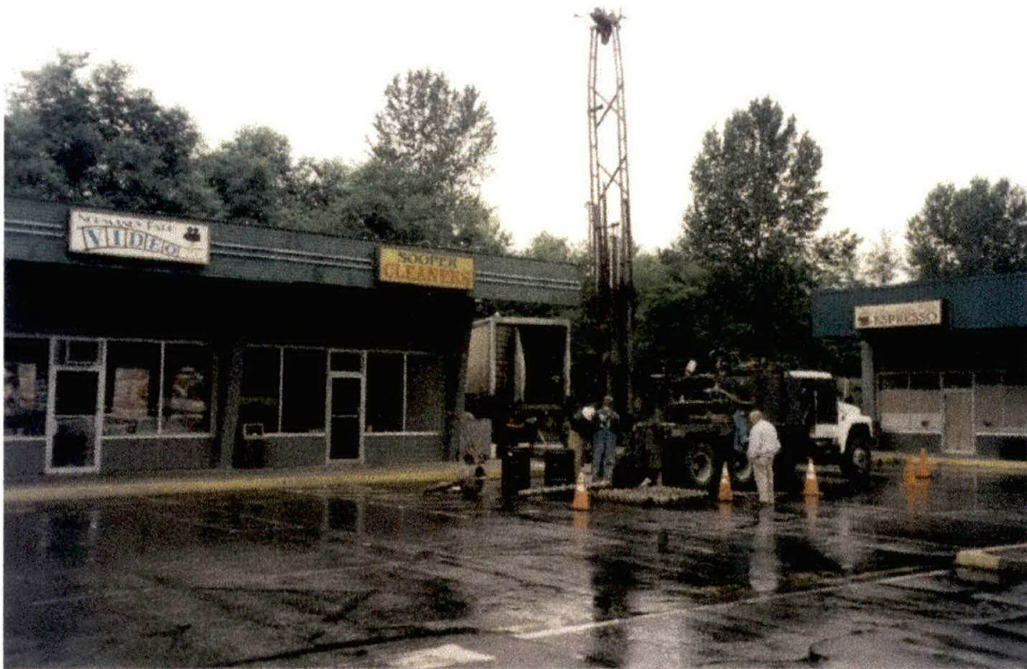
Photo 5. View towards the northwest during the installation of groundwater monitoring well MW-1 immediately upgradient of the former dry cleaner tenant space. Groundwater was encountered approximately 40 feet below ground surface.
