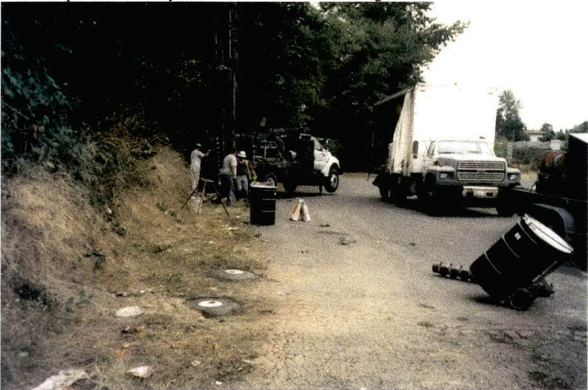
Photo 8. Installation of Stage II groundwater monitoring well MW-6 along the far western edge of the property. The surface monuments for well nest MW-5A/B are visible in the foreground.
