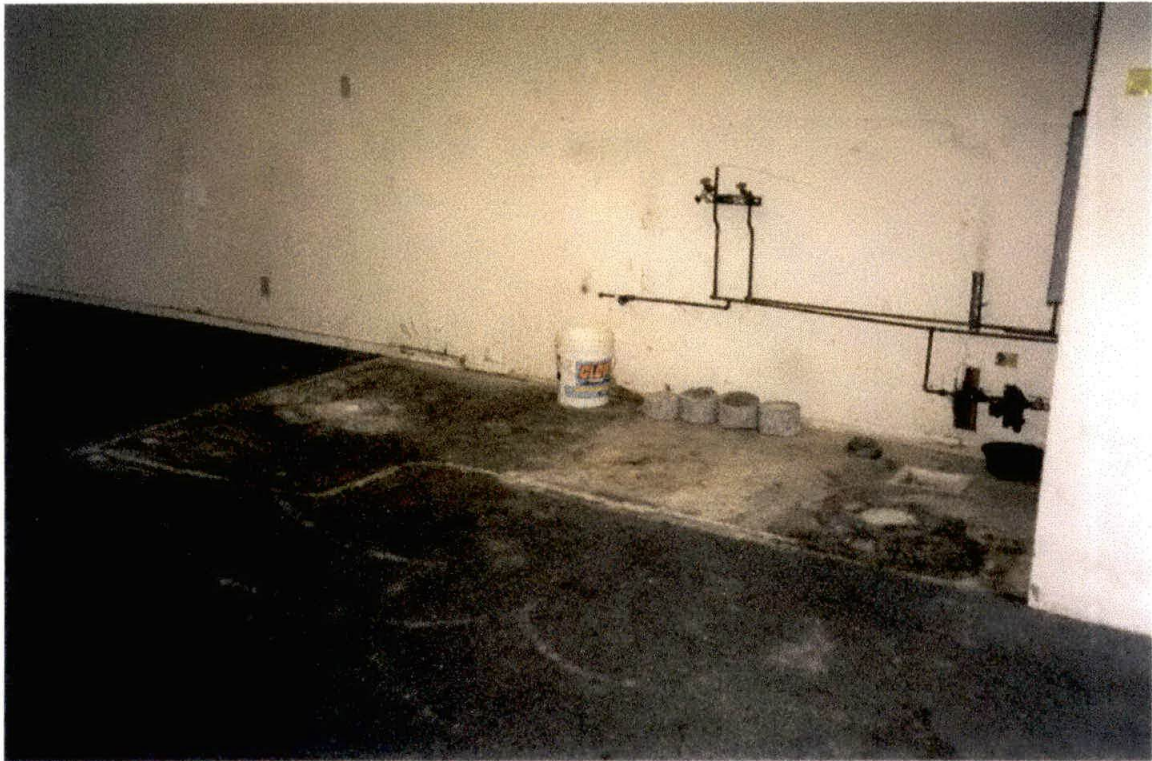
Photo 4. Close up view of the former dry cleaners floor drain and two of the indoor soil boring locations.
