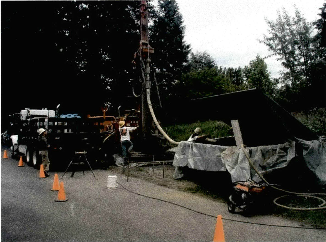
Photo 9. View to the northeast during the installation of off-site groundwater monitoring well MW-13. The well was located approximately 1,000 feet downgradient of the shopping center.
