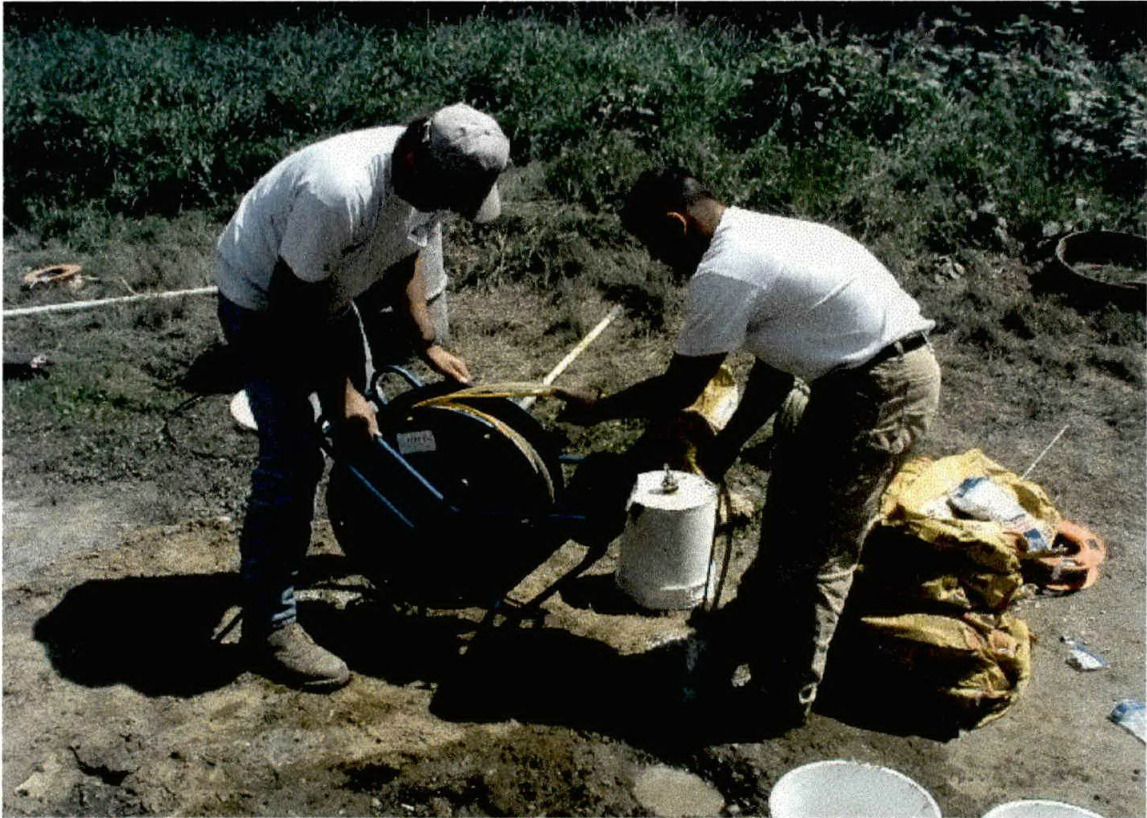
Photo 11. Completion of off site groundwater well MW-13. A stainless steel Grunfos submersible groundwater pump was used during well development to establish a good hydrologic connection to the aquifer.
