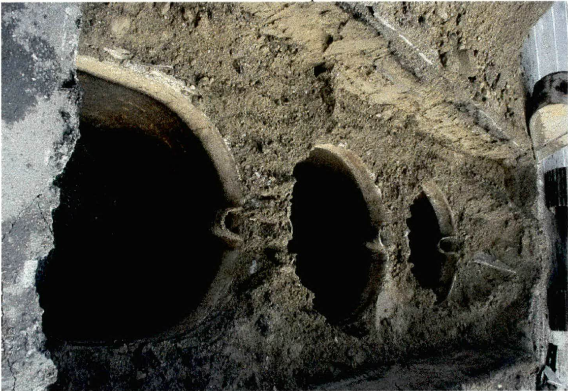
Photo 8. Exposed view of the three concrete septic tank chambers. Bottom sediment was drummed for disposal as a hazardous waste. The structures were washed, rinsed and removed from the excavation. Rinse water was carbon treated prior to METRO disposal.
