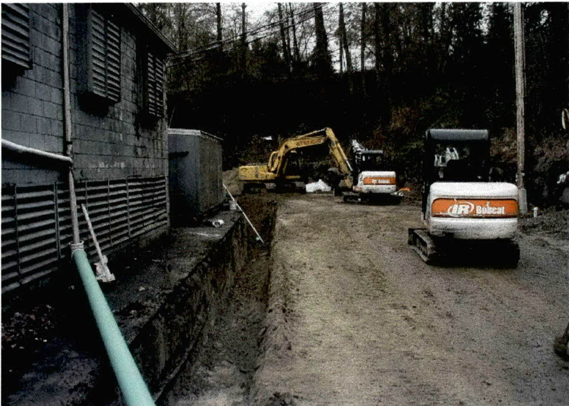
Photo 2. View towards south behind the supermarket building of the sanitary sewer trench immediately prior to installation of new PVC sewer line.
