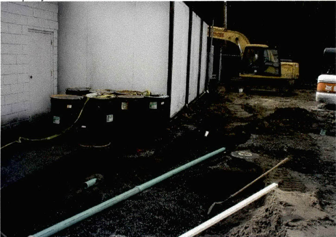
Photo 6. View towards the west showing the new sewer and roof drain lines being run around the building extension. The highest PCE soil levels encountered during the remedial activities occurred in the shallow materials excavated from along north side of the building extension.
