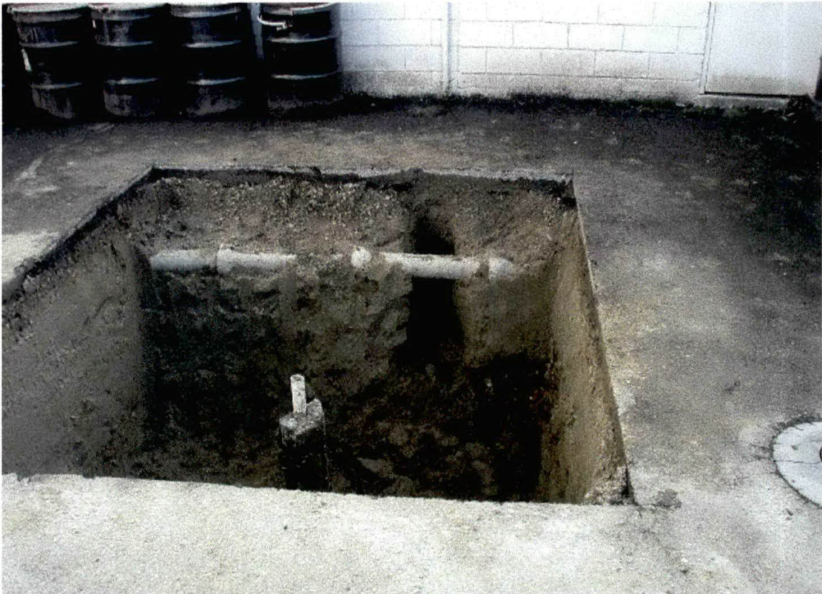
Photo 1. View looking south into initial dry well excavation. Decommissioned monitoring well MW-7 and the removed/replaced roof drain line are visible in the excavation.
