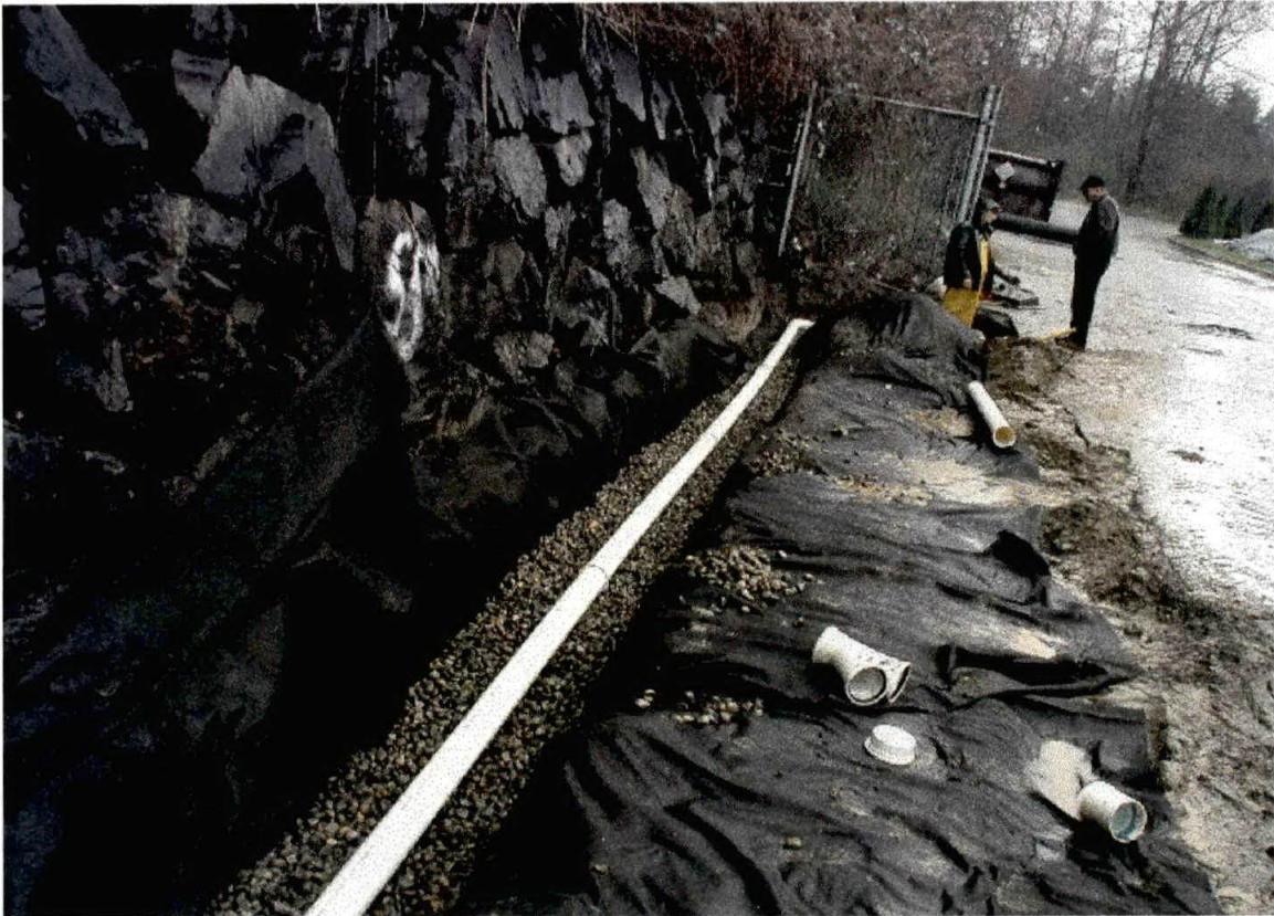
Photo 3. View looking north of the french drain installed along the western border of the property. The drain discharges into the stormwater catch basin located besides the rear gate.
