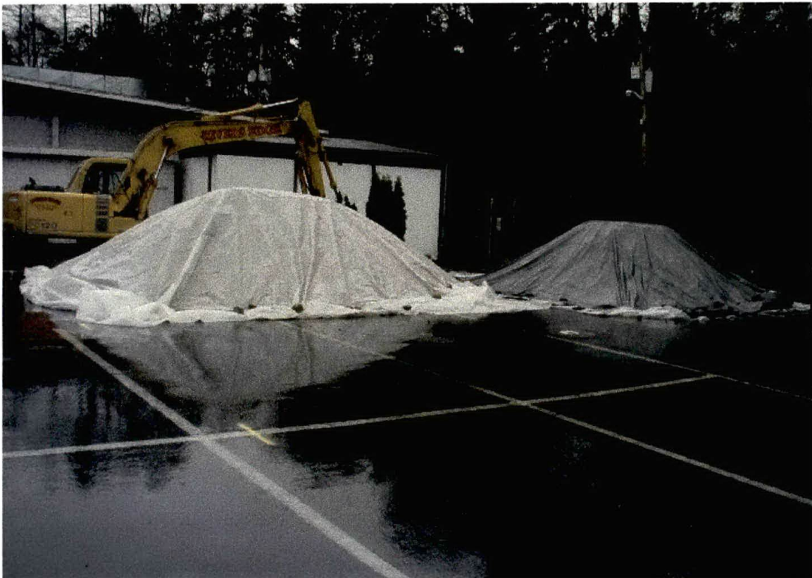
Photo 4. View of soil stockpiles. Excavated materials were stockpiled separately pending analytical testing. PCE soils were loaded into plastic lined steel containers for landfill disposal.
