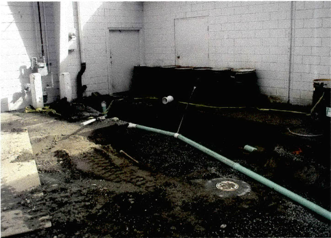
Photo 5. View towards the southeast behind the former dry cleaner. Note the new sewer line (which bypasses its former route beneath the building extension). The roof drain piping was subsequently rerouted in a similar manner.
