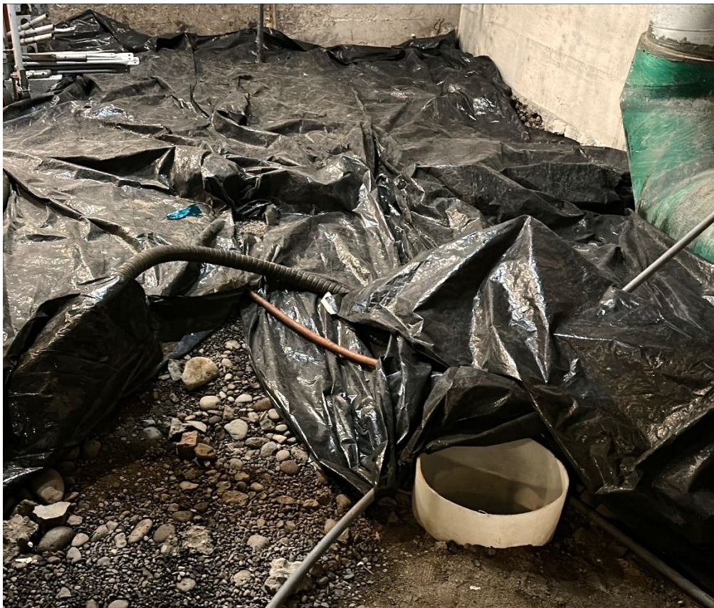
Figure 4. Aboveground Portion of Unknown Well
