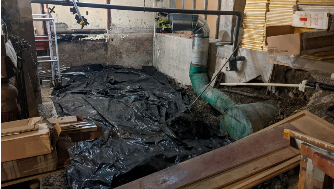
Figure 10. Unfinished Dirt Floor in Sub-Basement
