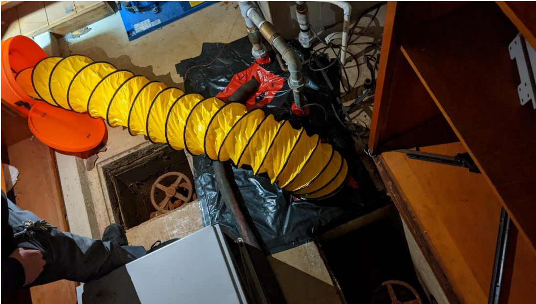
Figure 1. View of 106 Building Sump and Gate Valves (looking south)
