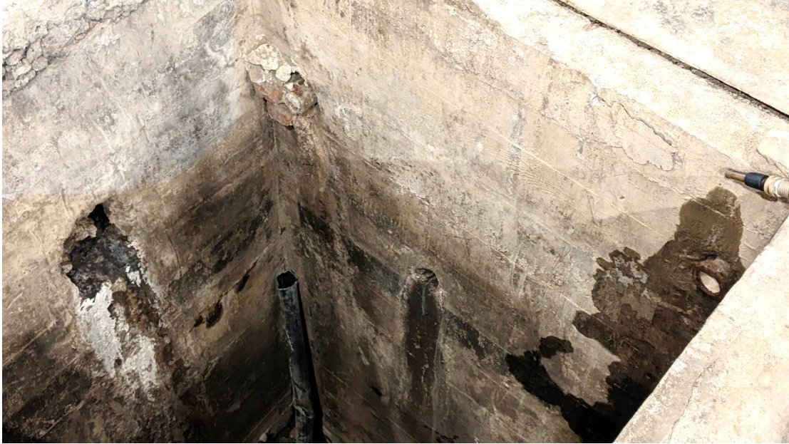
Figure 8. Interior View of Main Hotel Sump
