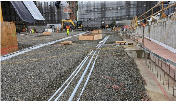
SV.02.05.A - South side of water storage tank (vapor barrier to be installed)
