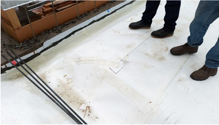
SV.02.01.E - Location marked by GCP to be fully taped by the water proofing installer
