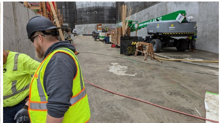
SV.02.05.B - North side of water storage tank (vapor barrier to be installed)
