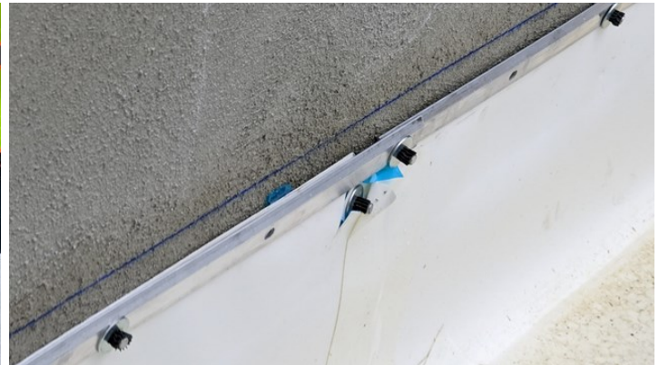
SV.02.02.B - Location where vapor barrier was torn at fastener
