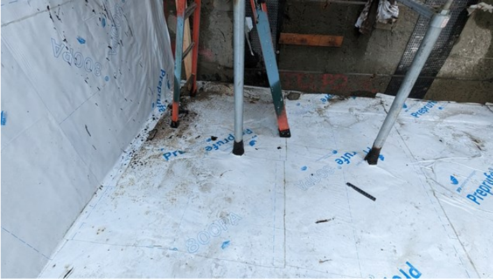
SV.04.03.E - Pipe penetration not yet detailed
