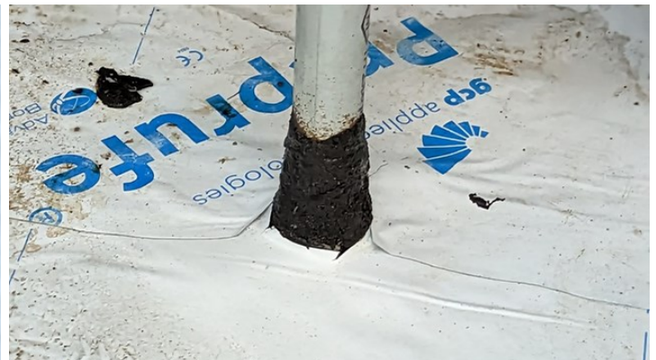
SV.04.03.D - Pipe penetration not yet detailed
