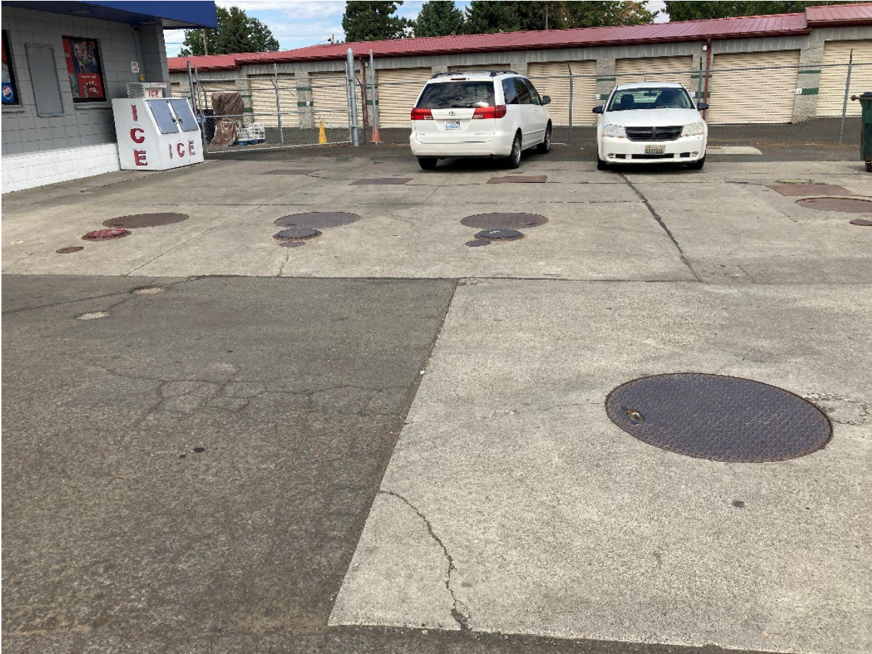
Photo 5: UST ports— from the south
