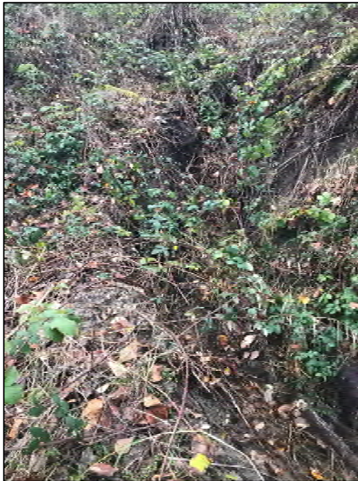
Photograph 8. Erosional feature. Surface water has been diverted to reduce further erosion. Contractor to use erosion control materials and monitor for erosion.
