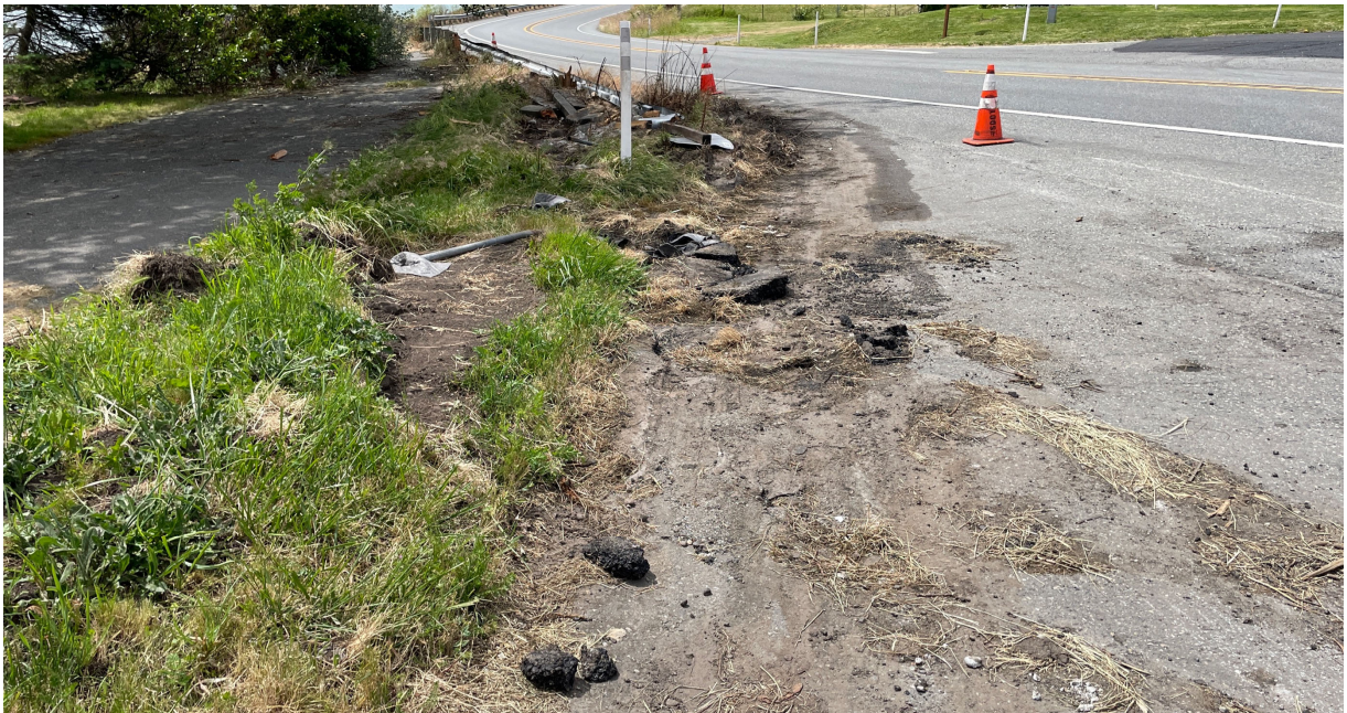
Photo 4 View of suspected contaminated soil along the shoulder of State Route 20 | Facing west | June 28, 2022
