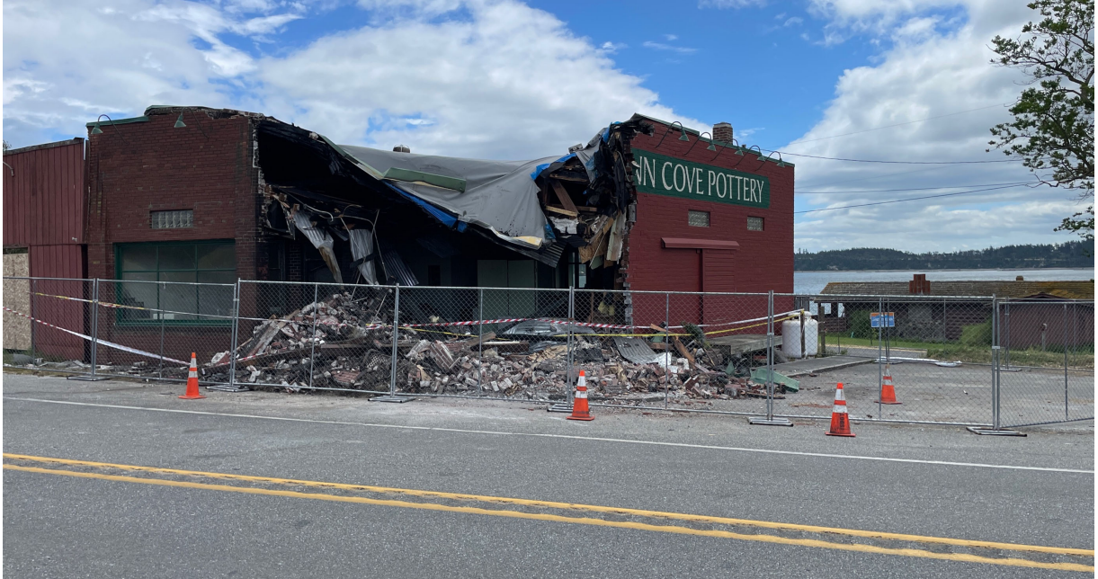
Photo 1 View of damaged building and temporary fencing | Facing south | June 28, 2022
