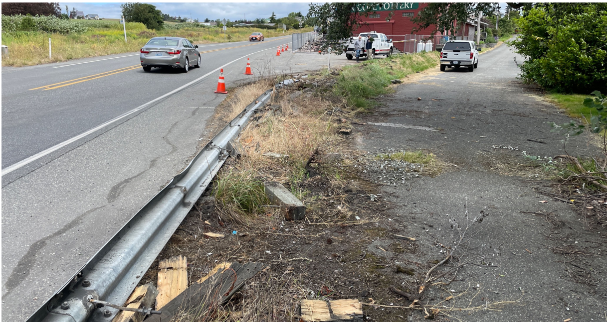
Photo 2 View of the damaged guard rail and suspected hydrocarbon impacted area on the south east edge of State Route 20. | Facing east | June 28, 2022
