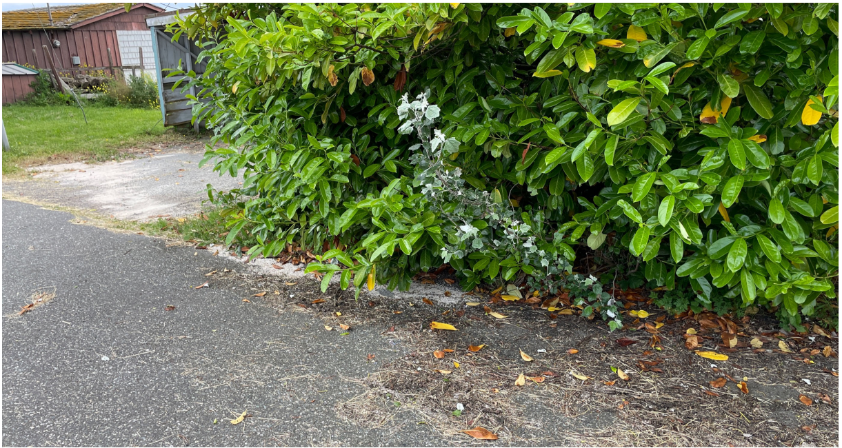
Photo 3 View of suspected hydrocarbon staining on asphalt on the south side of Penn Cove Road | Facing south | June 28, 2022
