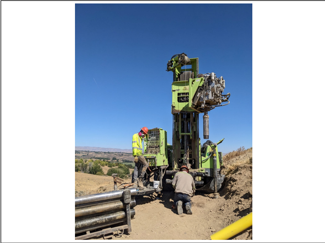
Drilling paused for repair. Example of respirator use due to gaseous odor at site T3.
