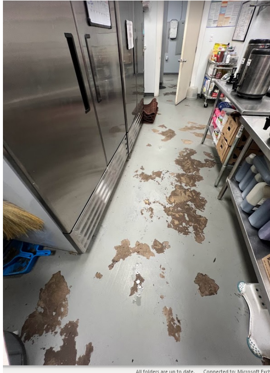
Photograph 11. Floor Slab in Kitchen of Adjacent-West Tenant Space (Suite B5) (December 8, 2023)
