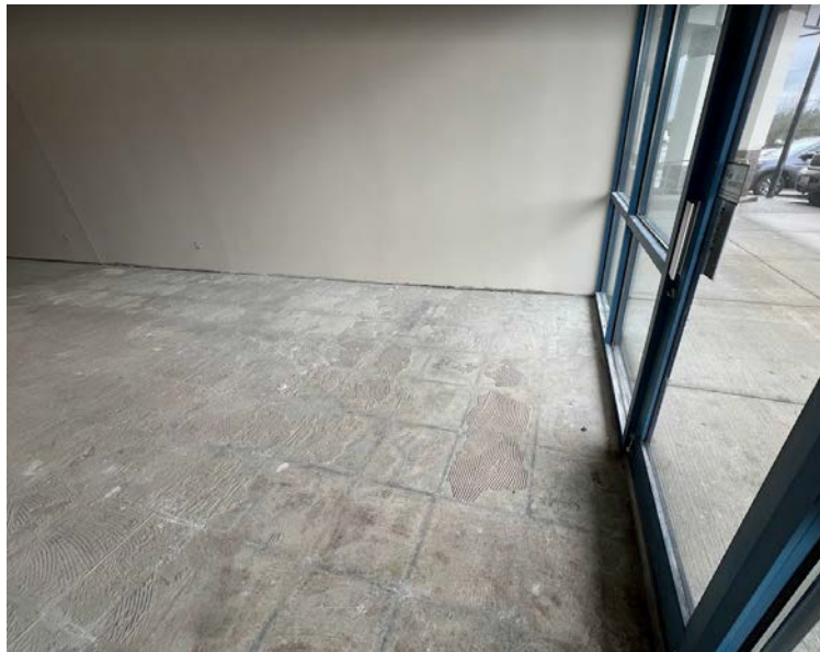
Photograph 6. Floor Slab in Front of Former Harbour Pointe Cleaners, Facing East (Suite B6) (December 8, 2023)
