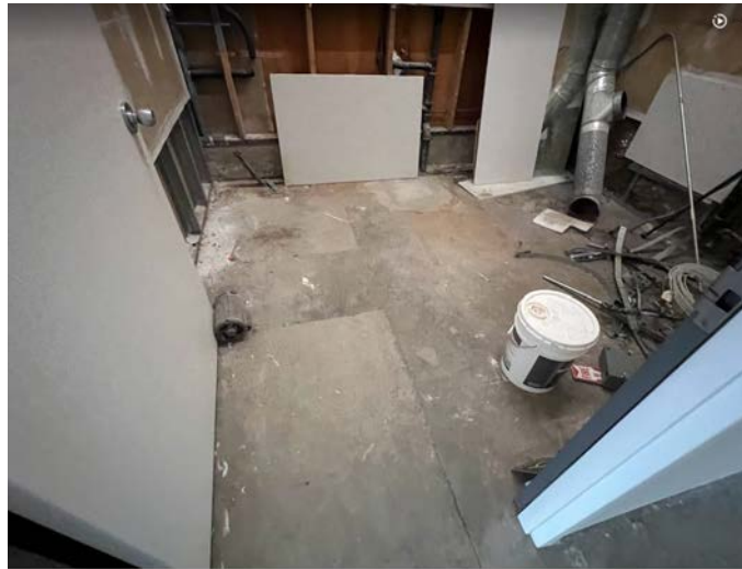
Photograph 4. Floor Slab in Rear Utility Room of Former Harbour Pointe Cleaners (Suite B6) (December 8, 2023)
