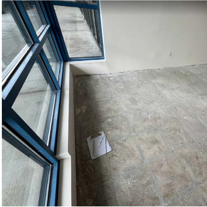
Photograph 5. Floor Slab in Front of Former Harbour Pointe Cleaners, Facing West (Suite B6) (December 8, 2023)
