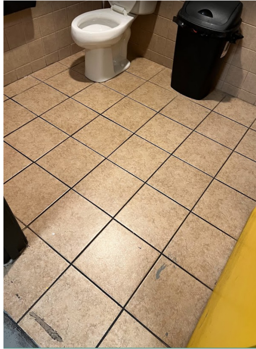
Photograph 13. Floor Slab in Bathroom 1 of Adjacent-West Tenant Space (Suite B5) (December 8, 2023)
