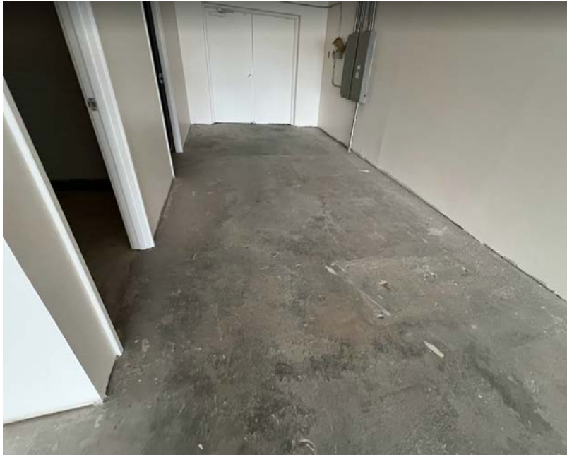
Photograph 2. Floor Slab in Rear of Former Harbour Pointe Cleaners (Suite B6) (December 8, 2023)
