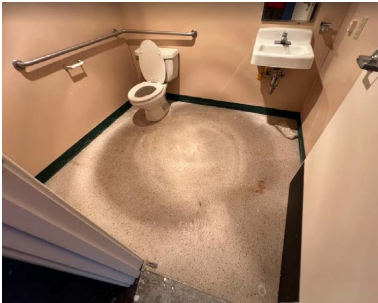
Photograph 16. Bathroom Floor in Suite B7 (December 8, 2023)
