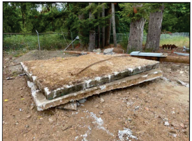
Concrete pads upon which the transformer was stationed
