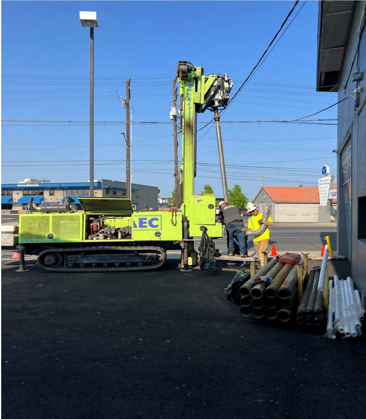
Photograph 2 – Anderson Environmental Contracting (AEC) employee carrying a soil sample bag from the drill rig to the geologist’s field table on May 19, 2023 (facing west).
