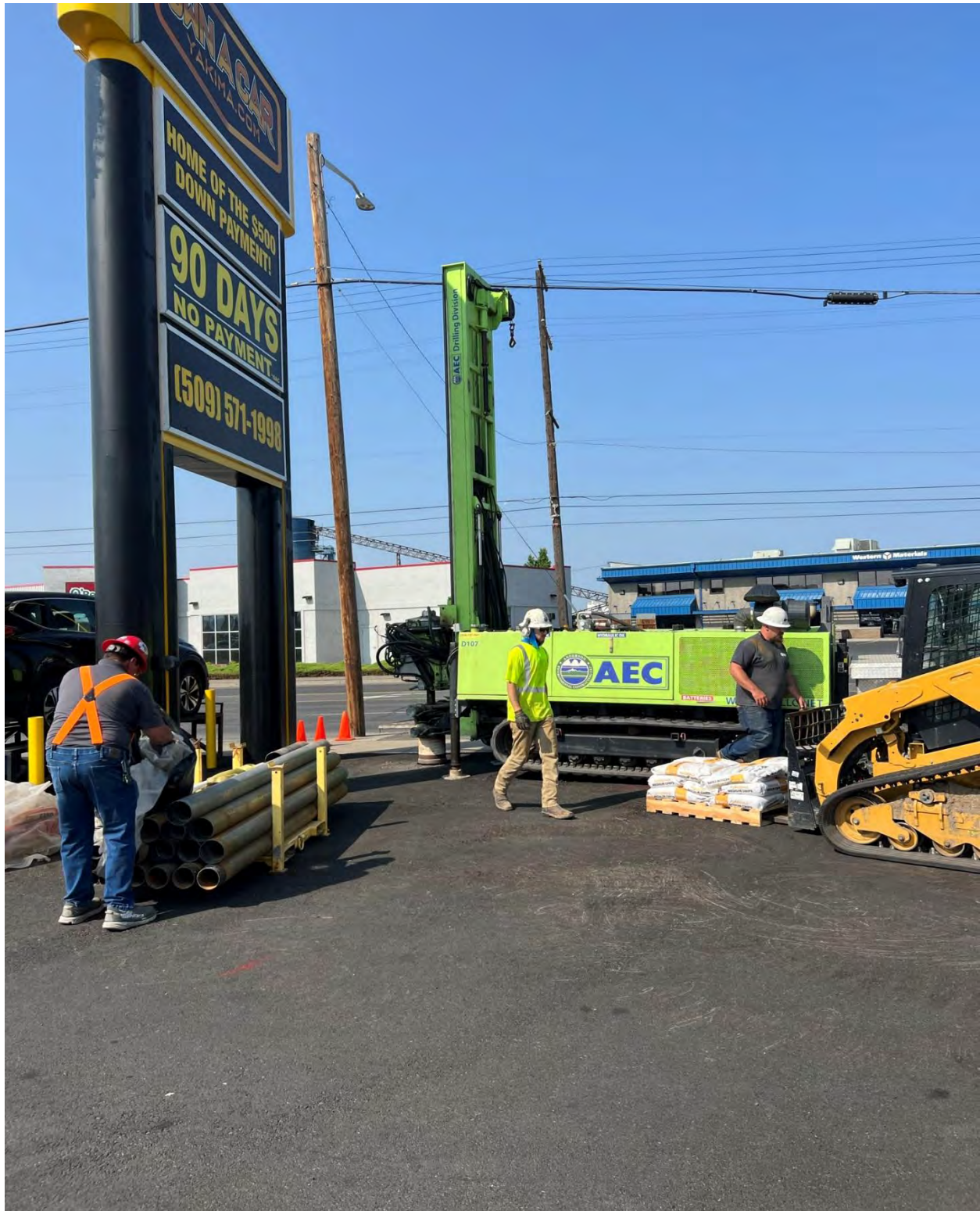
Photograph 3 – Terra sonic drilling rig set-up to advance boring MW8 on May 19, 2023 (facing west).
