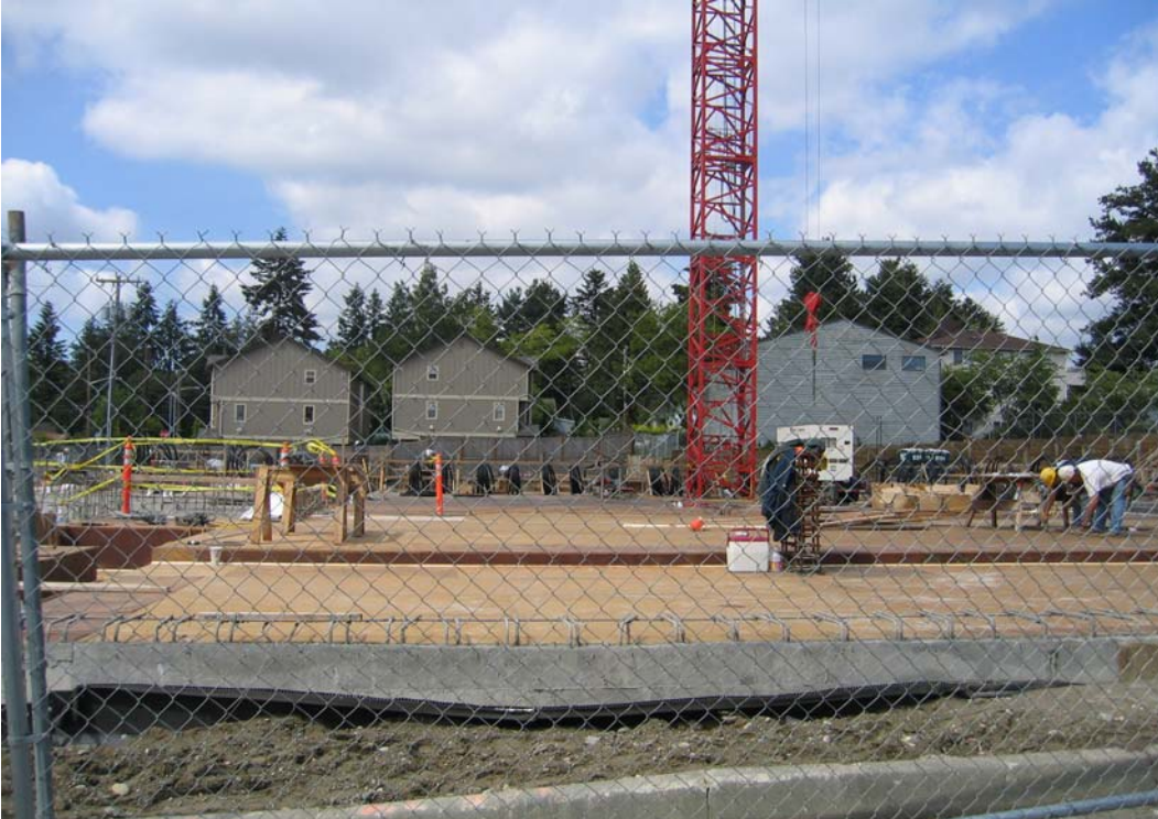
South to north view of Site (building under construction) and neighboring apartments in the background.
