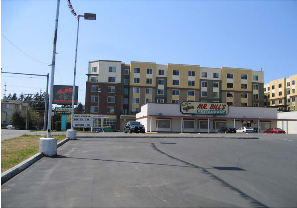
East to west view of a restaurant (foreground) and the southern portion of the Site (building under construction in background).
