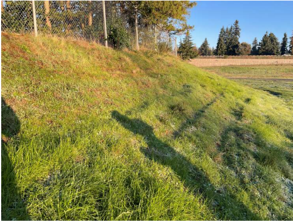
Photograph L5. Stations LLA 10 through LLA 13 during the November 16, 2023, follow-up barrier inspection. Improved conditions due to increased vegetation were noted; barrier repair is not required. See Photograph L4 for previous conditions.
