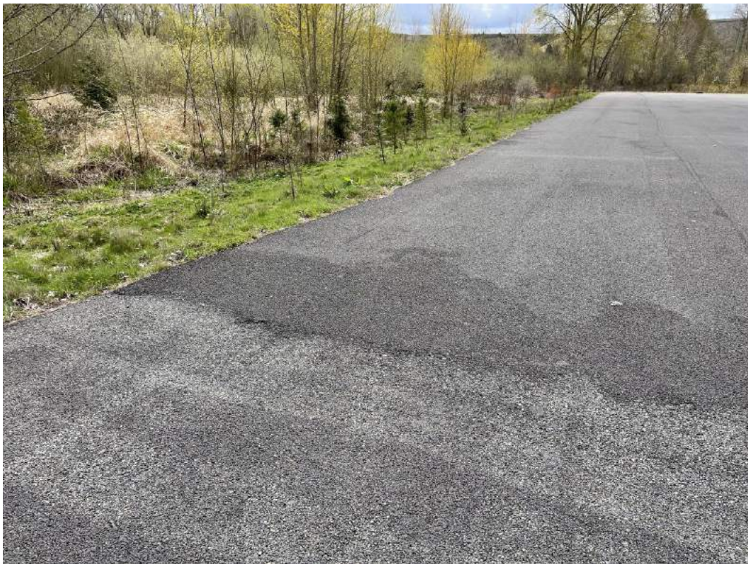
Photograph D3. East border of the DMCA near Station DMCA 05 showing potential signs of material loss, recommended for continued monitoring.
