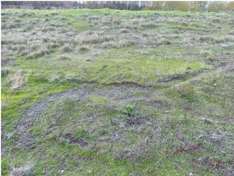
Photograph L6. Station LLA 15 showing signs of vegetation loss and exposed soil near the swale, similar to the loss noted at the slope near Stations LLA 16 and LLA 17.
