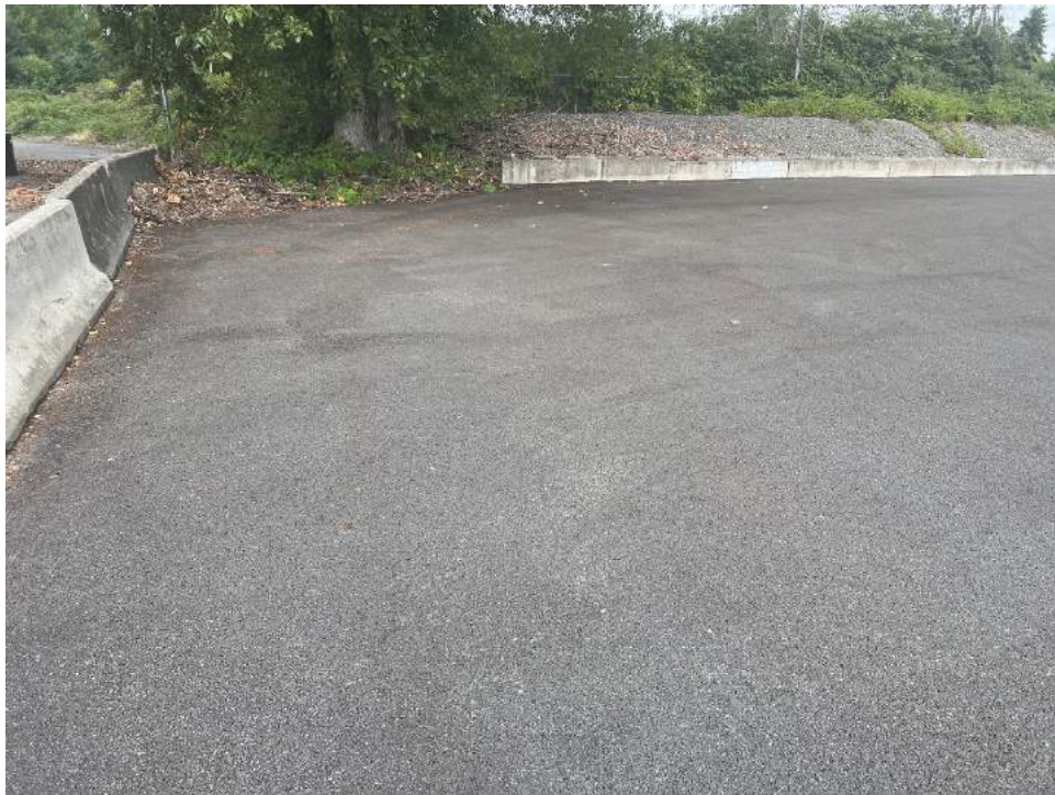
Photograph 2. The southwest corner of the 1982 Dredged Material Containment Area (DMCA) on July 12, 2023, after sweeping.
