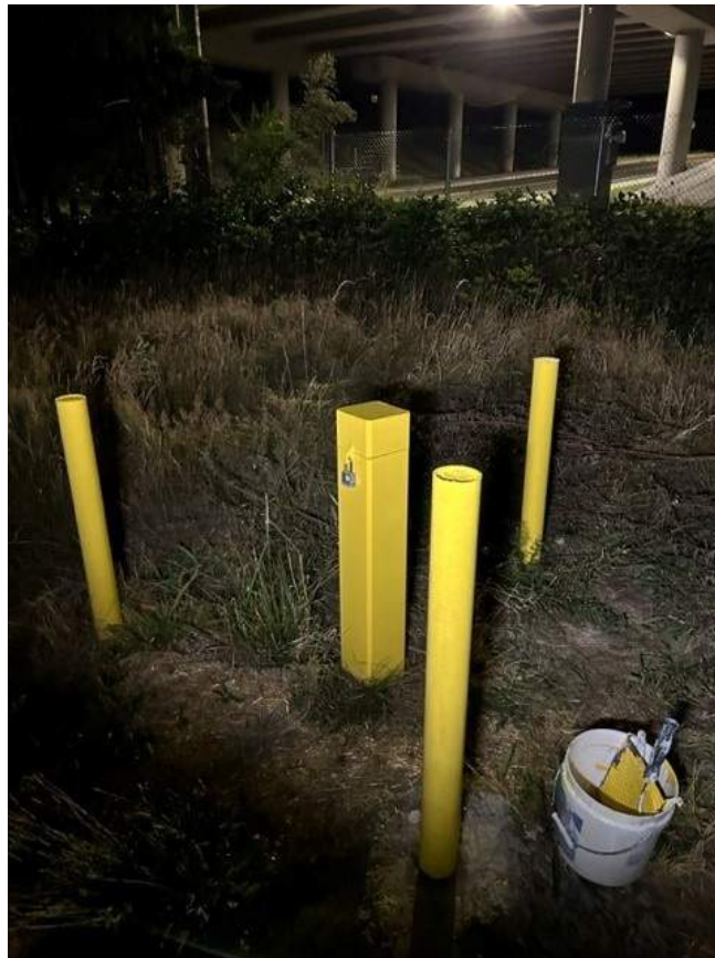
Photograph 8. Painted replacement bollard installed on July 14, 2023, near MW-C1/VB1 (northwest corner of the Lora Lake Apartments Parcel).
