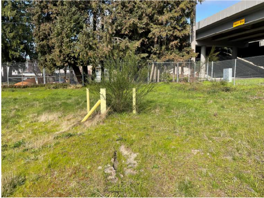
Photograph L3. Station LLA 07 showing damaged bollard near MW-C1/VB1.
