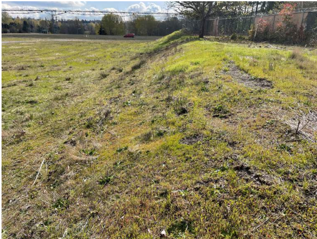
Photograph L4. Stations LLA 10 through 13 showing vegetation loss and exposed soil.
