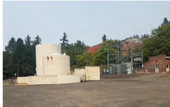
ASTs and electrical substation
