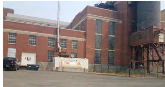
Backup generator and AST
