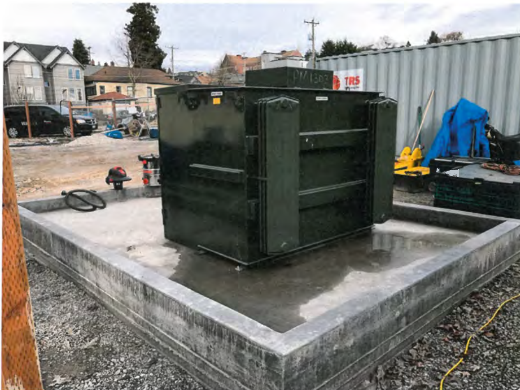
Example of transformer with secondary containment from a similar thermal remediation project.
