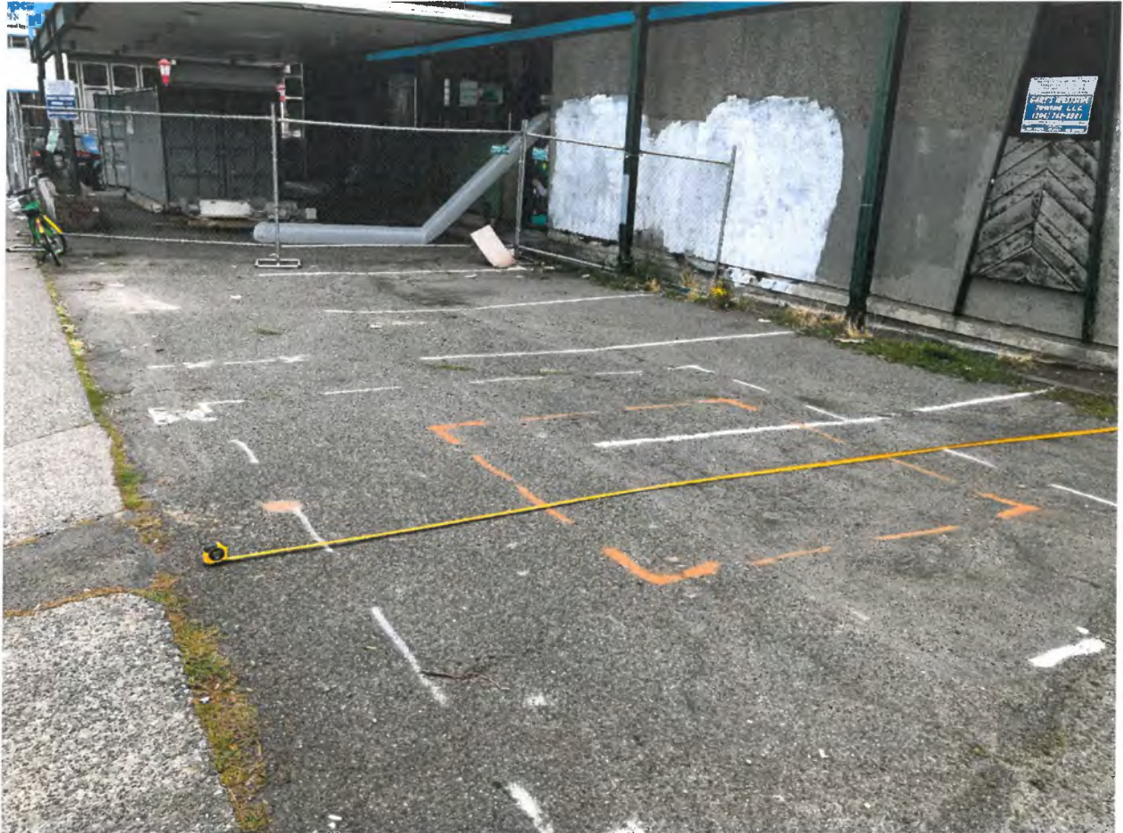
View of proposed transformer location from the sidewalk along S Dearborn St. Location of transformer containment pad is marked in white paint. Fence with mural will end where white X's are marked.
