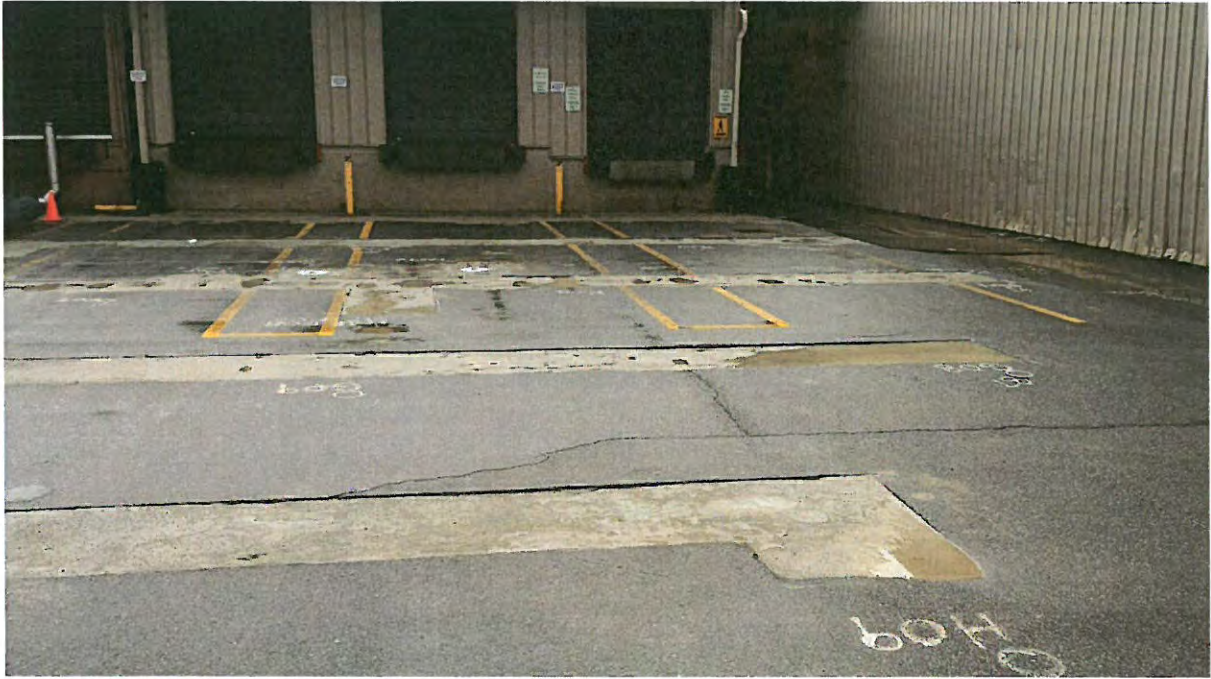
Trench in parking lot repaired with controlled density fill (CDF) during ERH operations. The CDF is removed and replaced with asphalt at the completion of operations.
