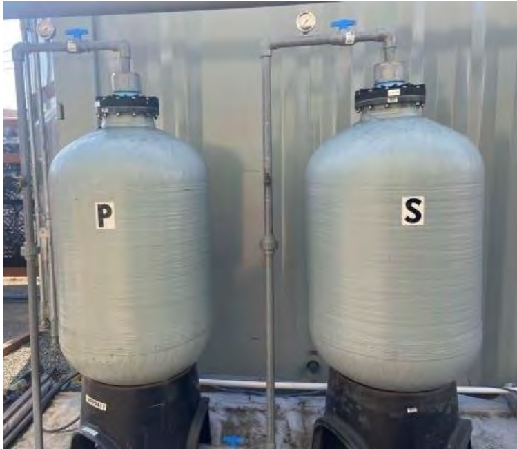
Photograph 3. Liquid GAC Vessels (July 2021)
