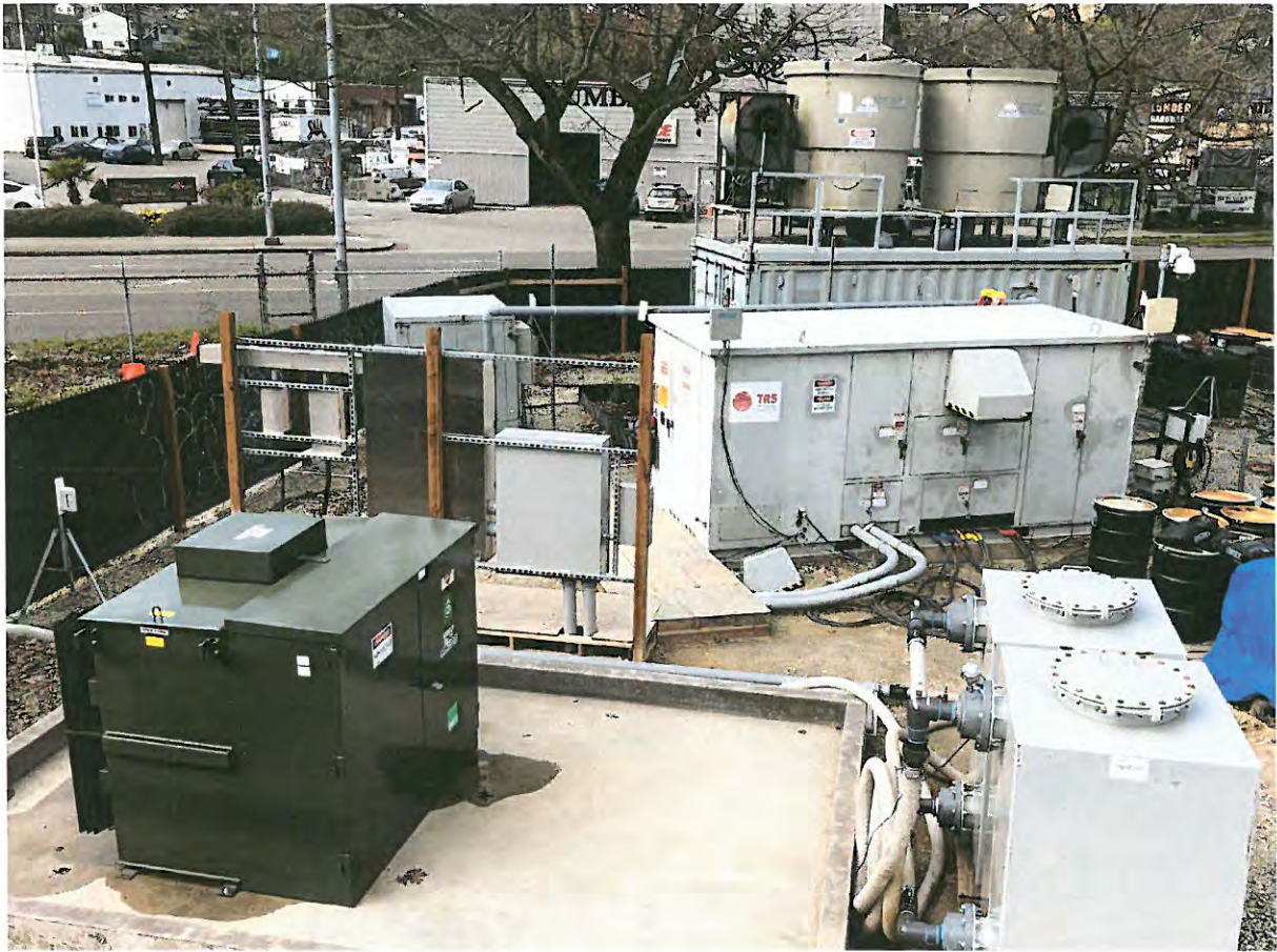
Typical ERH equipment compound. The equipment located in the center background are the condenser/cooling towers. The unit is 20' long by 8' wide by approximately 16' high. The equipment located in the center is the ERH power control unit (PCU). The PCU for this site will be 15' long by 8' wide by 9' high.
