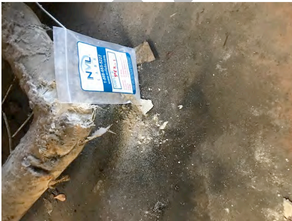
Photograph 2 – Pipe Elbow (PE3-1), Maintenance Building
