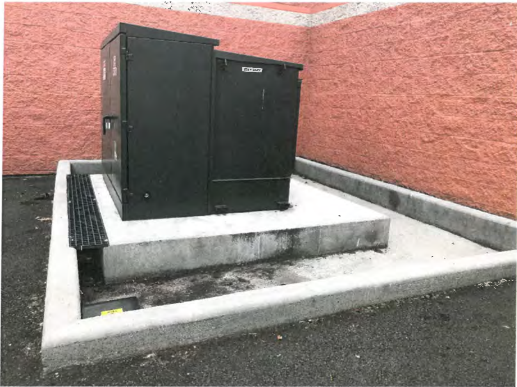
Example of similar transformer with secondary containment, provided by Seattle City Light.
