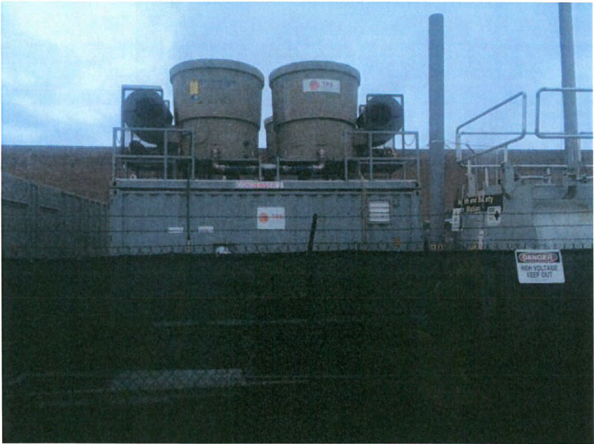
ERH equipment compound with privacy screening on security fence. The stack in the center of the photo is similar in height to what will be at the site.
