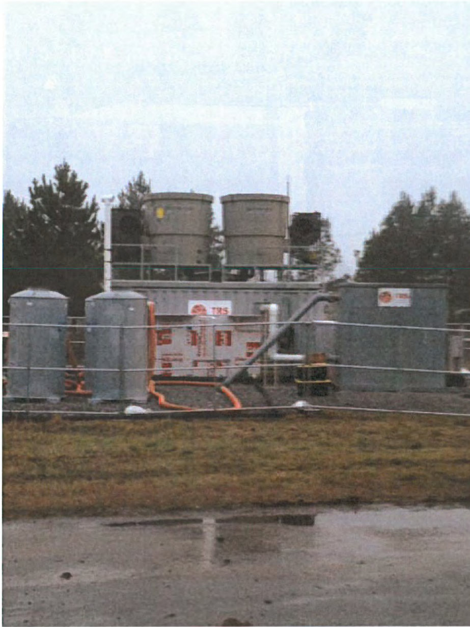
ERH equipment compound without privacy screening on fence. Vapor phase granular activated carbon vessels and discharge stack are located in the foreground.
