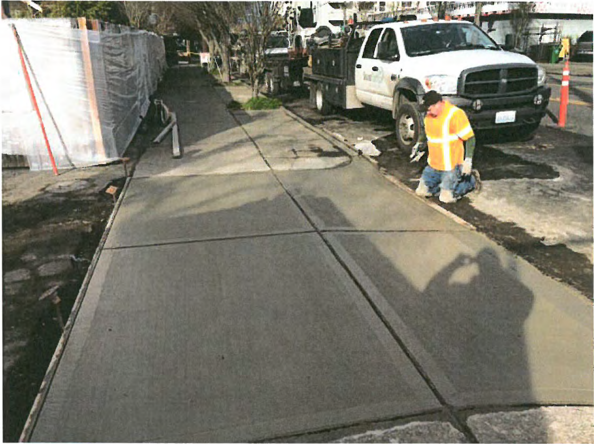
Newly installed driveway at the completion of ERH operations in the Green Lake area of Seattle. Plastic was used to cover fence in order to protect from graffiti. If fencing was tagged, plastic would be replaced.
