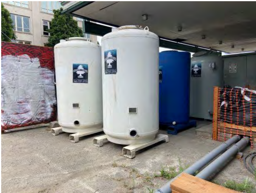
Photograph 4. Vapor GAC Vessels (July 2021)
