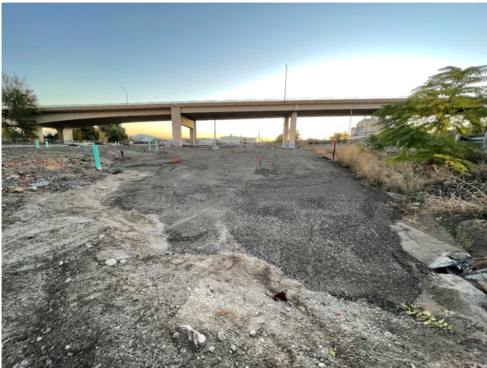
Photograph 4. View of proposed Building 2B footprint with building footprint excavation backfilled and stormwater cover placed and compacted. Looking east.
