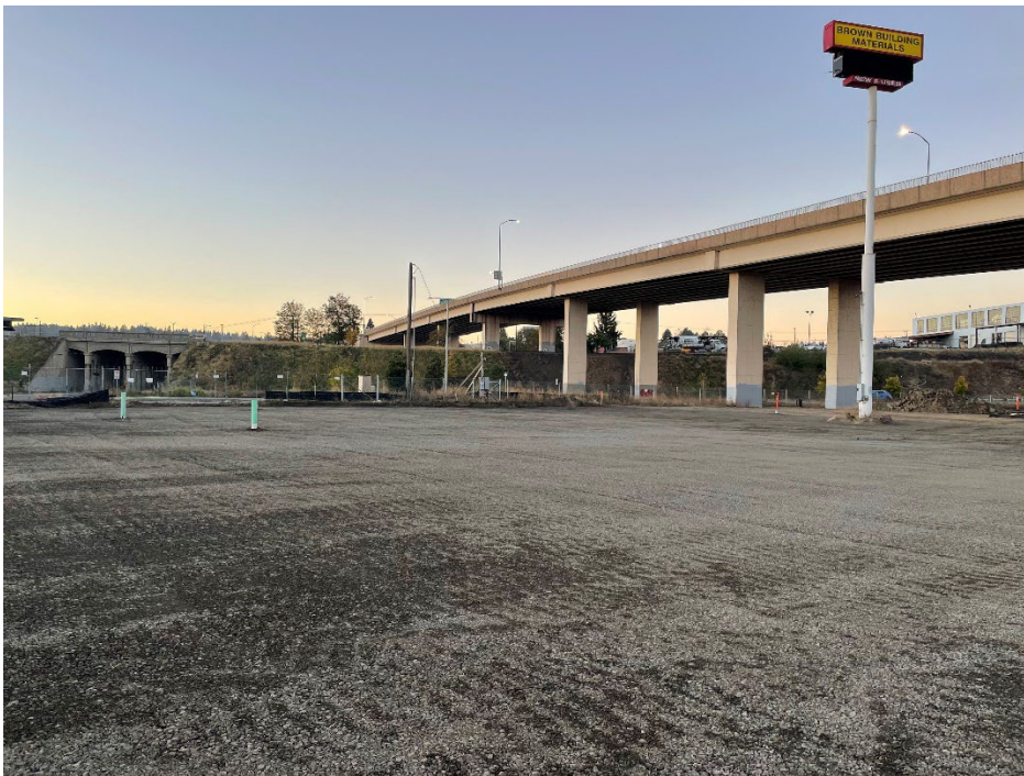
Photograph 2. View of proposed Building 2A footprint with building footprint excavation backfilled and stormwater cover placed and compacted. Looking southwest.
