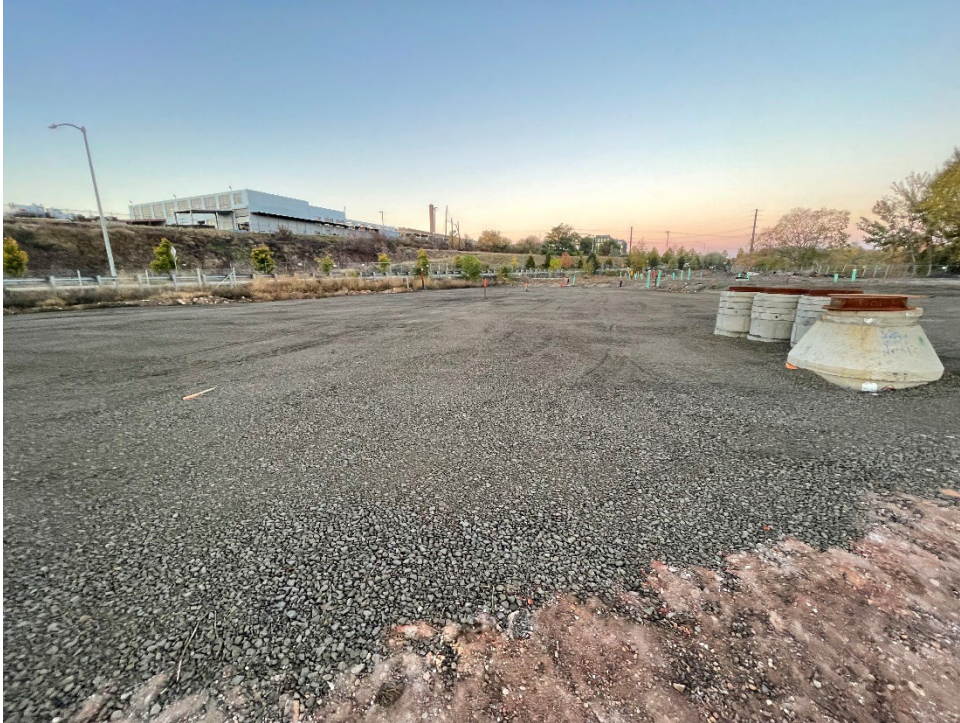
Photograph 3. View of proposed Building 2B footprint with building footprint excavation backfilled and stormwater cover placed and compacted. Looking west.
