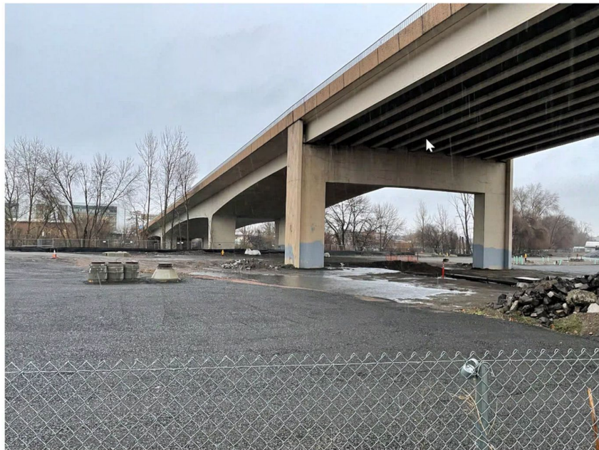
Figure 1. North, Northeastward view of Hamilton Street Bridge and water that has drained from the bridge deck onto Sagamore property.
