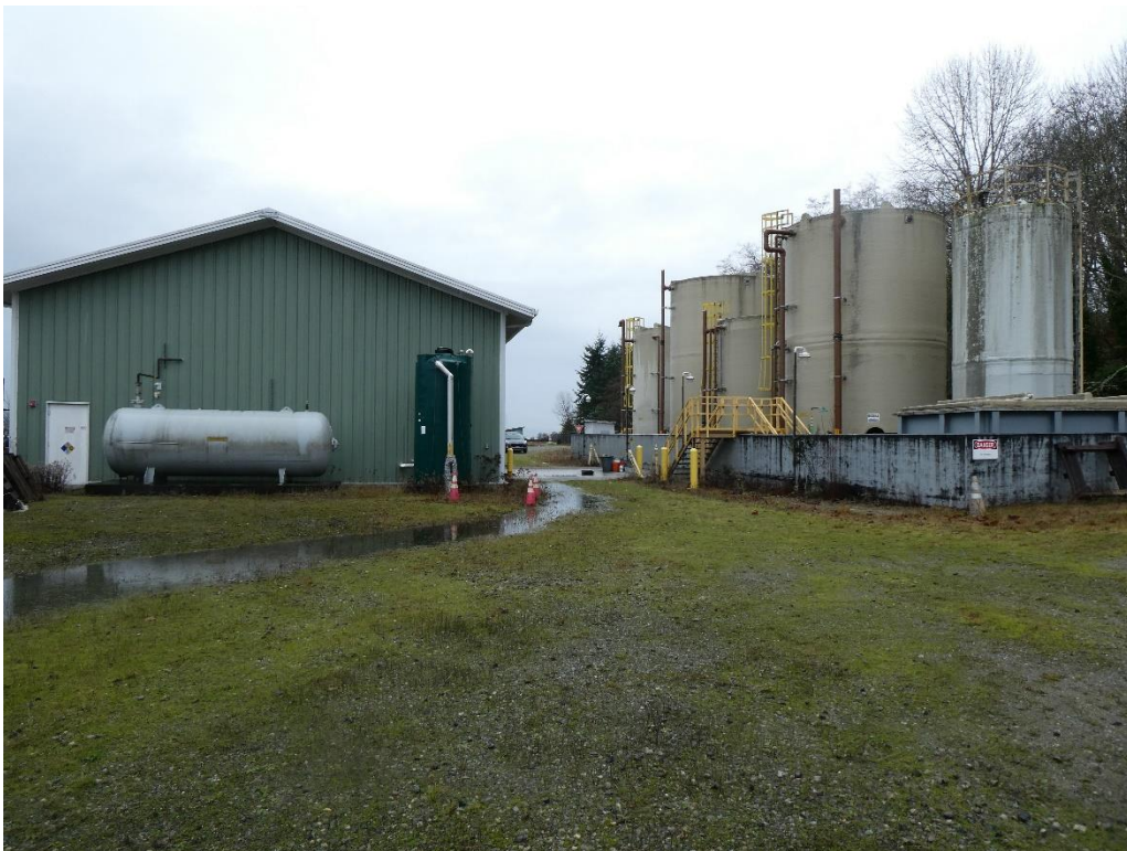
Groundwater treatment plant building and tank farm
