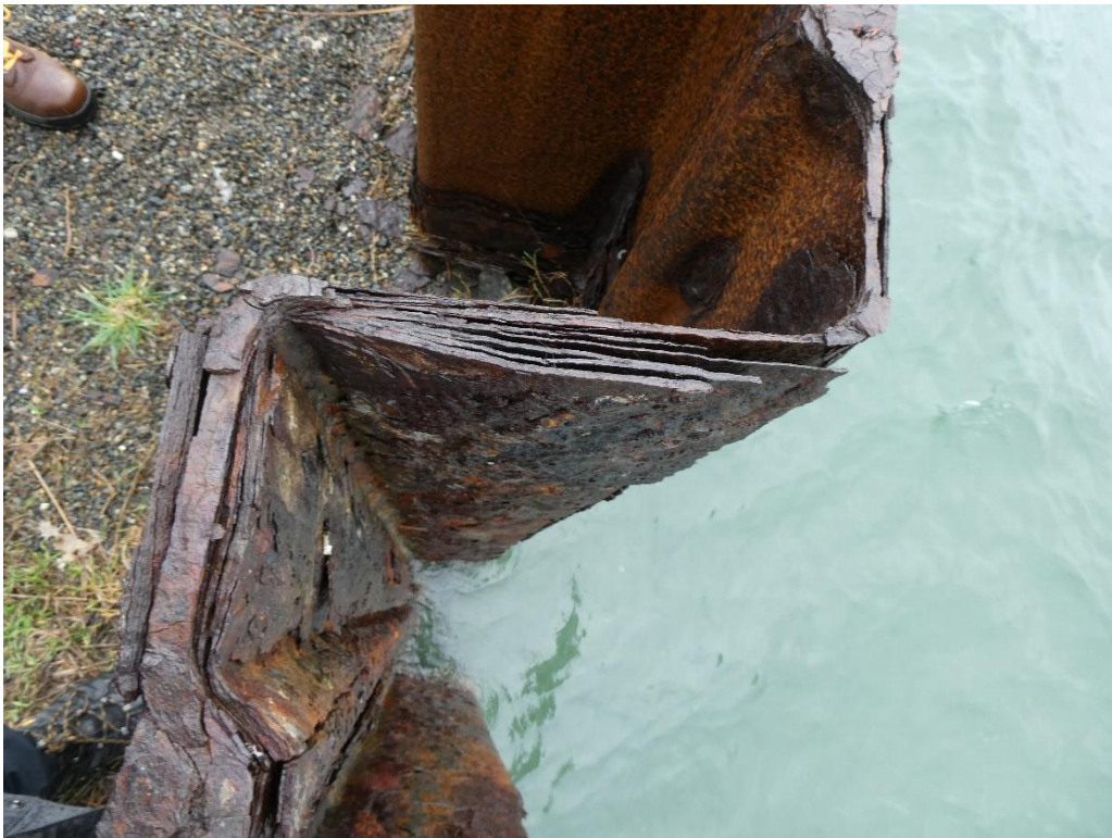
Degraded eastern sheet pile wall
