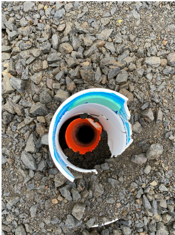
1. View of test pile within the cPAH impacted soil footprint on the former SGP property.
