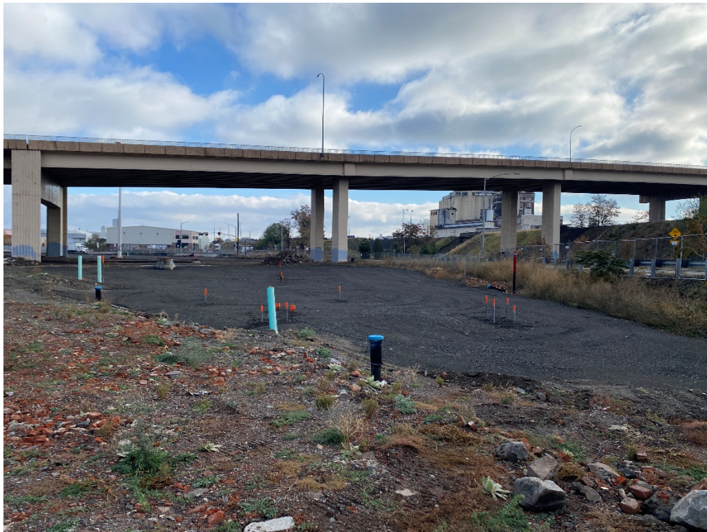
2. View of recently re-graded area in the footprint of Building 2B on former SGP property (looking east).
