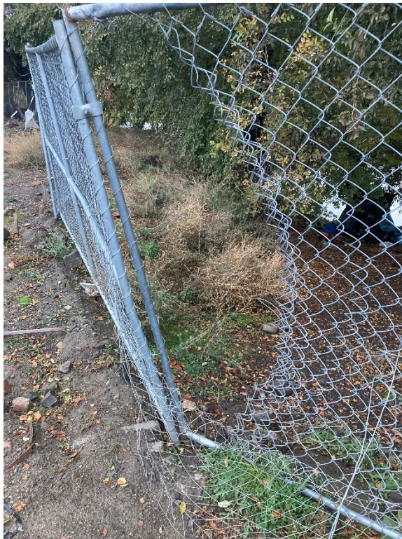
2. View of hole in fencing, leading to transient camp on shoreline, to the southwest of the north detention basin on former SGP property (looking west).
