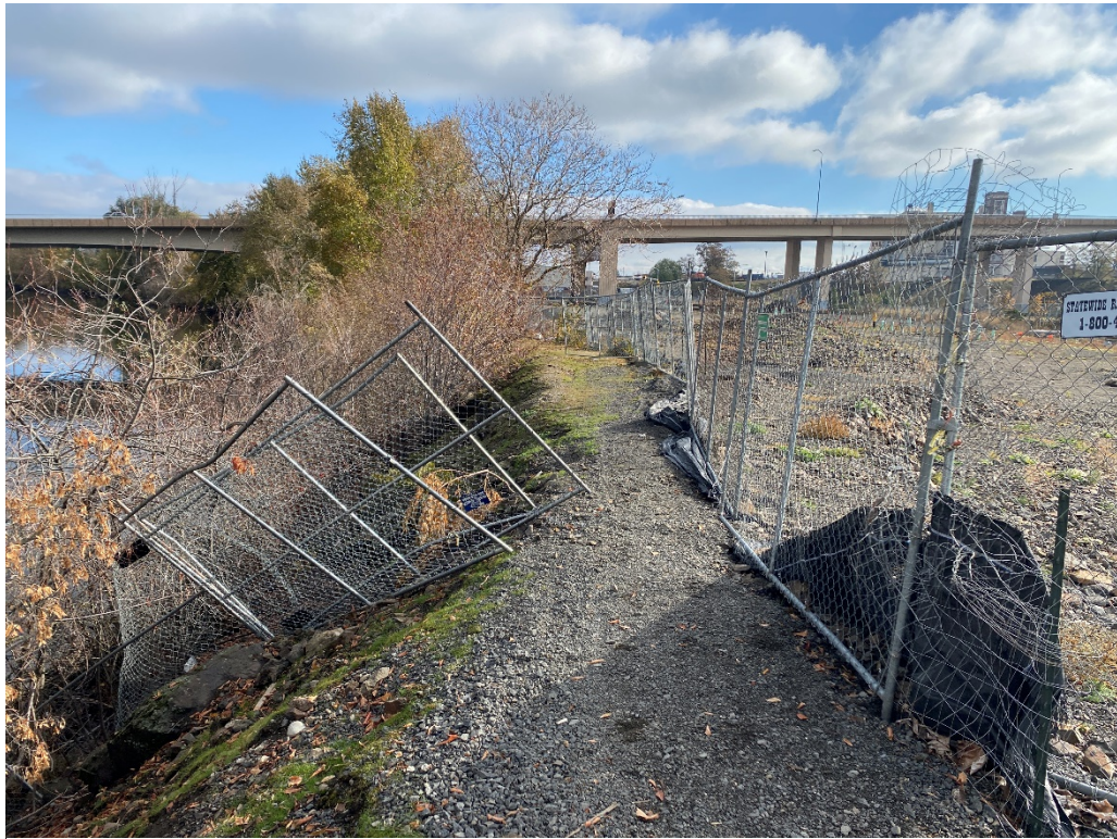
1. View of compromised perimeter fencing at the western boundary of the former SGP property (looking east).
