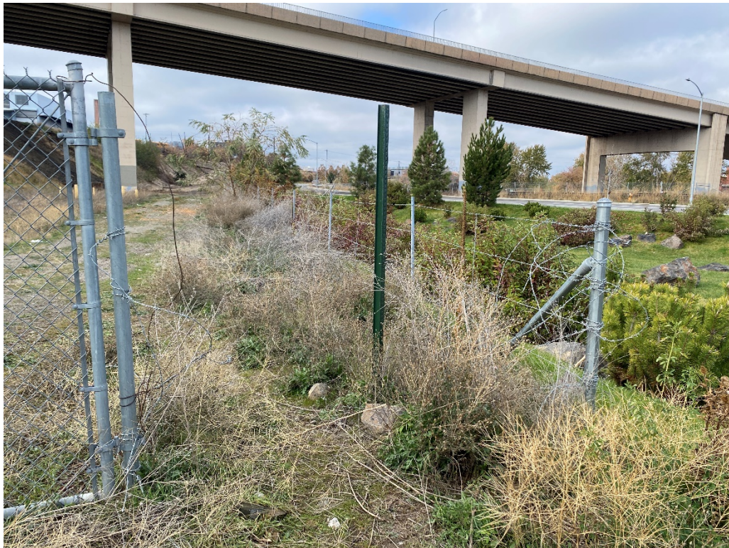
2. View of damaged perimeter fencing paralleling North Erie Street near ATC07-20 on the former ATC property (looking west).
