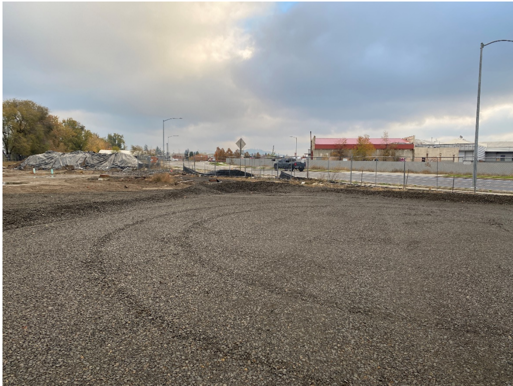
1. View of the east end of the recently re-graded area in the footprint of Building 2A sloped to sumped basin in center of photo on former SGP property (looking east).
