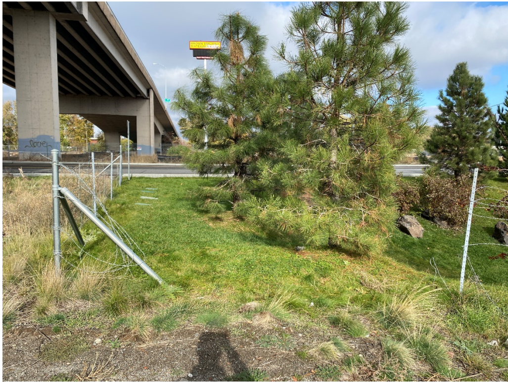
1. View of damaged perimeter fencing at the southwest corner of the lined evaporation pond on the former ATC property (looking north).
