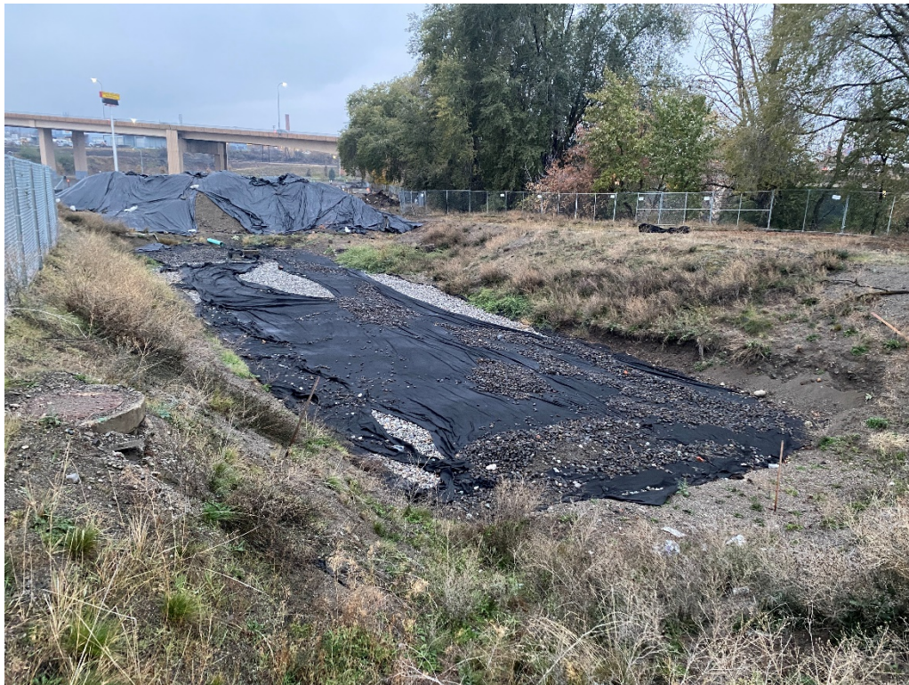
2. View of north detention basin and stockpile to the southwest of the north detention basin on former SGP property (looking west).
