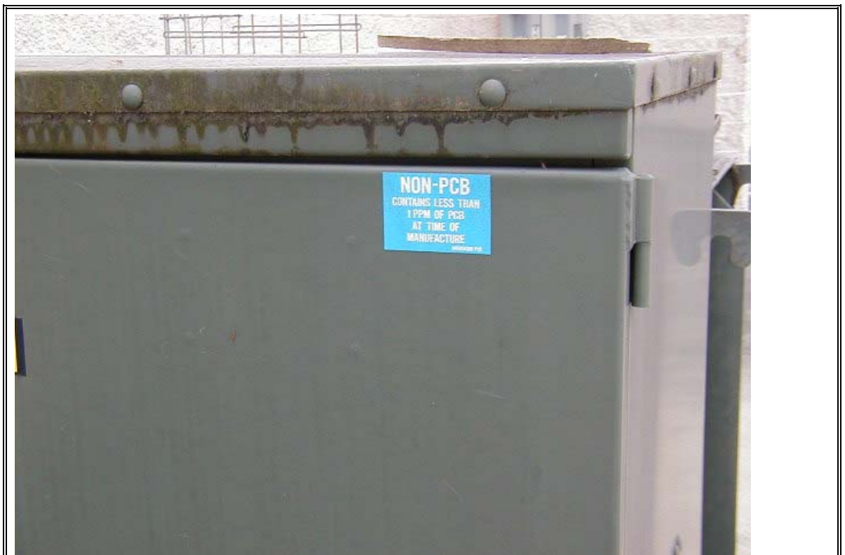
Photograph Number 2: Pad-mounted transformer labeled as non-PCB
