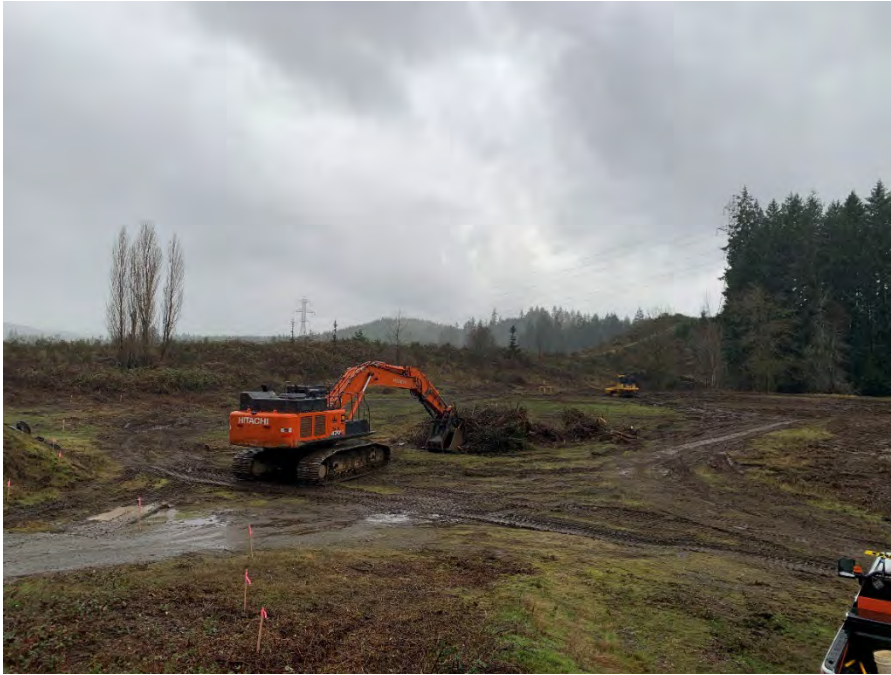
Photograph 1. View of the Property landfill area prior to the start of cleanup construction, during vegetation grubbing. Photo faces south-southwest.
