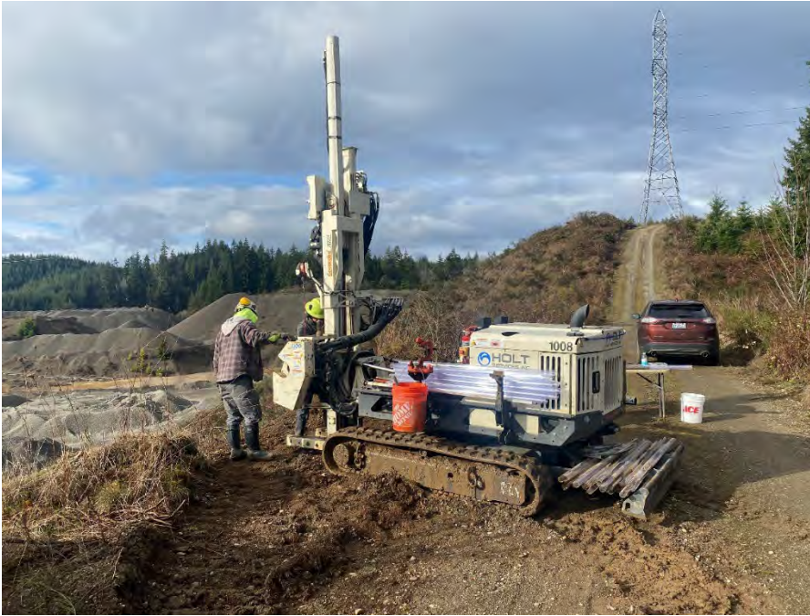
Photograph 3. Exploratory drilling on the south-adjointing property to delineate the extent of landfill waste beyond the south Property boundary. Photo faces west.
