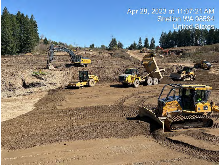
Photograph 5. Backfill and compaction of landfill waste relocation excavation on south-adjacent property. Photo faces north.
