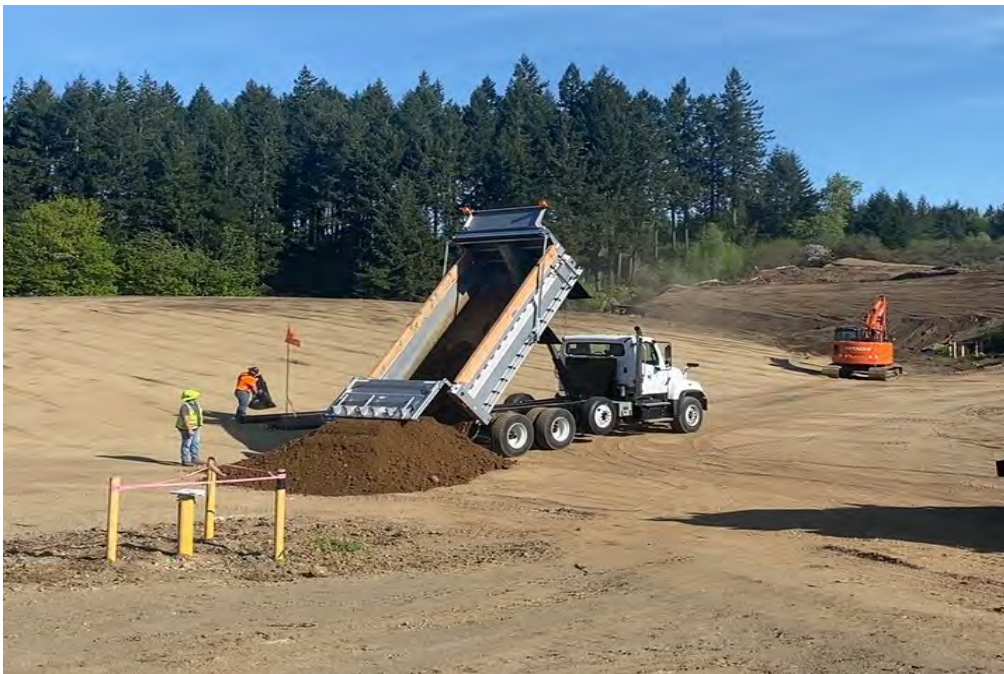
Photograph 6. Construction of foundation layer on Property. Wells AMW-02 and AMW-03 are shown. Photo faces west-northwest.
