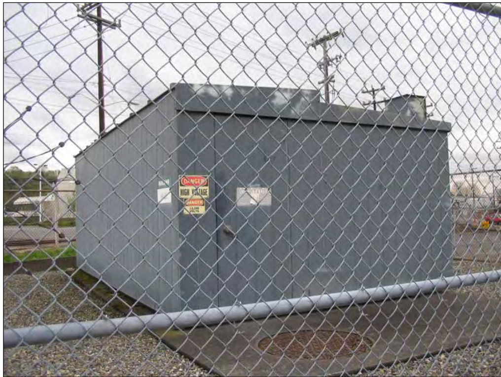
12. An electrical substation located in the southeastern portion of the subject property.
