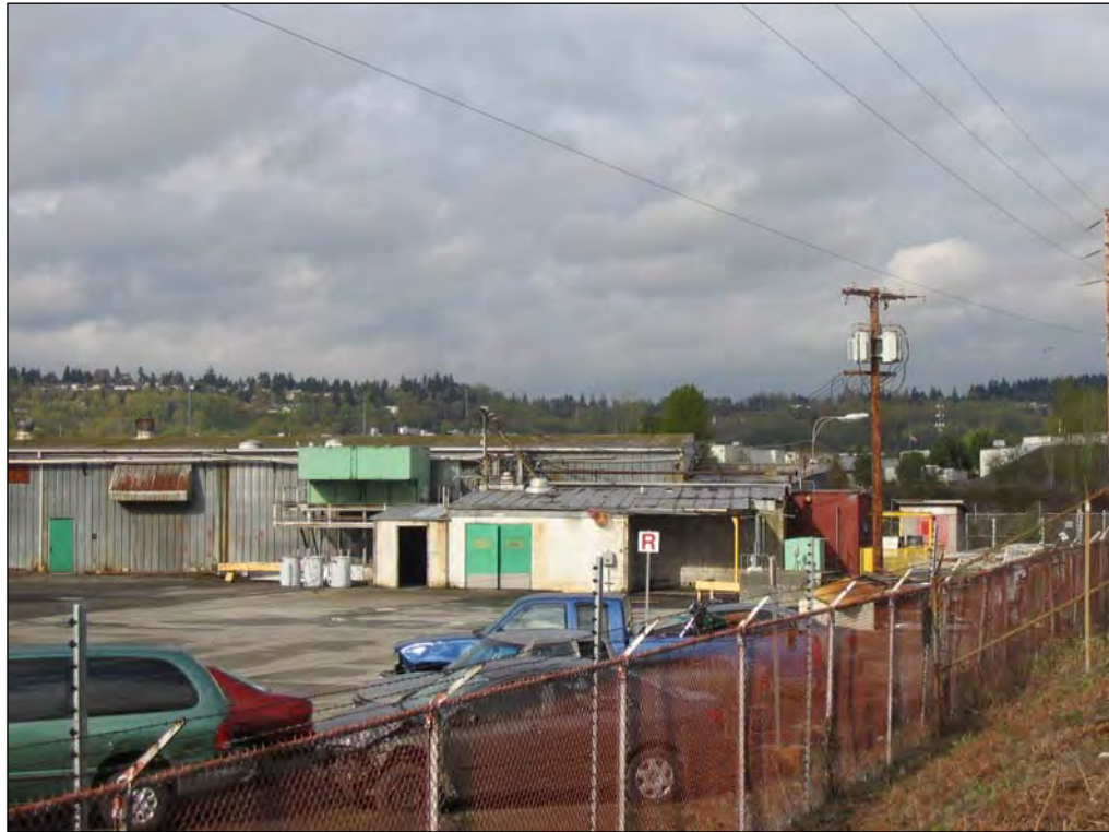
11. Electrical transformers on the adjacent property to the south.
