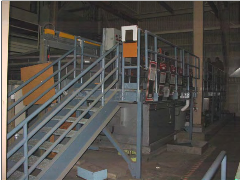
1. Aqueous degreaser located in the southwestern portion of Building 14-01.
