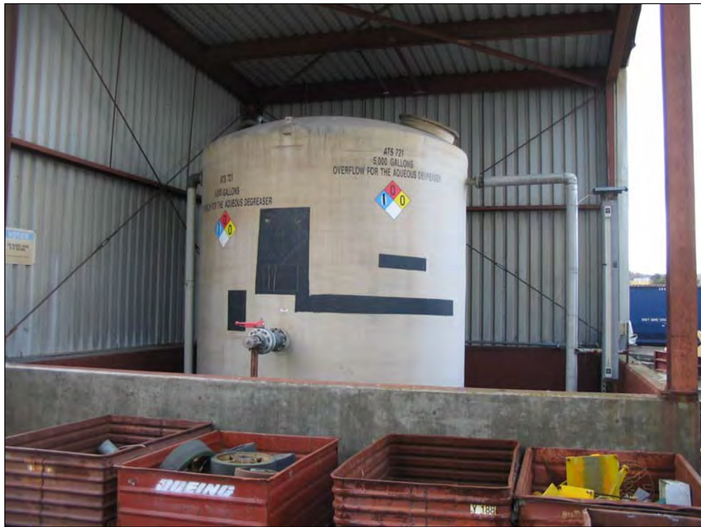
2. 5,000-gal wastewater tank located in the western yard of Building 14-01.
