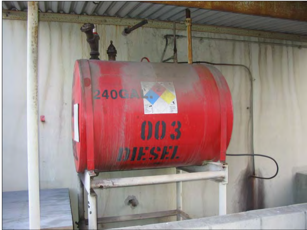
3. Diesel tank located on the northern side of Building 14-13.
