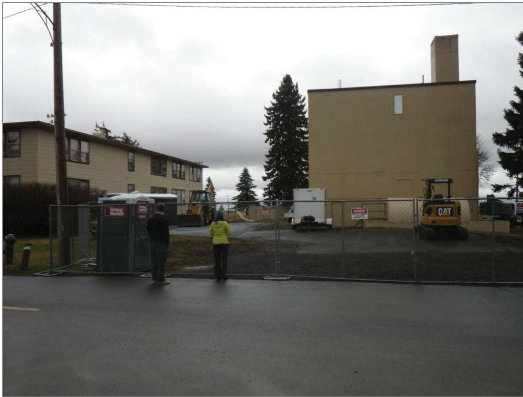
Photo 11. Site PS-7 (ST010) – Fuel Oil Storage Tanks, looking east
