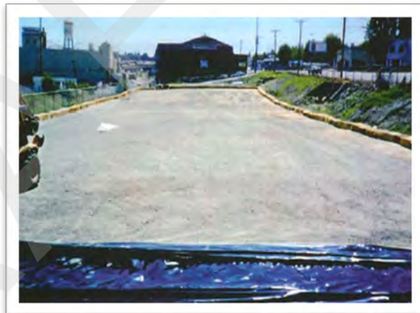
Photo 16-4. Circa 1997 photo of the southern portion of Jet Parking used as a treatment cell for petroleum-contaminated soil (looking north).
