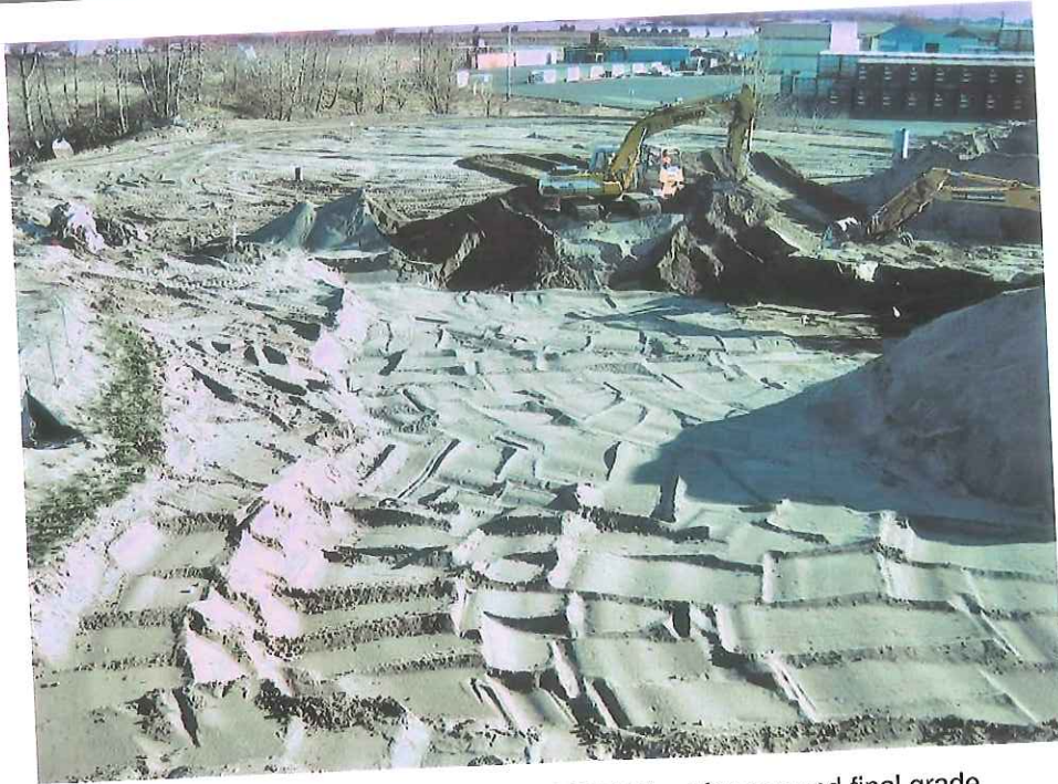
Excavation of unimpacted soil below HDPE liner for cap and final grade
