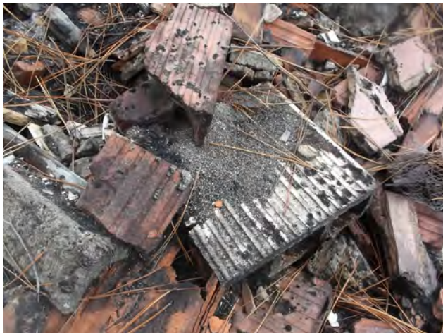
Close-up View of the RACM Vermiculite Insulation Present with the Large Building Materials Debris Pile.
