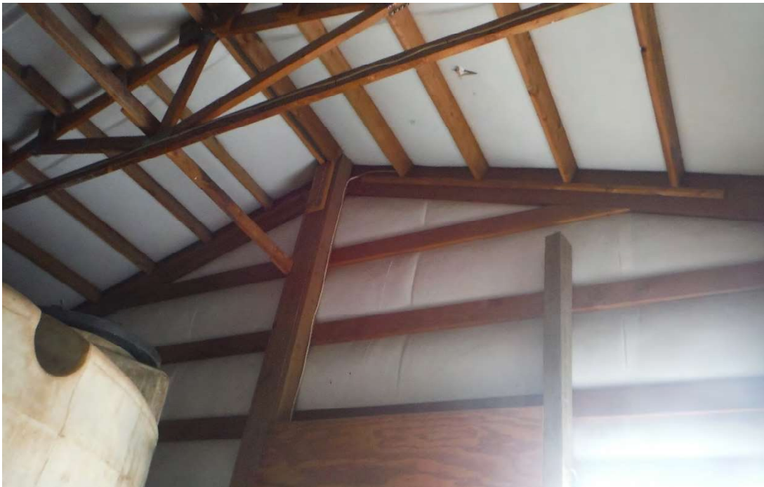
Photo 8 – Stormwater Treatment Building Interior
