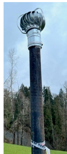
Figure 9. Wind Turbine Cap on Vent Pipe.
