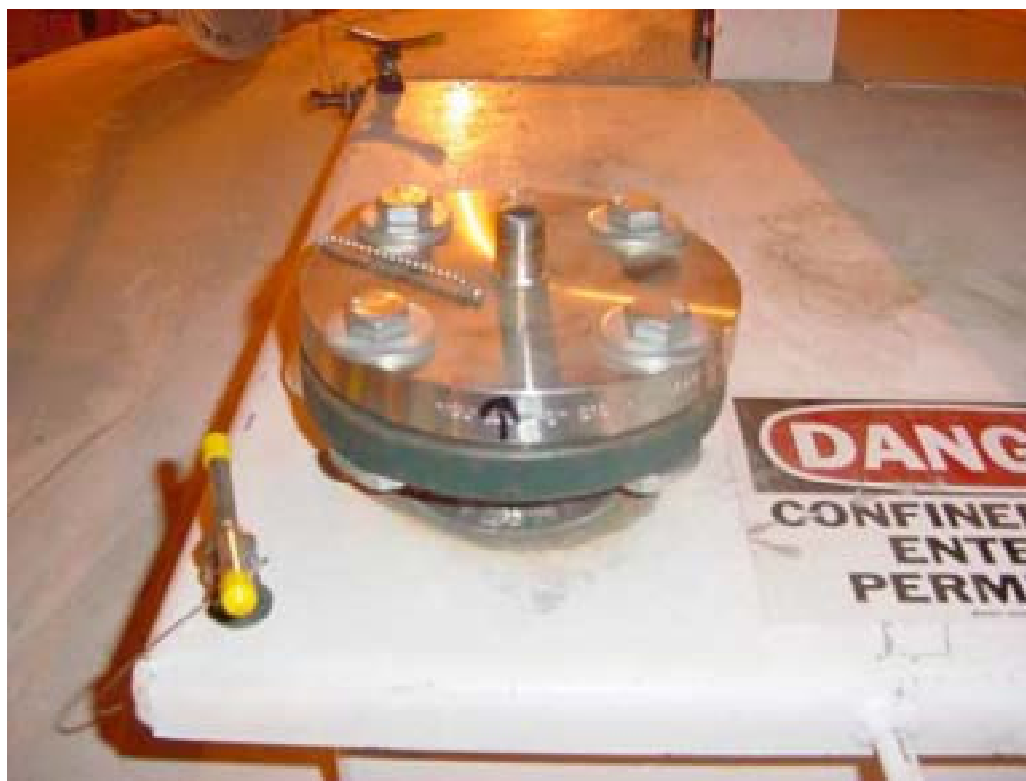
Figure 8. Tank 104 mechanical level sensor AIF-2. Test perimeter of flange.
