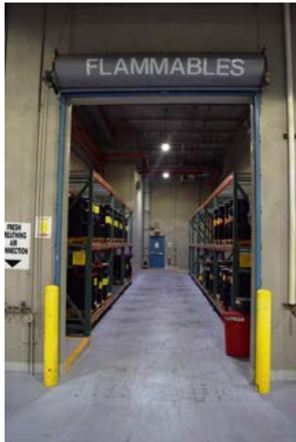
Photo 22: Flammables Storage (Rm 134), December 2017
