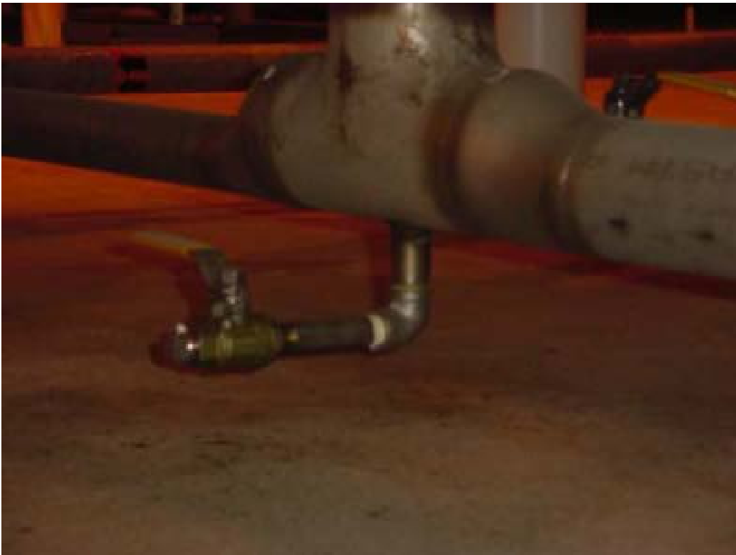
Figure 24. Tank 104 sample port valve AOV-2 and drain AOD-3. Test four threaded fittings and valve stem seal.
