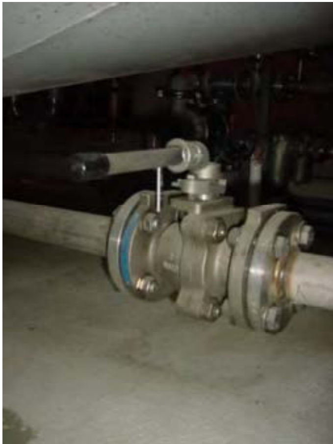
Figure 47. Tank 104 recirculation drain valve ARV-13.
