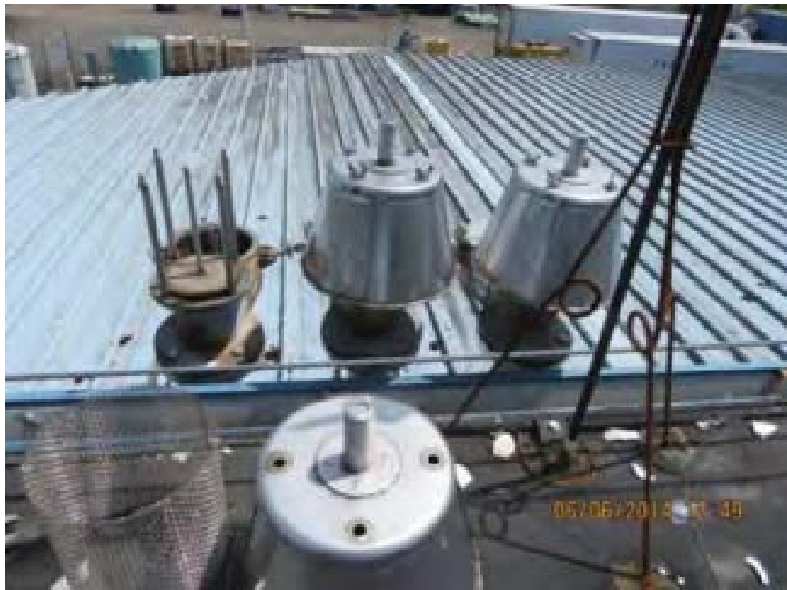
Figure 2. From left to right, vents AOF9 (105), COF8 (106) and AOF8 (104) located about 4 meters to the right of the Figure 1 vents on the BLDG 1051 roof. The pressure hood assembly is shown at the bottom right, the pressure screen is shown at the bottom left.
