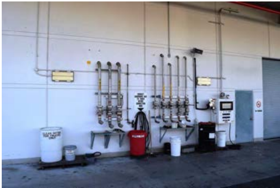
Photo 10: Truck Load/Unload Hose Station, December 2017
