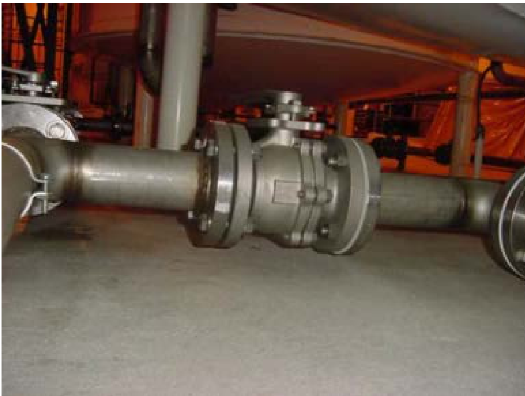
Figure 32. Tank 106 drain valve COV-2. Test perimeter of flanges at either end of valve, valve center flange, and valve stem seal.
