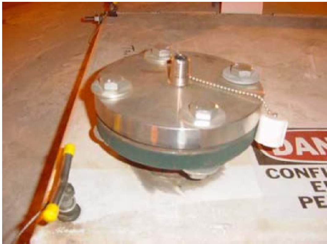
Figure 14. Tank 105 mechanical level sensor AIF-5. Test perimeter of flange.
