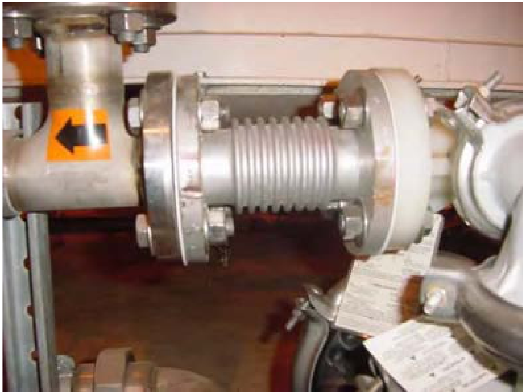
Figure 54. Recirculation fill pipe flex fitting ARF-5. Test perimeter of two flanges.
