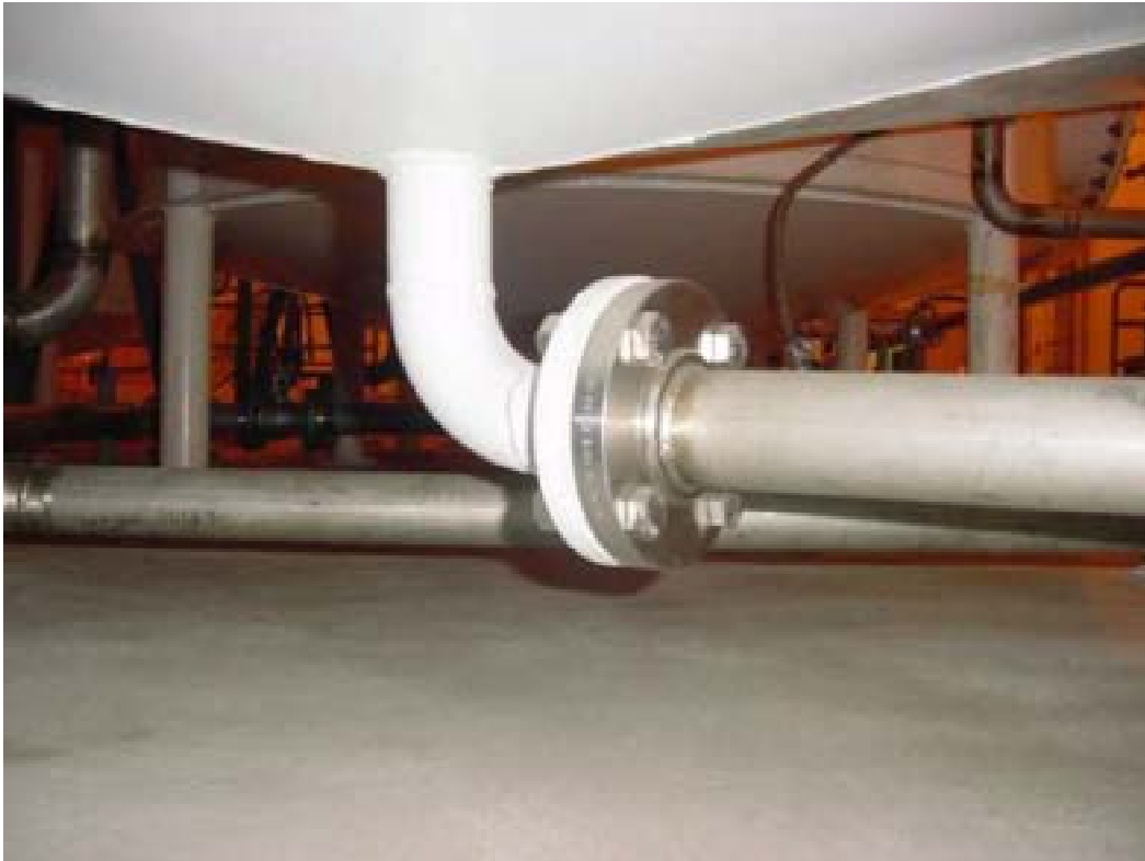
Figure 38. Tank 106 drain pipe flange (to be deleted in upgrade). Test perimeter of flange.
