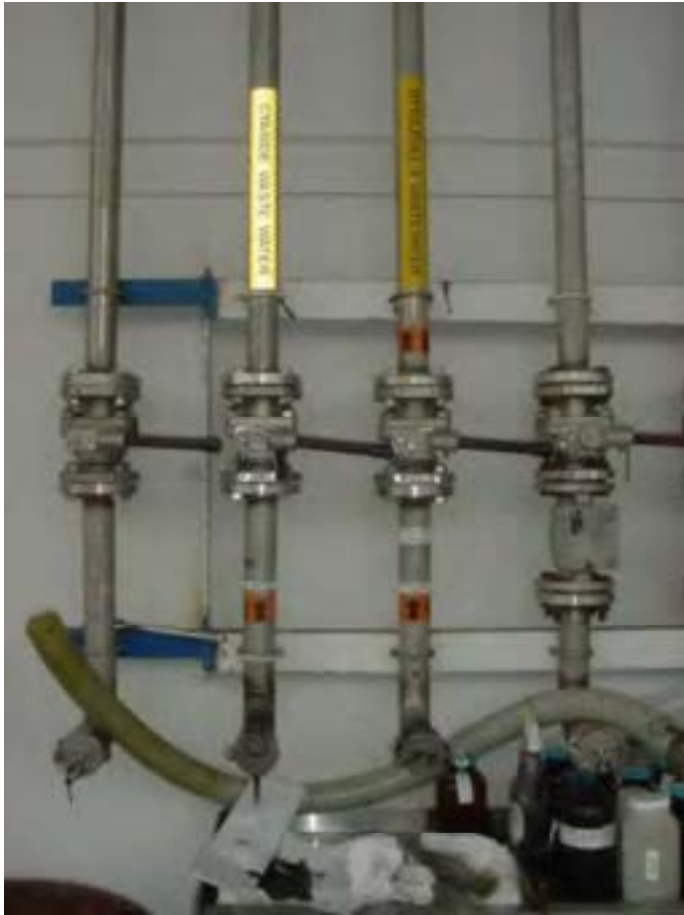
Figure 1. Outside waste tank fill pipe rack valves AIV-1, CIV-3 and end caps AID-1 and CID-2.
