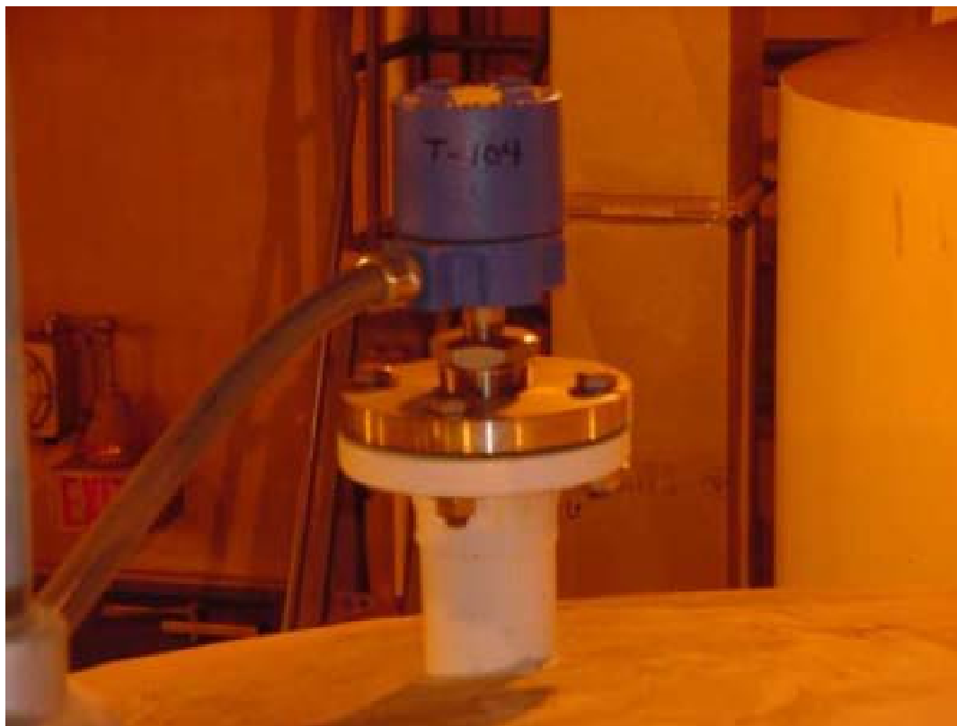
Figure 6. Tank 104 electronic level sensor AIF-3. Test perimeter of flange and two threaded fittings at base of sensor.
