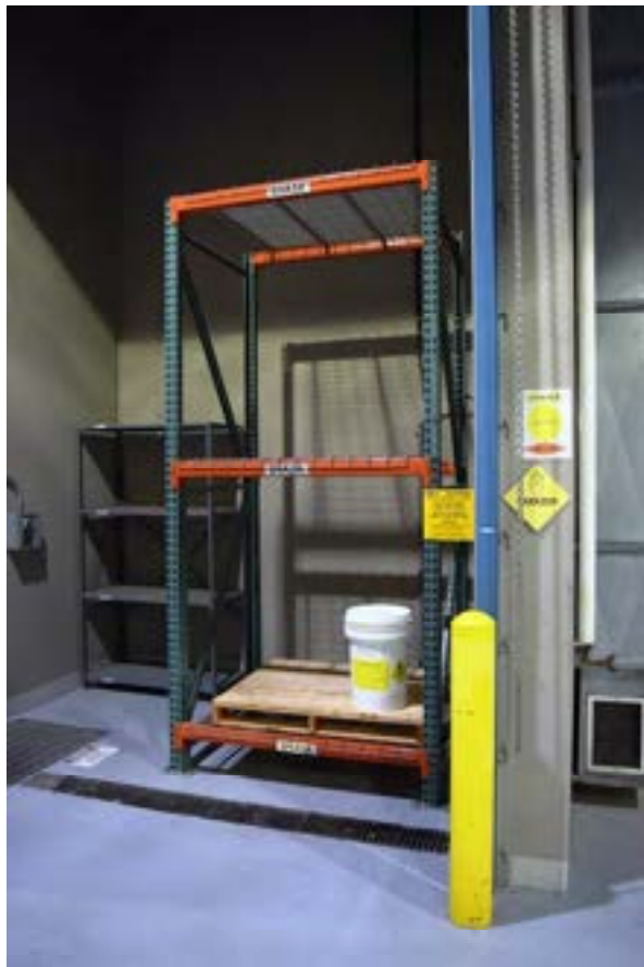
Photo 17: Oxidizer Storage (Rm 129), December 2017
