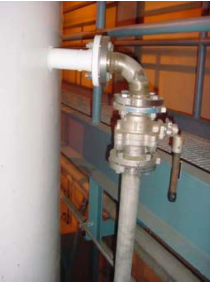
Figure 15. Tank 106 fill pipe valve CIV-5 and flange CIF-2.
