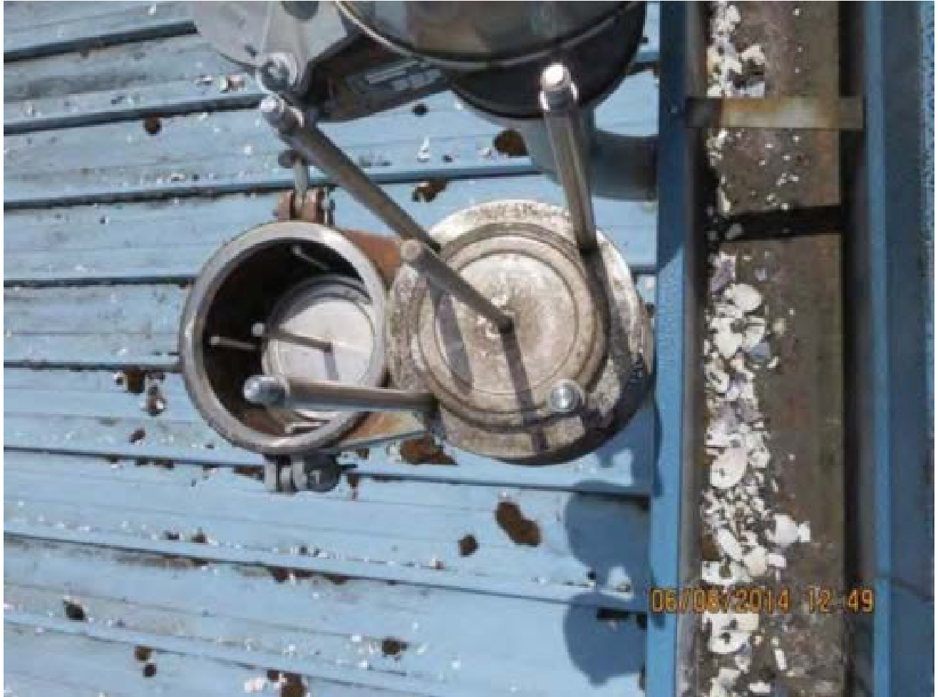
Figure 3. The pressure vent (right side in picture) cover and screen have been removed by detaching 4 wing nuts from the top. The suction vent (left side in picture) cover has been removed by releasing the hold-down wing nuts on both sides.
