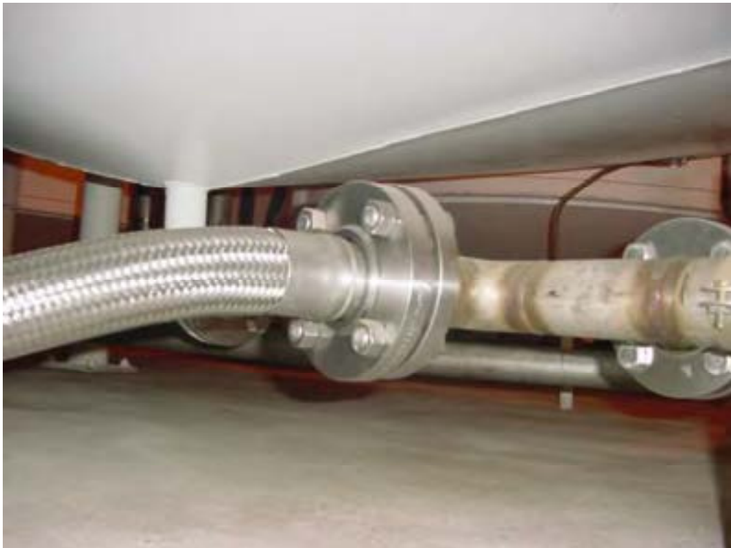
Figure 41. Backflush flex hose flange (to be deleted in upgrade). Test perimeter of flange.
