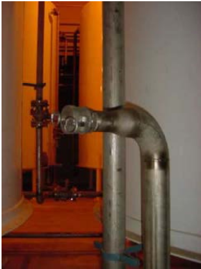
Figure 33. Tank 106 overflow cap COD-3.
