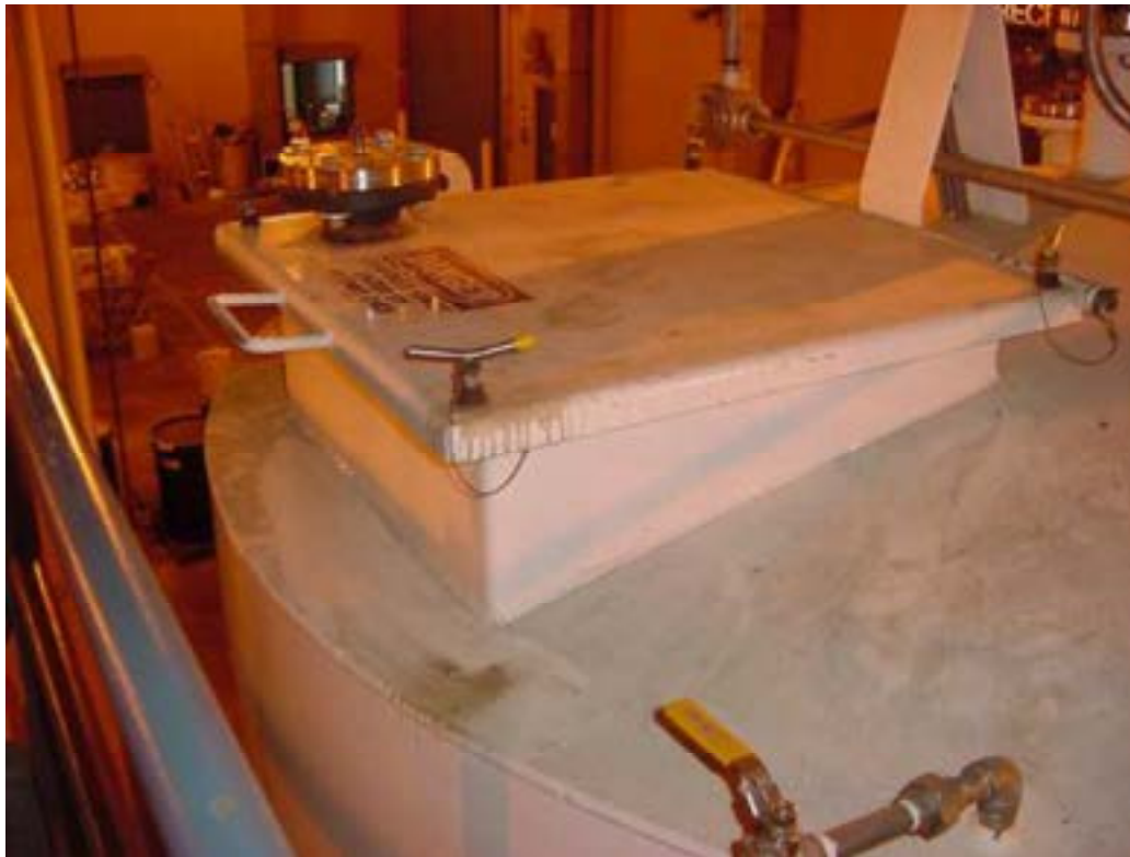
Figure 7. Tank 104 upper access hatch cover AIF-1. Test underside of entire hatch perimeter.
