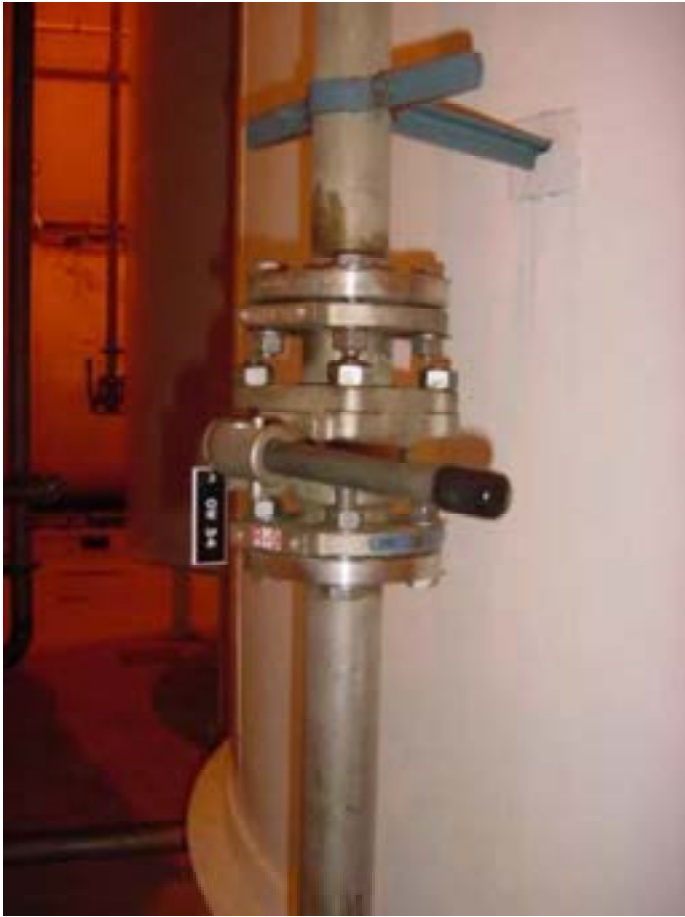
Figure 61. Tank 105 recirculation fill valve ARV-9.
