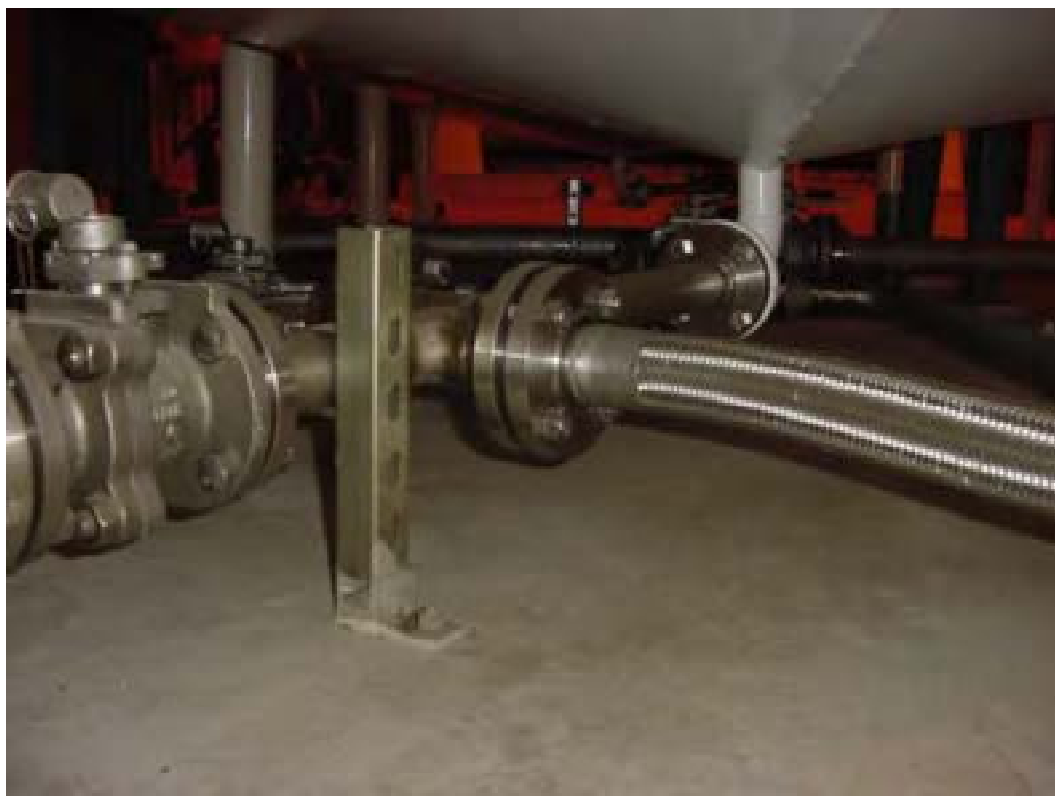
Figure 42. Recirculation drain flex hose flange (to be deleted in upgrade). Test perimeter of flange.
