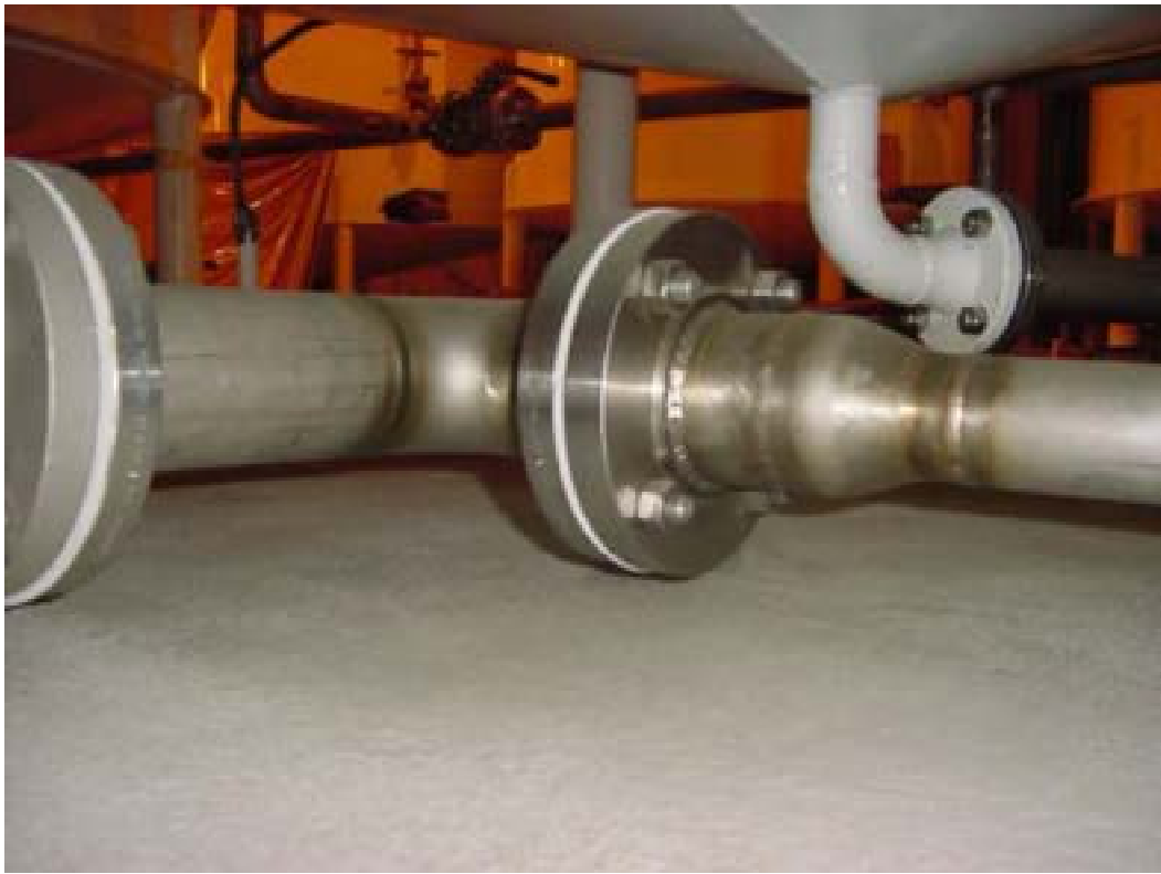
Figure 39. Backflush pipe flange (to be deleted in upgrade). Test perimeter of flange.
