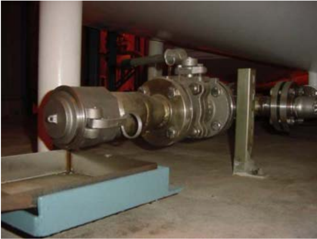
Figure 37. Backflush drain valve COV-1 and drain cap COD-1. Test perimeter of flanges at either end of valve, valve center flange, valve stem seal, and perimeter of end cap.
