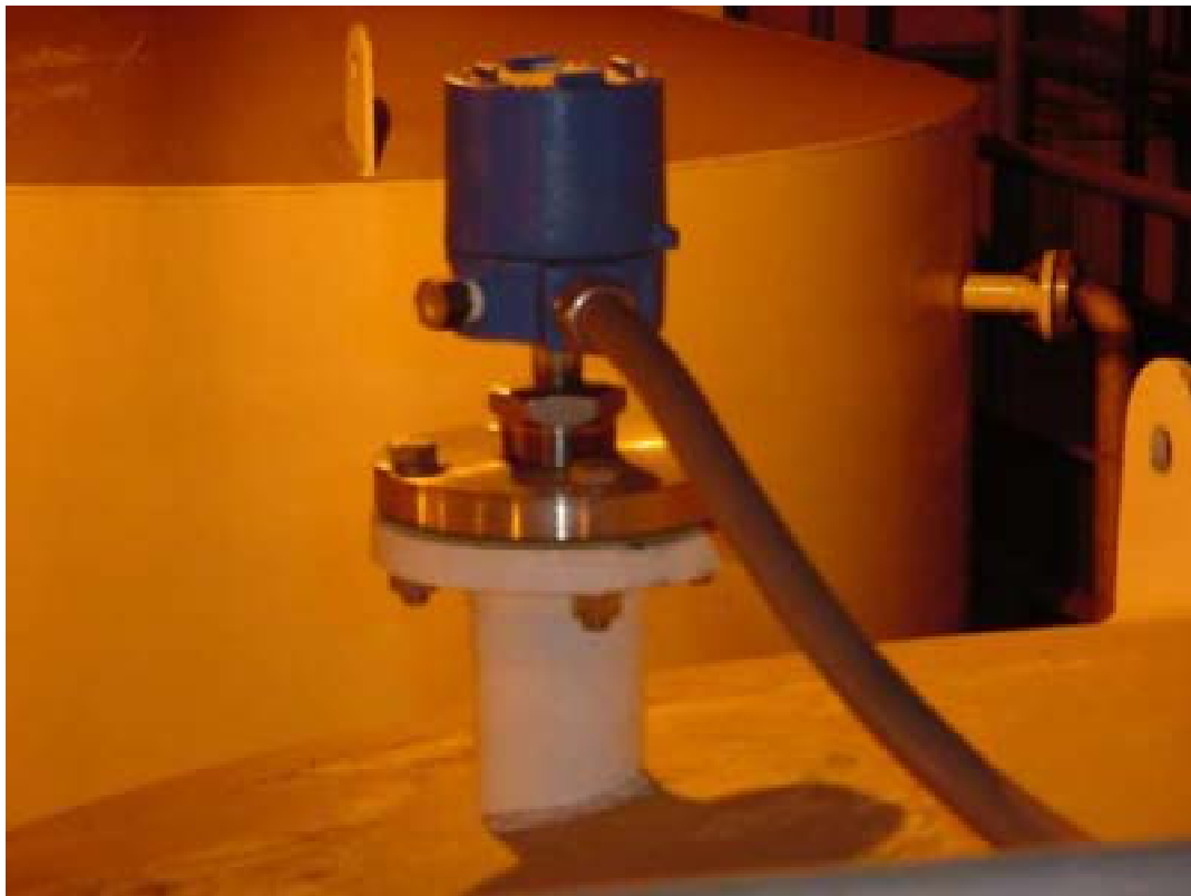
Figure 18. Tank 106 electronic level sensor CIF-8. Test perimeter of flange and two threaded fittings at base of sensor.
