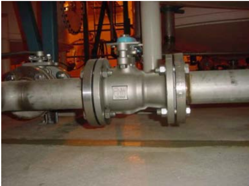
Figure 29. Tank 105 drain valve AOV-8. Test perimeter of flanges at either end of valve and valve stem seal.
