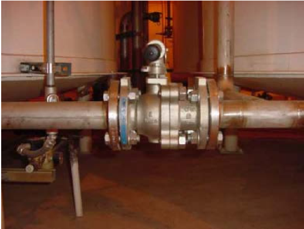
Figure 60. Recirculation fill valve ARV-8. Test perimeter of flanges at either end of valve, valve center flange, and valve stem seal.
