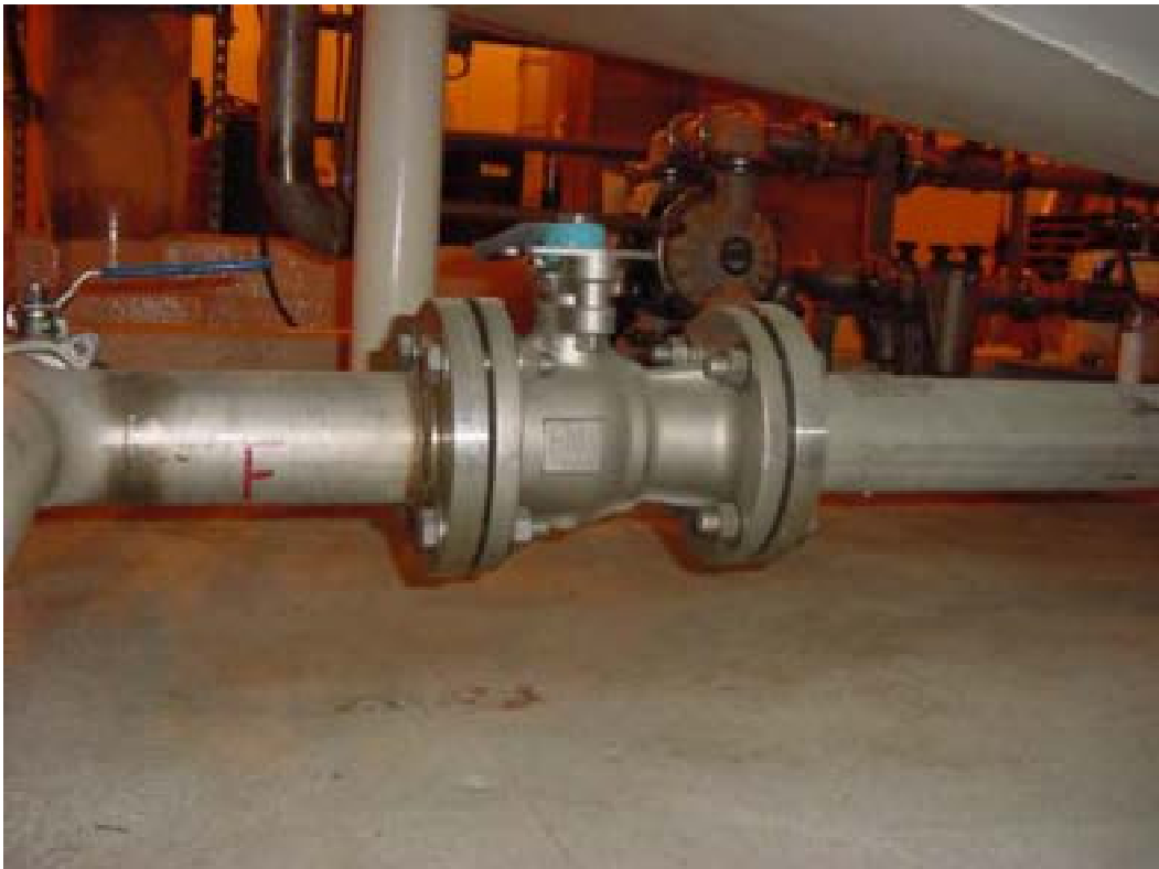
Figure 22. Tank 104 drain valve AOD-2. Test perimeter of flanges at either end of valve and valve stem seal.
