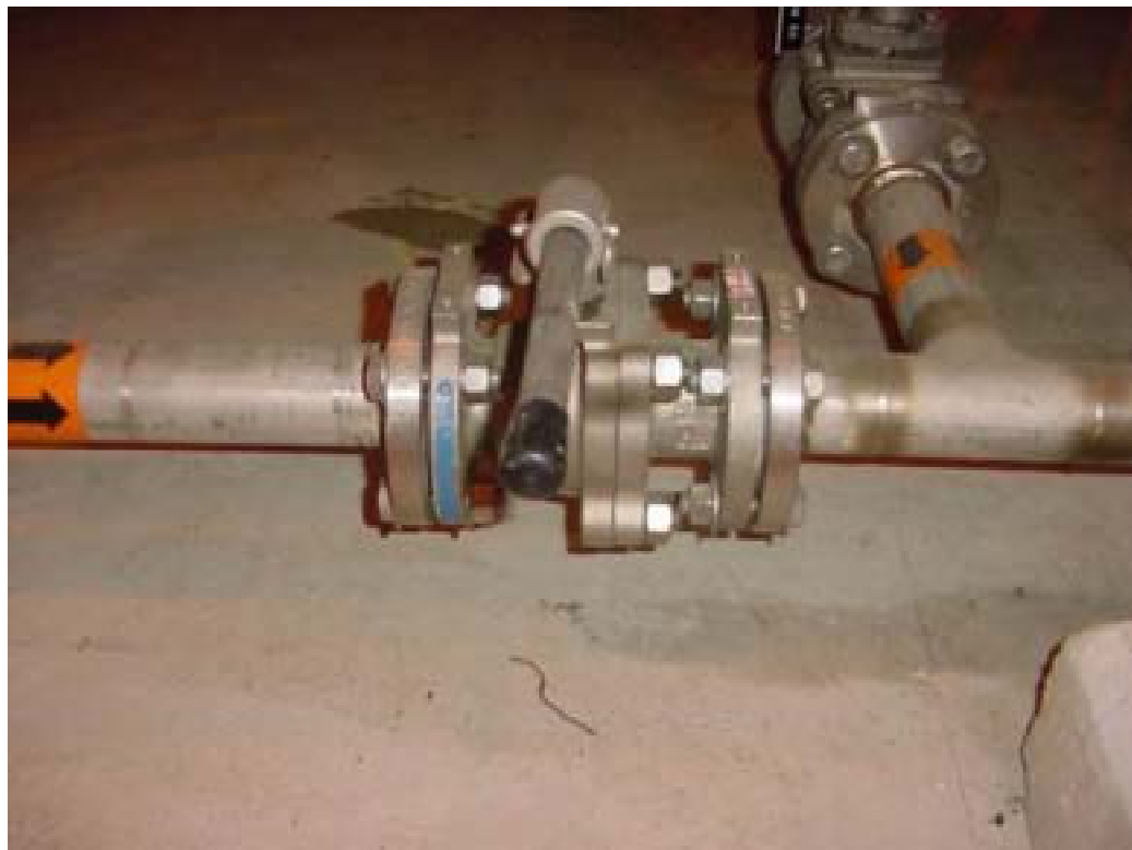
Figure 46. Recirculation drain valve ARV-12. Test perimeter of flanges at either end of valve, valve center flange, and valve stem seal.
