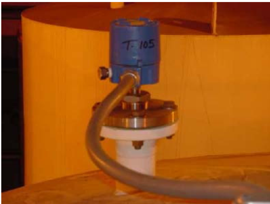
Figure 12. Tank 105 electronic level sensor AIF-6. Test perimeter of flange and two threaded fittings at base of sensor.
