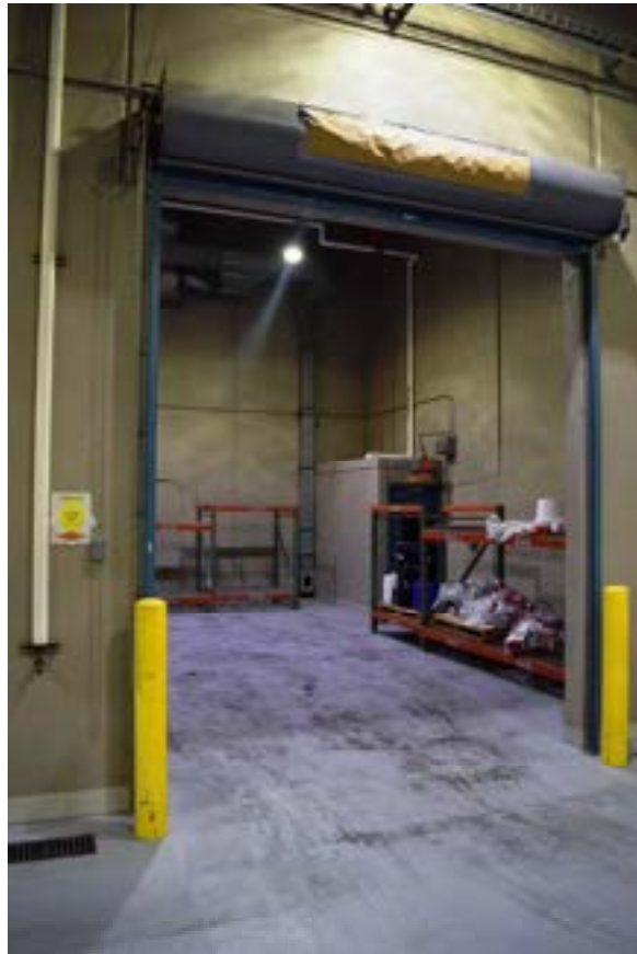
Photo 25: Used Oil Storage (Rm 139), December 2017
