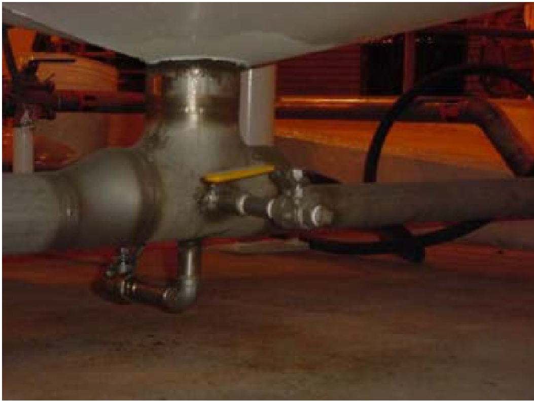
Figure 23. Tank 104 sample port valve AOV-3 and drain AOD-4. Test three threaded fittings and valve stem seal.
