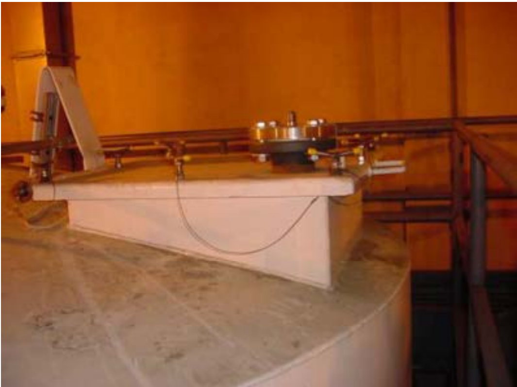
Figure 19. Tank 106 upper access hatch cover CIF-6. Test underside of entire hatch perimeter.
