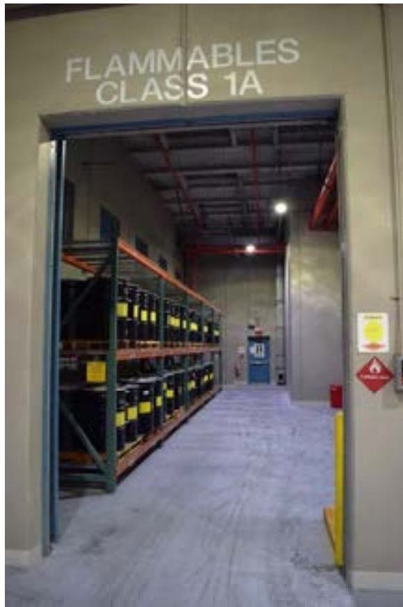
Photo 23: Flammables Class 1A (Rm 136), December 2017
