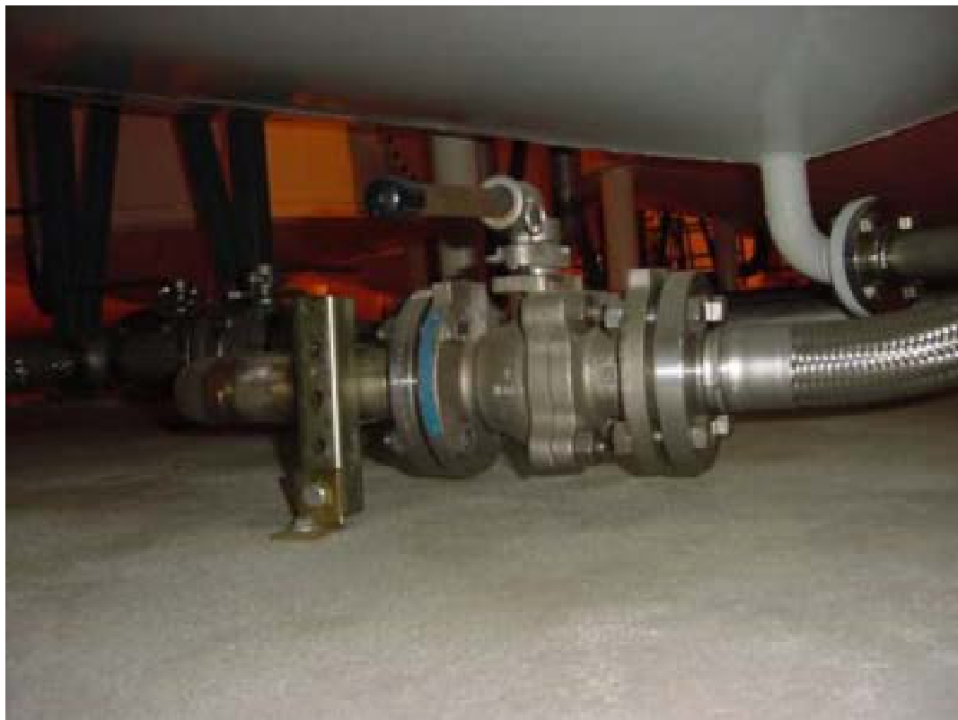
Figure 40. Backflush valve (to be deleted in upgrade). Test perimeter of flanges at either end of valve, valve center flange, and valve stem seal.
