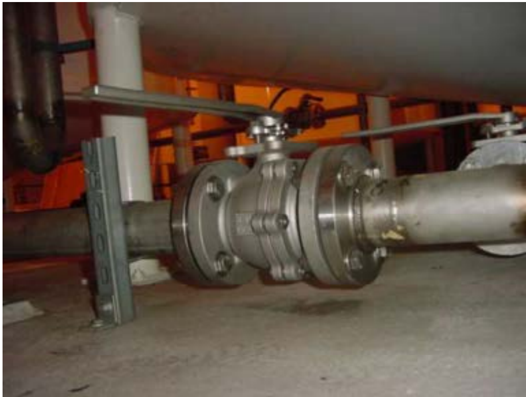
Figure 31. Main drain pipe valve AOV-9. Test perimeter of flanges at either end of valve, valve center flange, and valve stem seal.
