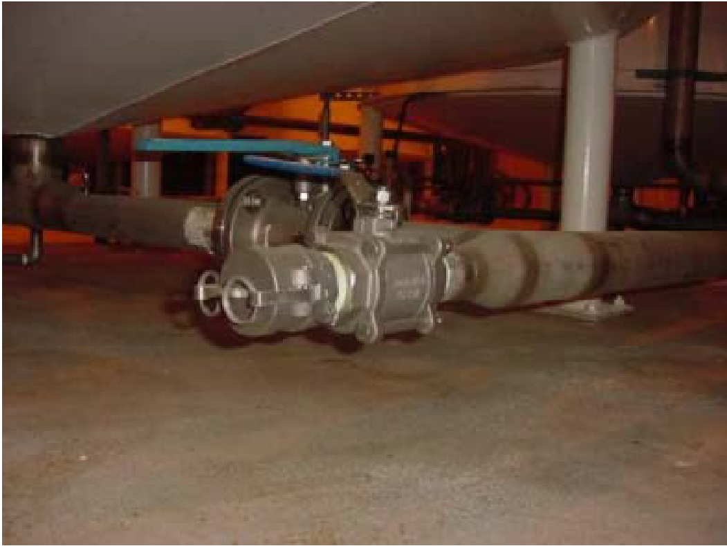
Figure 21. Main drain pipe valve AOV-1 and end cap AOD-1. Test perimeter of cap, perimeter of flanges at either end of valve, valve stem seal, and perimeter of end cap.
