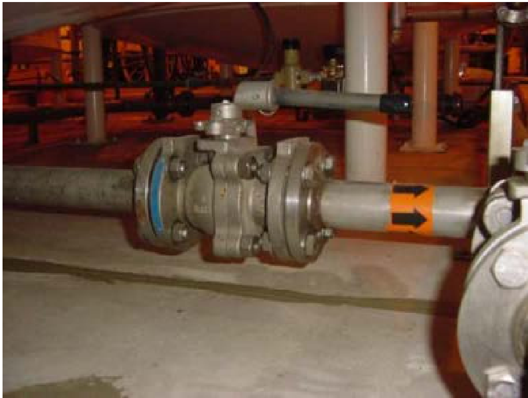
Figure 45. Tank 105 recirculation drain valve ARV-11. Test perimeter of flanges at either end of valve, valve center flange, and valve stem seal.
