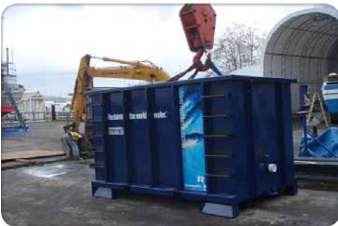
Installation of an Aquip 50 system
