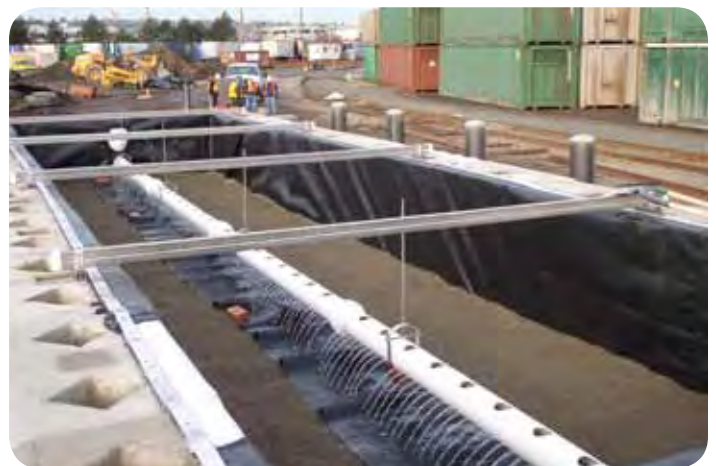
View of Aquip inlet distributor
