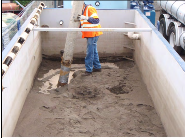
Figure 9. Vactor service removing the top layers of sand during a Seasonal Maintenance
