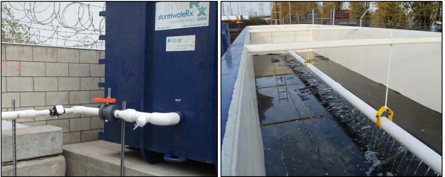
Figure 4. Inlet piping with flow meter (right); Uniform flow out the inlet distributor (left)
