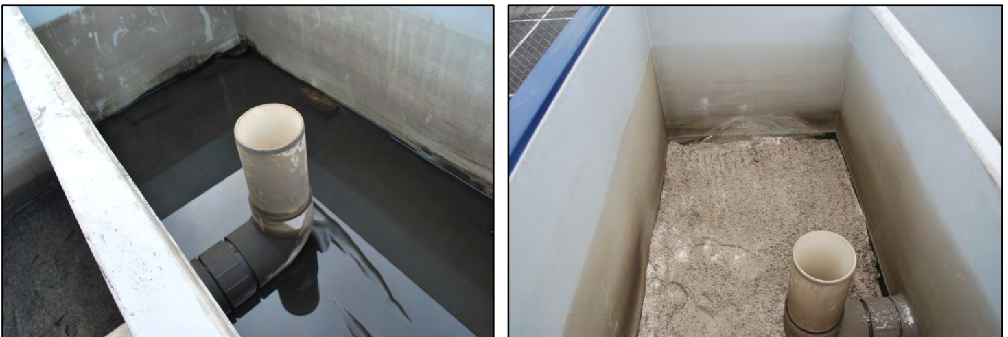
Figure 11. Pretreatment chamber (with pretreatment media) in need of maintenance (left); pretreatment media after maintenance (right)
