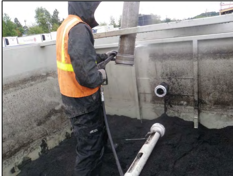
Figure 10. Pressure wash the sidewalls of Aquip before removing filter media during a full maintenance.
