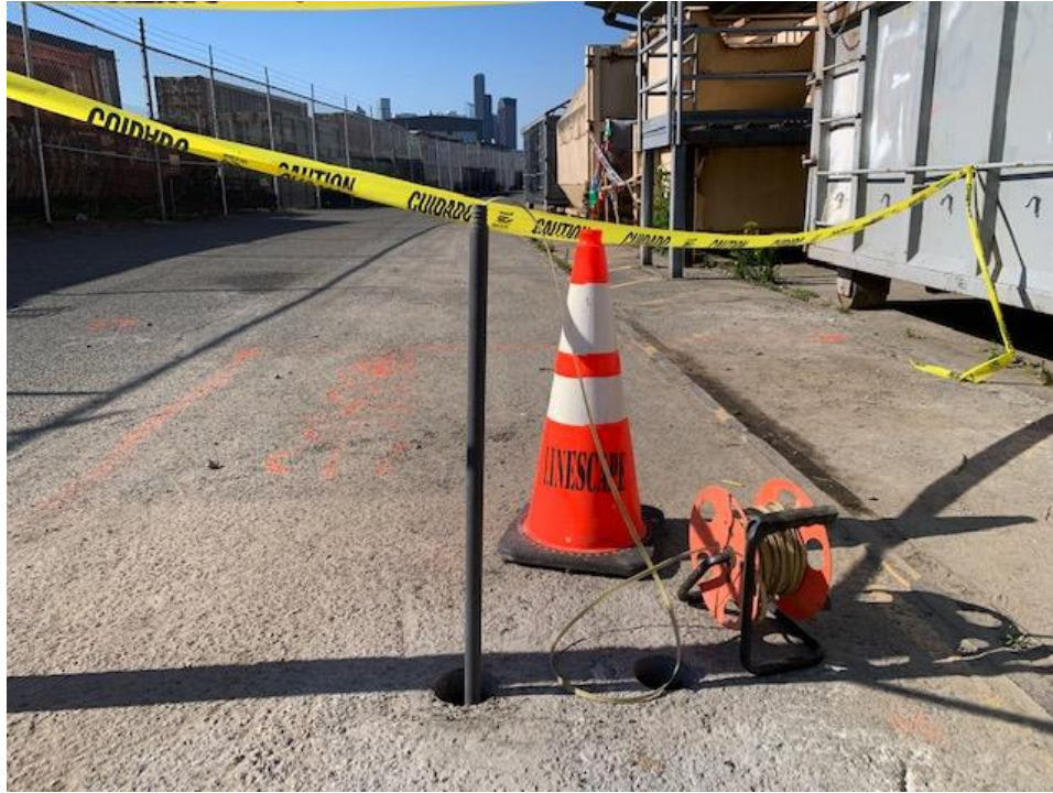
Photo 5: Groundwater infiltrating into borehole B6
