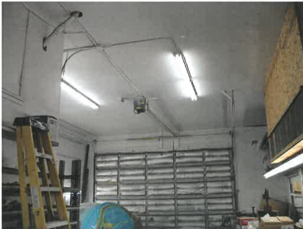
18. Fluorescent lights in the paint/body work room
