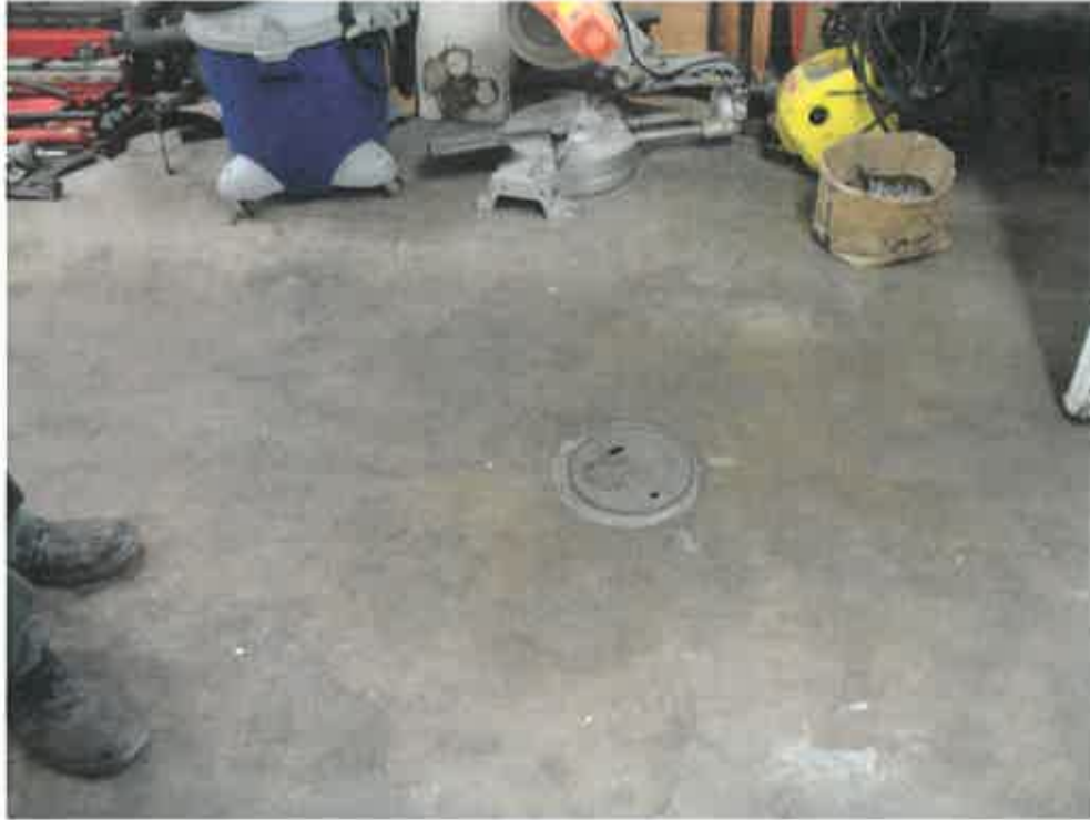
17. The waste oil UST port in the floor at the west end of the paint/body work room
