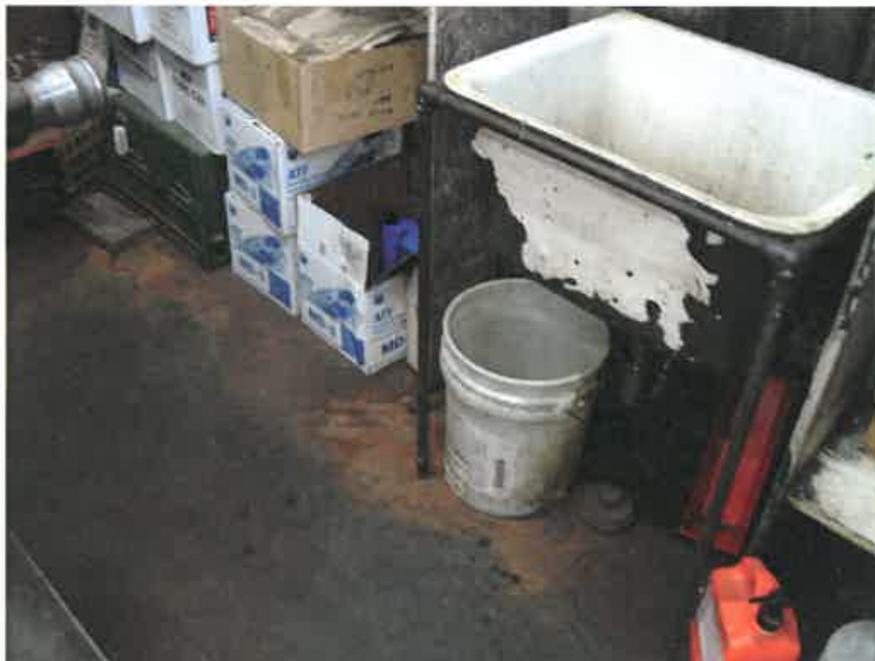
14. A sink and drain in a room adjacent to the service bays
