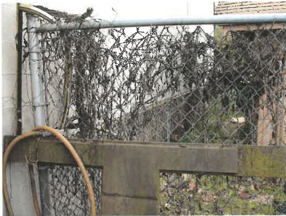
19. Looking east across the north side of the paint/body work room addition
