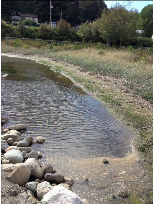
Photograph 15 – Tidal inundation within wetland mitigation area
