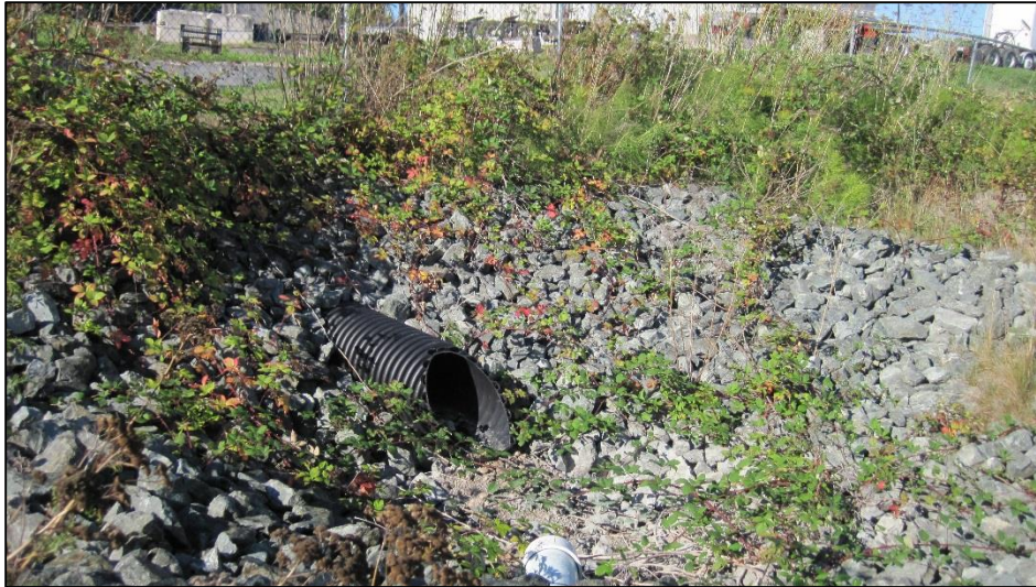
Photograph 18 – Himalayan blackberry and other non-natives present at entrance of stormwater swale
