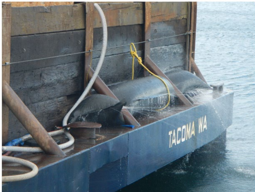
Photo #18: Example of dewatering by filtering excess water through a “geotube” on the materials barge.
