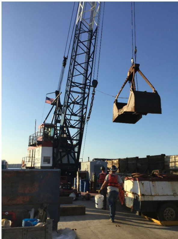
Photo #6: Clamshell bucket predominately utilized during both dredging and backfill, approximate volume of 4 cubic yards
