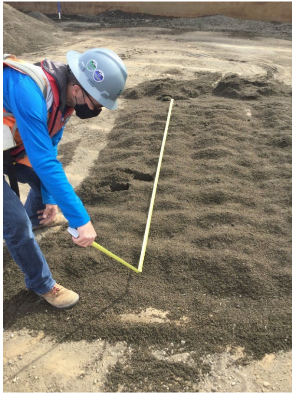
Photo #13: Measurements taken during a practice dry-run on the barge of the 2-inch thin layer cap table.
