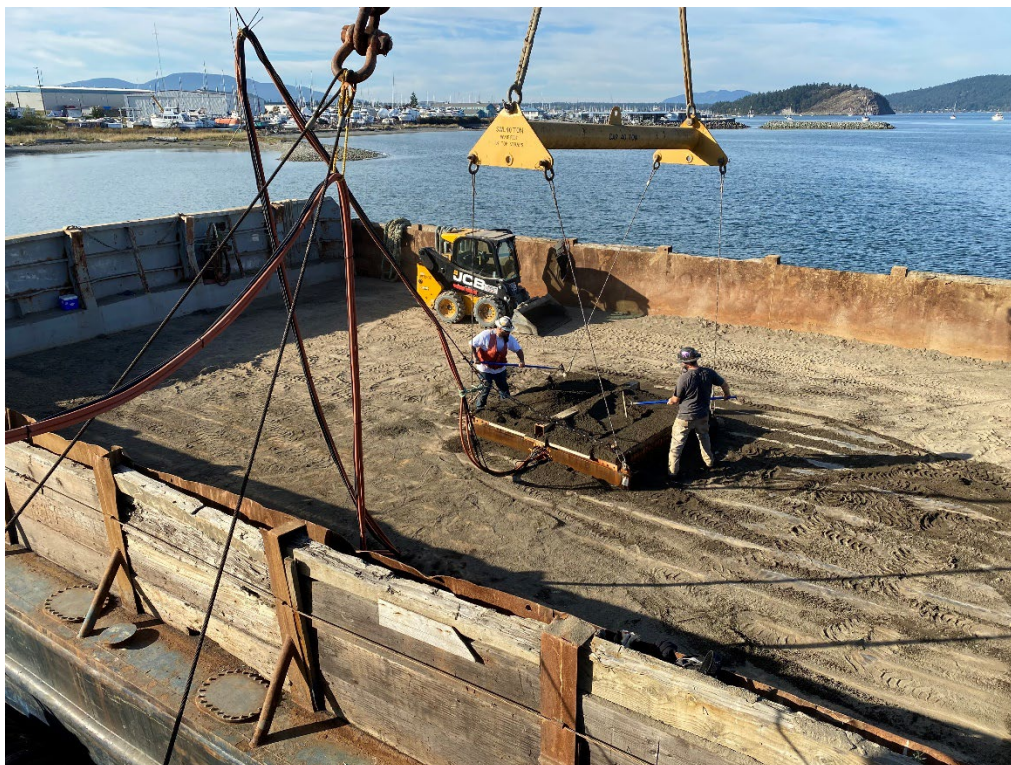
Photo #12: The steel table was filled using a small skid steer loader and then two deck hands used rakes to remove excess and level out the backfill to be placed
