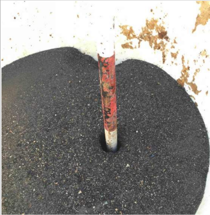
Measurement of RB #14 (5.5", fail)
