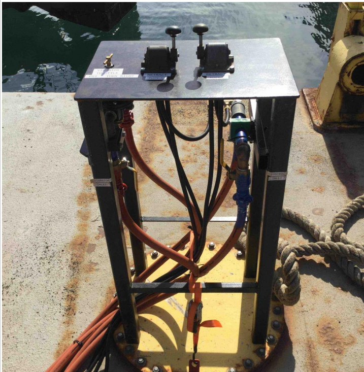
Controls for 2" table to be tested today, implemented tomorrow 9/16.
