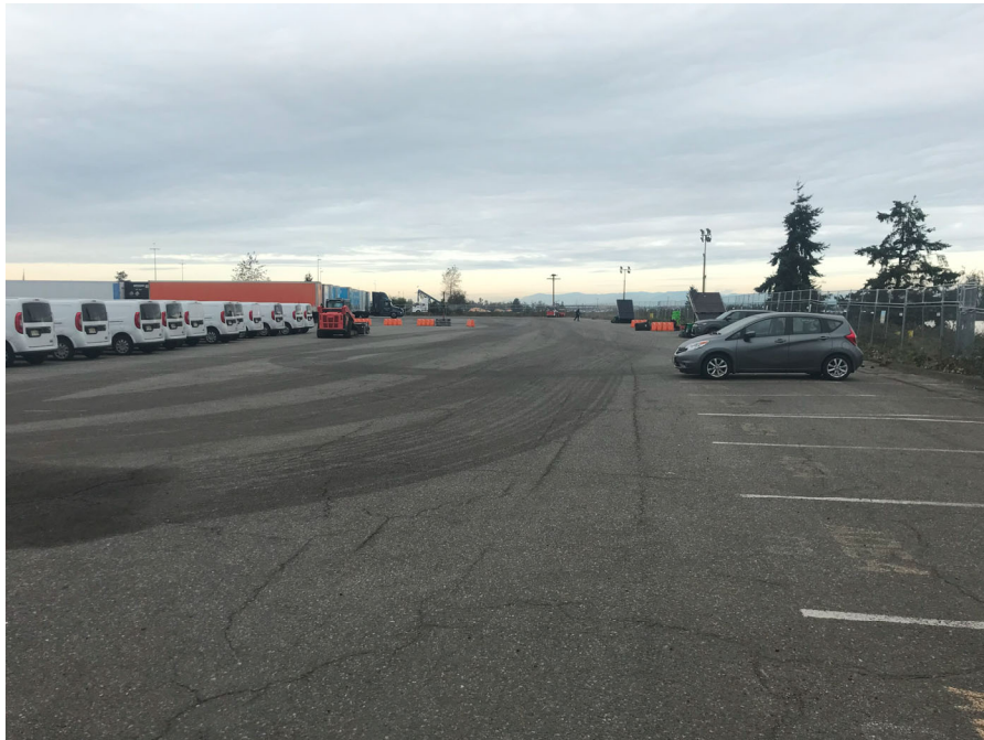
Photograph 2 – Looking north-northeast at the southeastern portion of the asphalt cap with thin cracks on surface.
