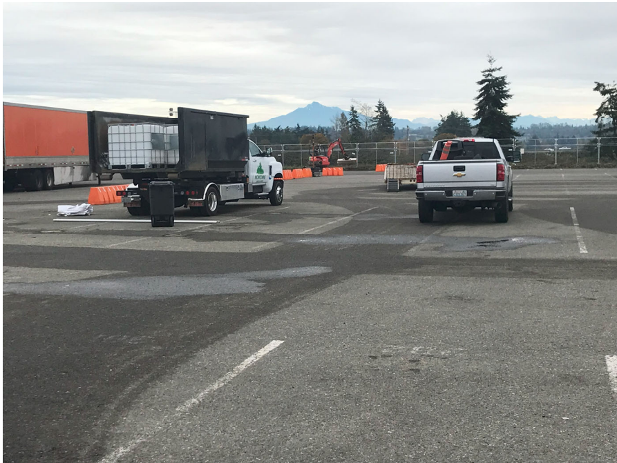
Photograph 6 – Looking east at center portion of the asphalt cap. Minor ponding observed on the asphalt surface after a rainfall event.
