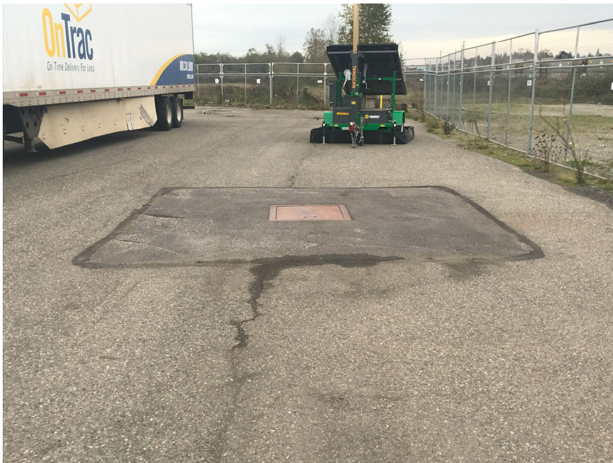
Photograph 4 – Looking south at central western portion of the asphalt cap with observed minor cracking on the surface.
