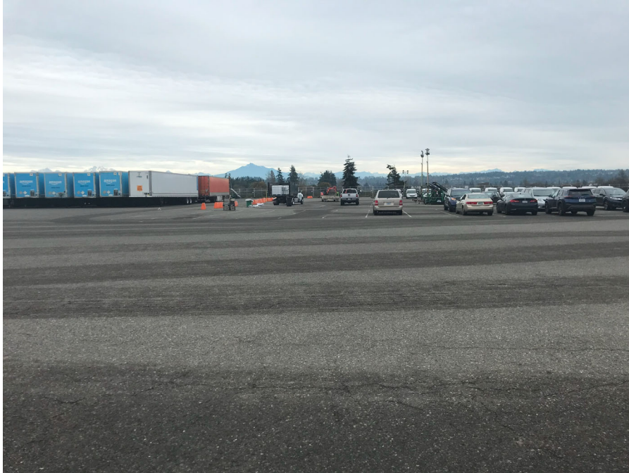
Photograph 5 – Looking east at central western portion of the asphalt cap. Minor ponding observed on the asphalt surface after a rainfall event.
