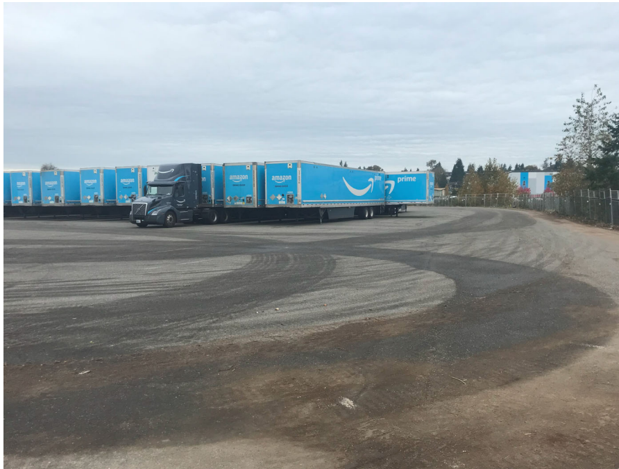
Photograph 1 – Looking west at the northern portion of the asphalt cap. Multiple cracks are observed to be repaired with a crack joint sealant.
